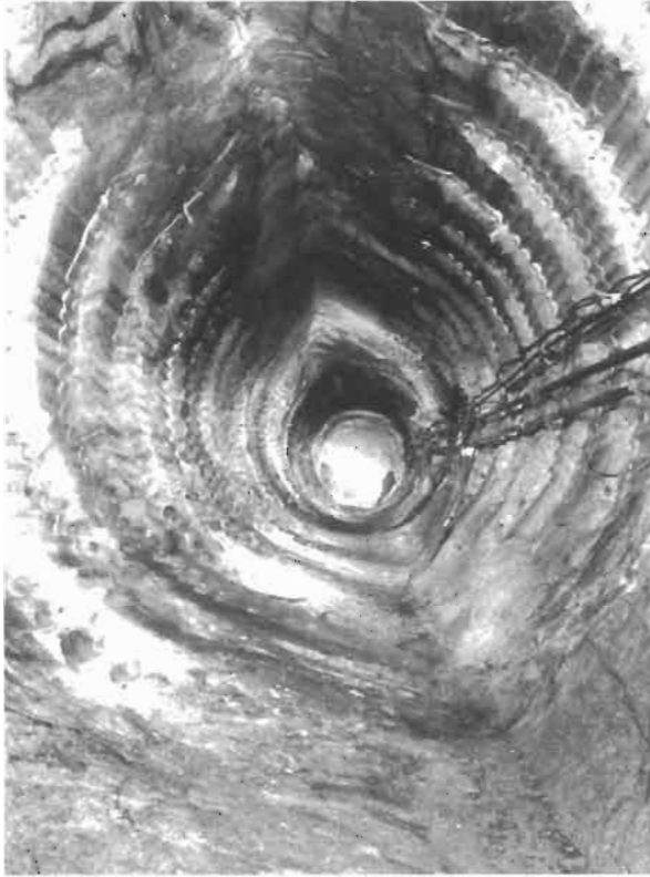
Figure 2.7 Tunnel deformation caused by high rock stresses at the Underground Research Laboratory, Manitoba, Canada.
