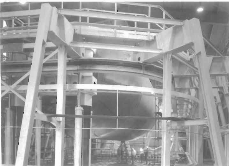
Figure 4.20 RP 150,000 gal tank
