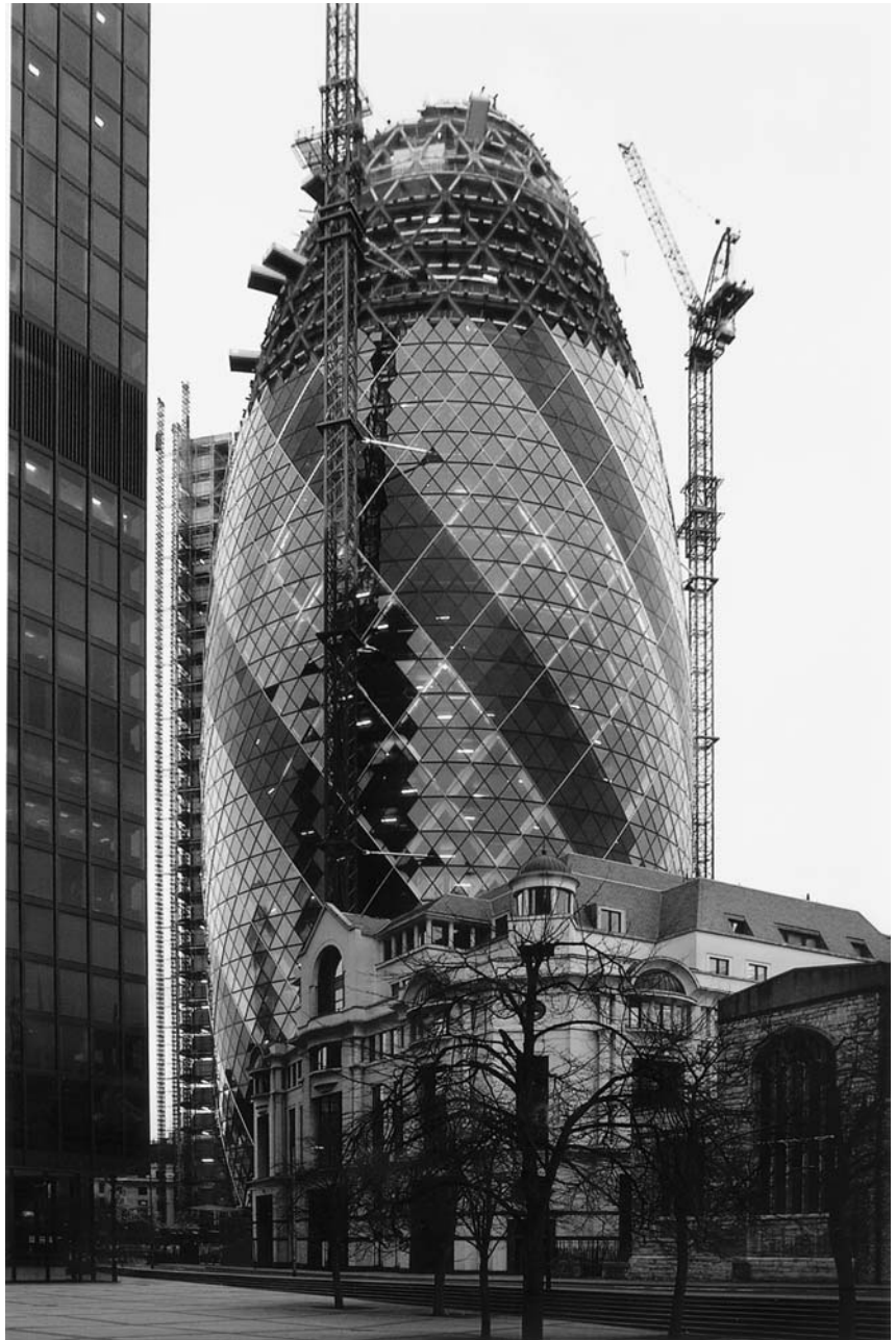
▲ A11.3 Swiss Re, London, England. Installation of cladding. Foster and Partners, 1997–2004. Photo: Norman Childs.
