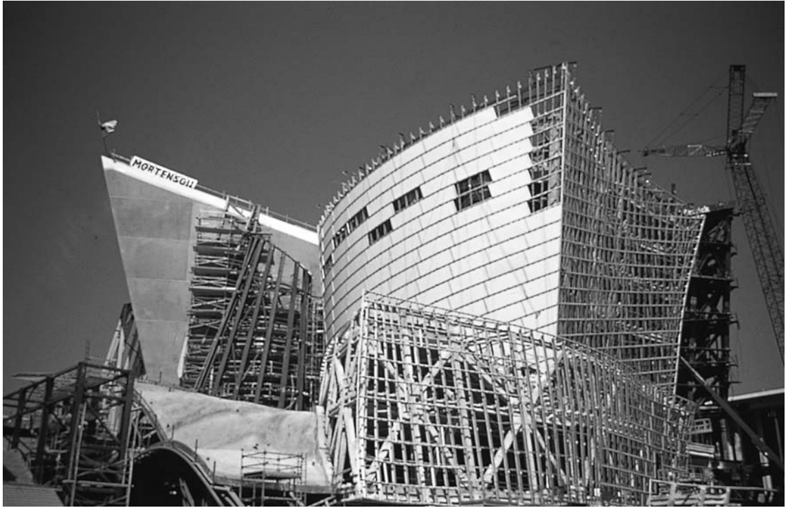
▲ 4.65 Walt Disney Concert Hall. View under construction showing primary and secondary steel structures beneath stainless steel skin. Photo: Lara Swimmer/Esto.
