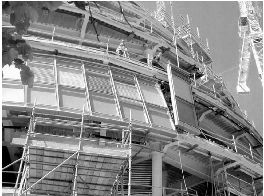
► AII.2 GLA Headquarters, London. Installation of cladding. Norman Foster, 1998–2002. Photo: Nigel Young/Foster and Partners.
