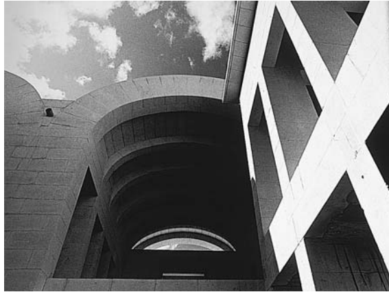
► 6.20 Victor Mangion's House. View of house under construction showing stone vaulting system. Photo: David Pisani.
