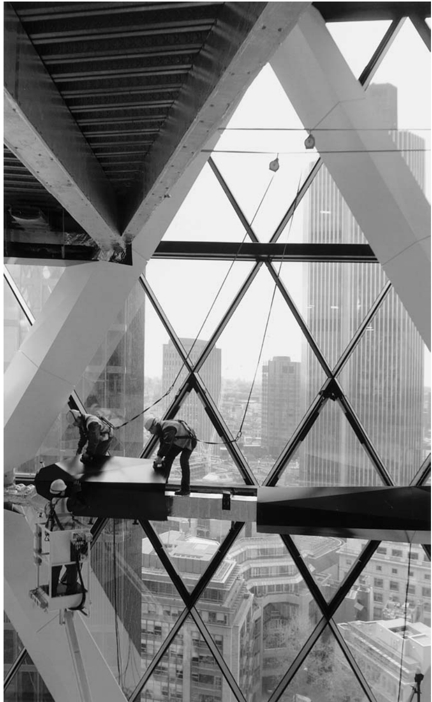
► AII.4 Swiss Re, London, England. Diagonal kink in metal cladding of structure necessitated by twisting geometry is clearly visible from interior. Foster and Partners, 1997–2004. Photo: Norman Childs.
