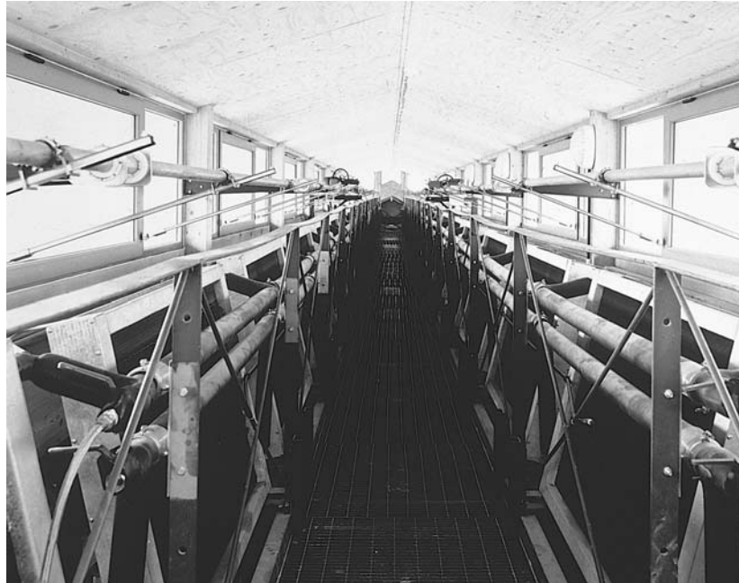
► 6.12 Malta Stock Exchange. Evaporative cooling system. View under ridge showing chilled water cooling coils and hydraulically operated vents. Photo: David Pisani.
