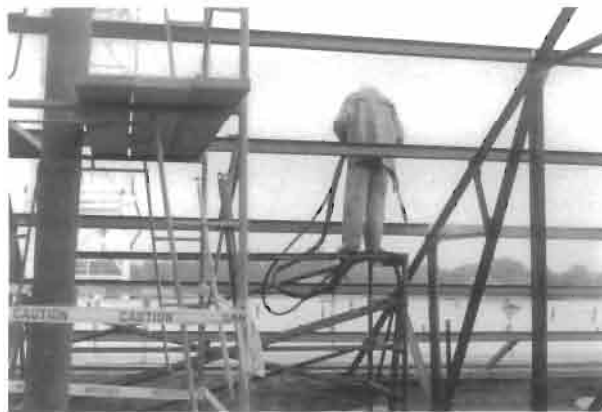
Figure 7.26 Use of ice jetting during a steel bridge rehabilitation project (photographs: Universal Ice Blast, Bellevue, WA).
