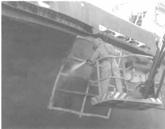
Figure 7.20 Ultra-high pressure abrasive blasting (UHPAB) systems in operation (photographs: Mühlhan Surface Protection Intl. GmbH, Hamburg).
