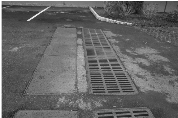
FIGURE 9.29 Underground sand filter, clogged by silt and totally ineffective. (Photo by the author.)
