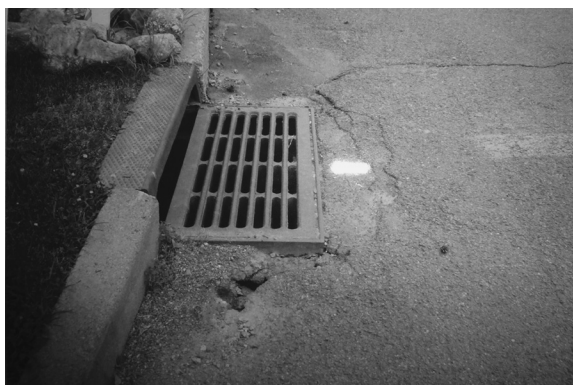
FIGURE 9.17 Pavement damage due to joint leak. (Photo by the author.)
