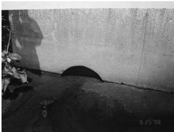
FIGURE 9.28 Drainage pipe, over two-thirds filled with silt. (Photo by the author.)
