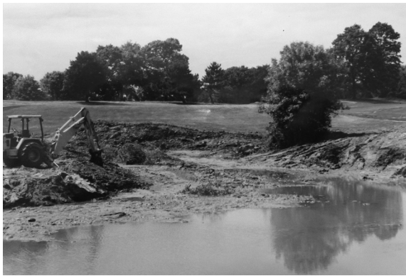
FIGURE 9.2 Loose, highly erodible soil at a construction site; a potential source of water pollution.
