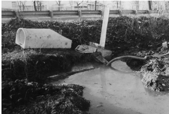
FIGURE 9.10 Sump pump dewatering pipe installation in a high water table site. (Photo by the author.)
