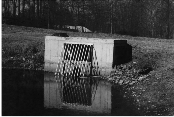
FIGURE 9.26 Trash rack with parallel bars on an outlet structure. (Designed by the author.)
