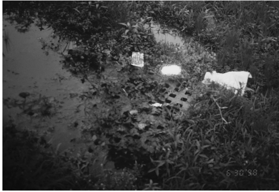
FIGURE 9.27 Inlet grate, clogged by leaves. (Photo by the author.)
