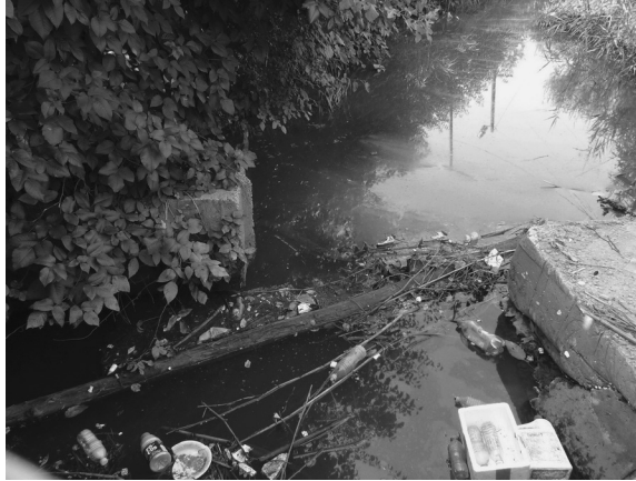
FIGURE 1.3 Bottles and floatables trapped behind culverts. (Photo by the author.)
