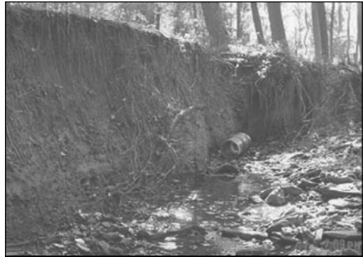
High volumes of stormwater discharge have badly damaged this stream near Philadelphia, which is suffering from Urban Stream Syndrome. Photo by Chris Crockett, City of Philadelphia Water Department.
