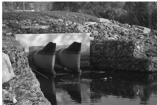
FIGURE 4.49 Gabion walls at drainage outfall at a tidal channel. (Photo by the author.)
