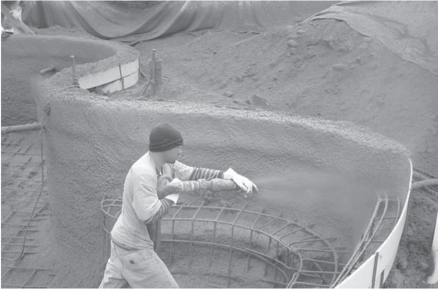
FIGURE 7.46 Constructing a swimming pool using shotcrete. (Courtesy of the American Shotcrete Association)
