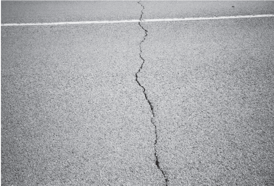
FIGURE 9.12 Thermal cracking resulting from the use of too-stiff asphalt in a cold climate area. (Courtesy of FHWA)
