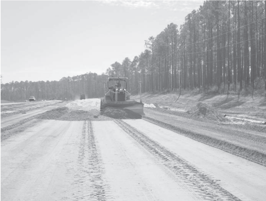
FIGURE 5.2 Constructing aggregate base before placing the hot-mix asphalt or portland cement concrete layer of a paved road.
