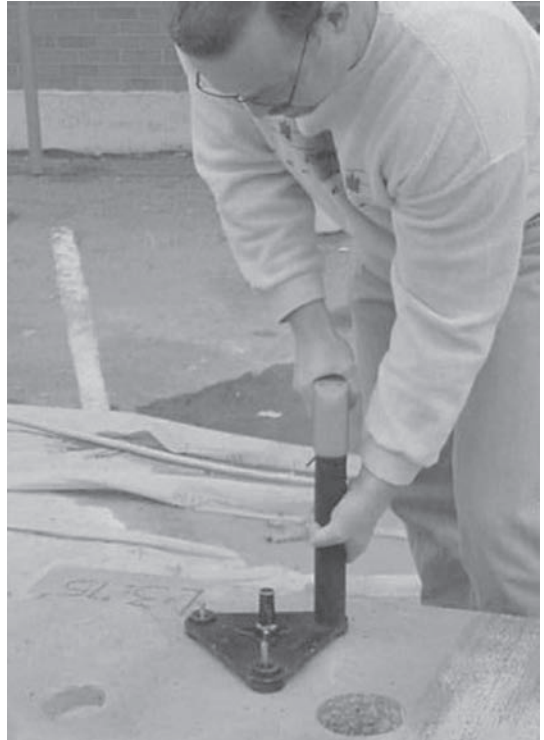
FIGURE A.48 Firing and driving Windsor probe into concrete using triangular positioning device.
