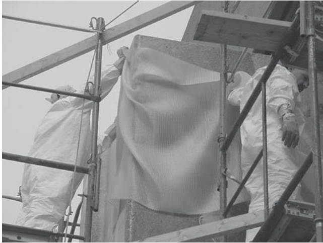
FIGURE 11.10 Wrapping an old structure with glass fiber-reinforced polymer composite. (Courtesy of R.J. Watson)
