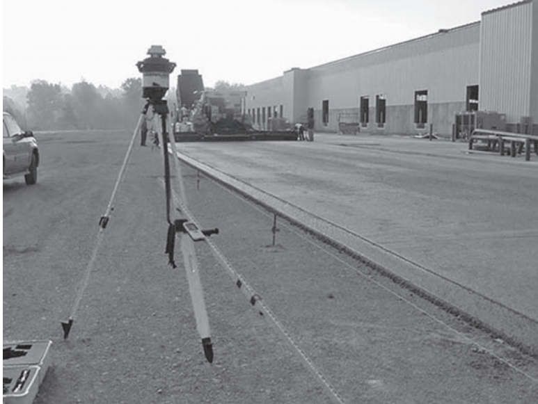
FIGURE 7.52 Placing roller compacted concrete with a vibratory screed. (Courtesy of A.G. Peltz Group, LLC)
