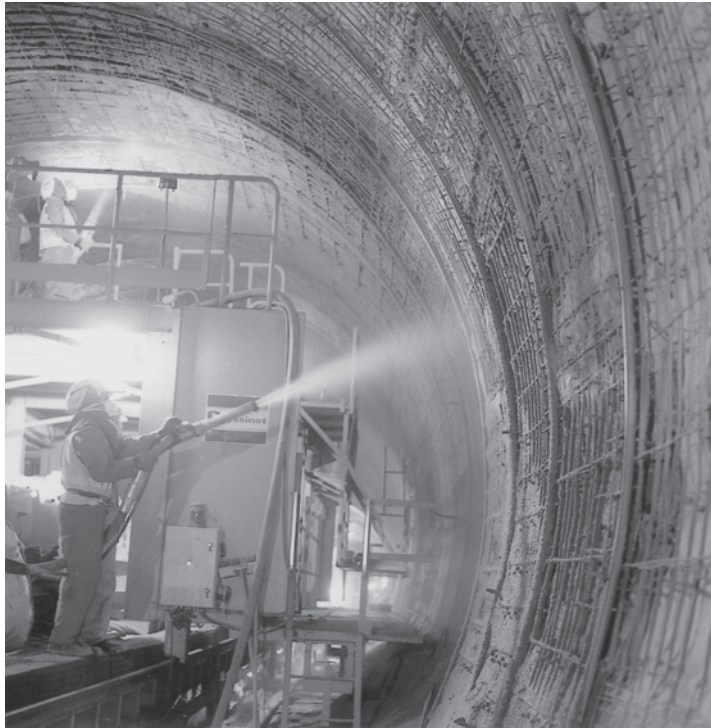
FIGURE 7.47 Shotcrete used in lining a tunnel. (Courtesy of the American Shotcrete Association)
