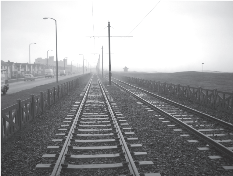
Figure 4.38 Example of segregated open light rail tracks in Blackpool (Photo: L. Lesley)
