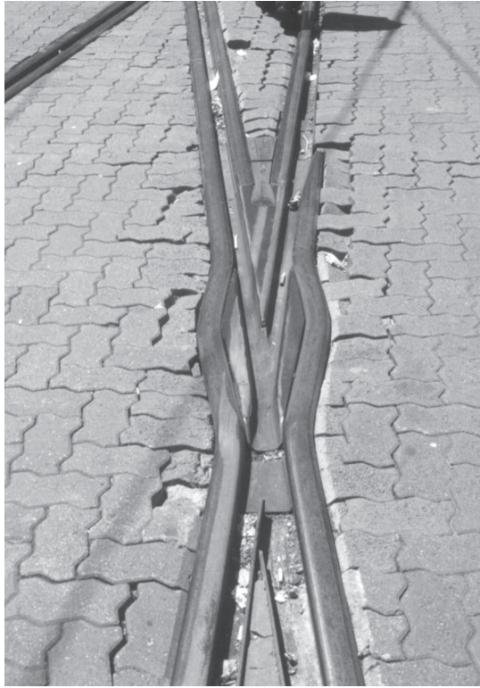
Figure 4.48 Crossing failure in Sacramento (Photo: L. Lesley)
