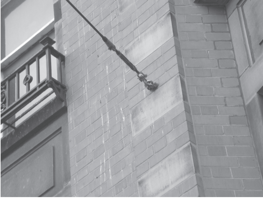
Figure 4.25 Span wire wall fixing in Sheffield, 2008 (Photo: L. Lesley)
