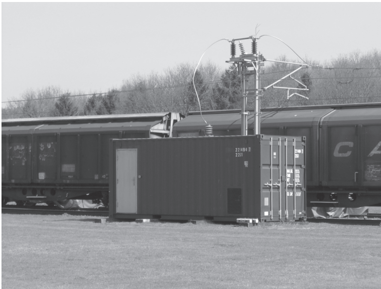
Figure 4.31 Portable substation in container (Photo: L. Lesley)
