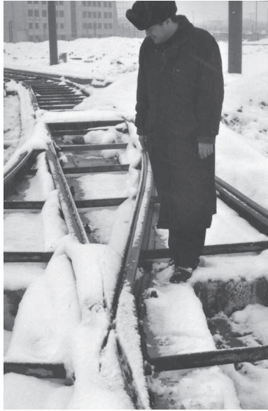
Figure 4.49 Snow-blocked light rail track (Photo: L. Lesley)
