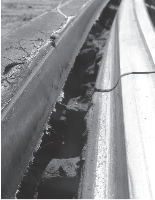
Figure 4.5 Worn side rails on Blackpool track curve, 2006 (Photo: L. Lesley)
