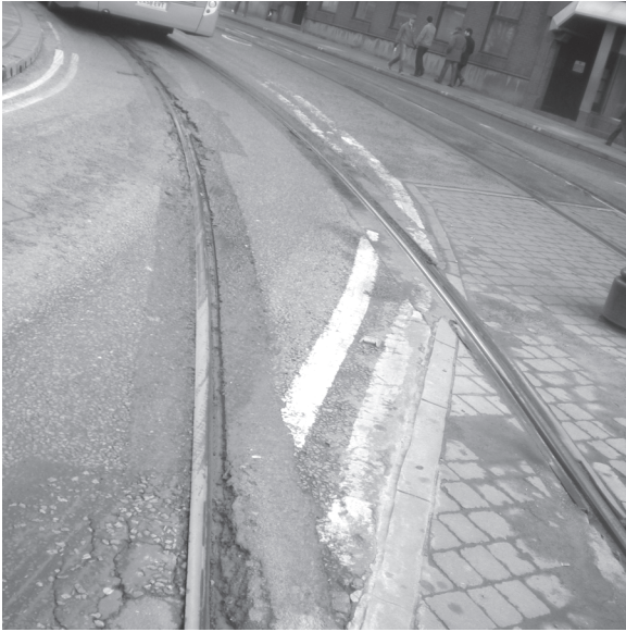
Figure 4.12 Track damage in Manchester, 2009 (Photo: L. Lesley)
