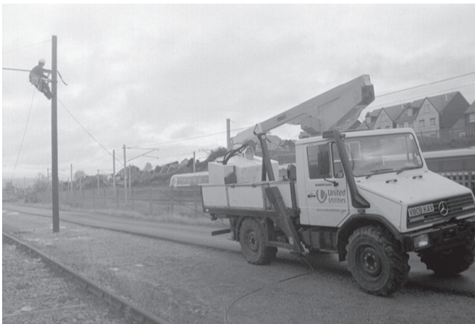
Figure 4.26 Wooden pole used at Carnforth (Photo: L. Lesley)
