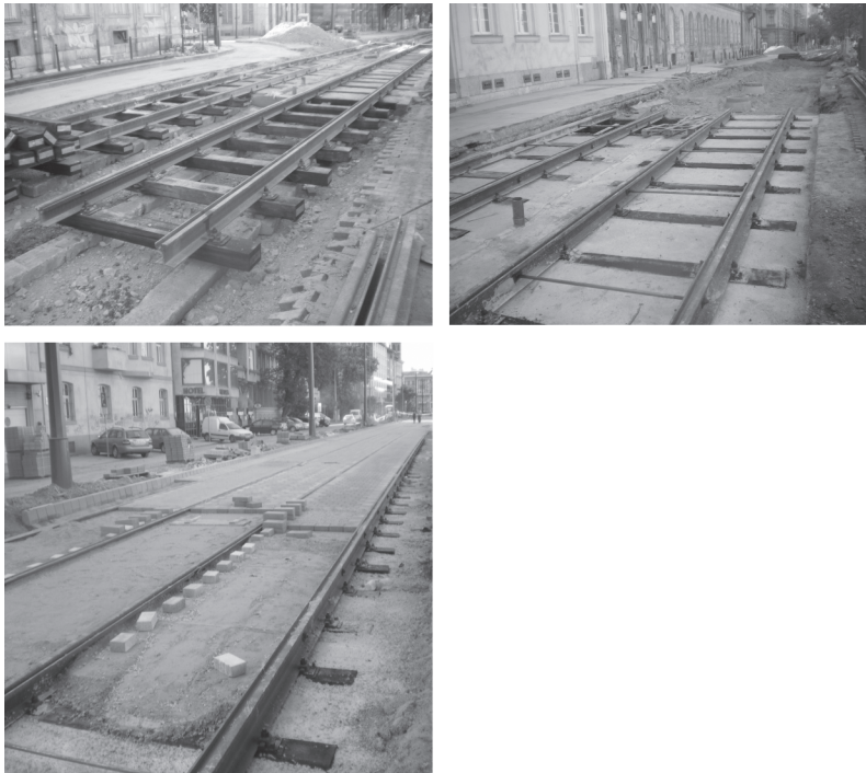
Figure 4.32 Budapest embedded-track-laying sequence, 2009: (top left) track panels on concrete strip foundations, (top right) mass concrete poured to rail bottom (note the gauge bars), and (bottom) sand compacted as base for stone block road surface (Photos: L. Lesley)
