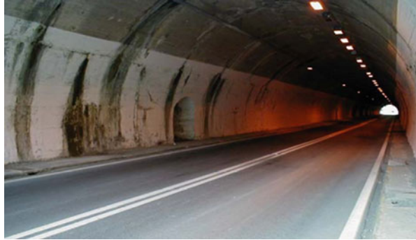
Fig. 6.58 Damages caused by inflows in an operating road tunnel
