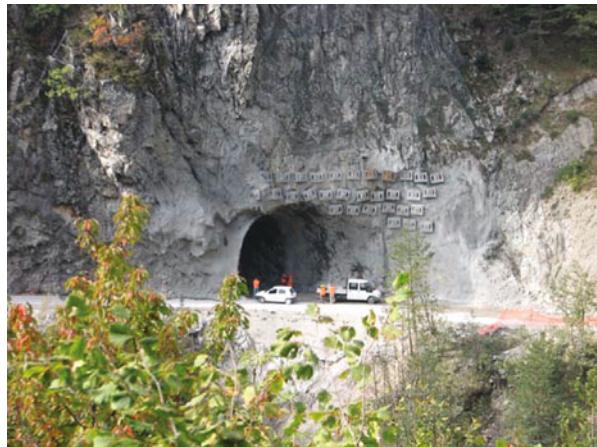
Fig. 2.6 Tunnel portal affecting the slope obliquely: stabilization with tie rods. (By Pizzarotti)
