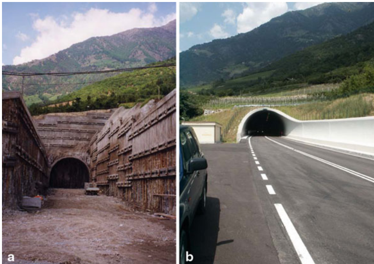
Fig. 1.19 An example of a portal stabilized by means of retaining walls with anchors a during construction, b final configuration. (By Pizzarotti)
