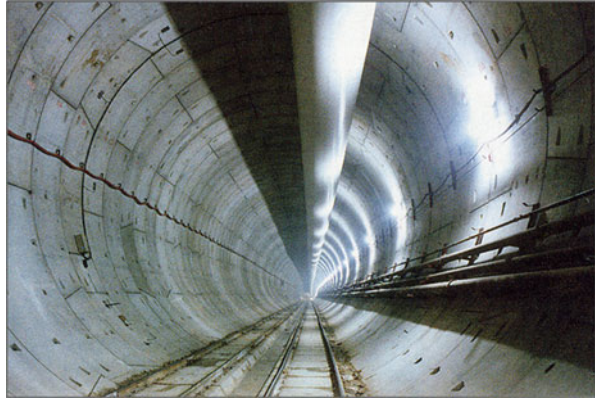
Fig. 6.66 Tunnel lined with precast segments; notice the slots for longitudinal and transversal bolts. (By Pizzarotti)
