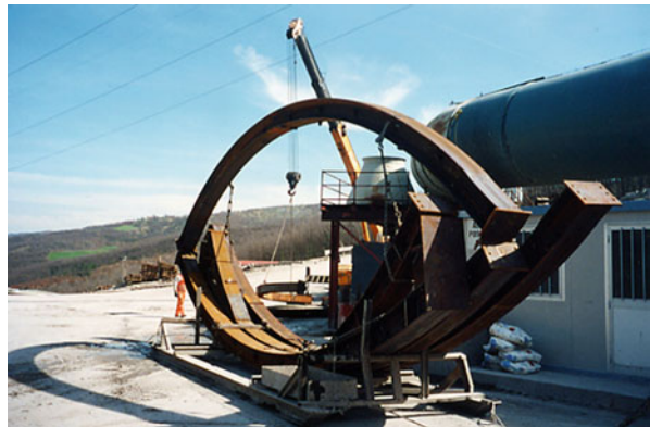
Fig. 6.51 Steel profile ribs
