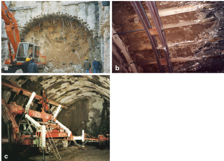
Fig. 6.42 Forepoling (from top ). a portal area with forepoles on the contour and jet-grouting columns at the face. b detail of the forepoles on the steel ribs. c implementation of forepoles on the tunnel contour. (By Pizzarotti)
