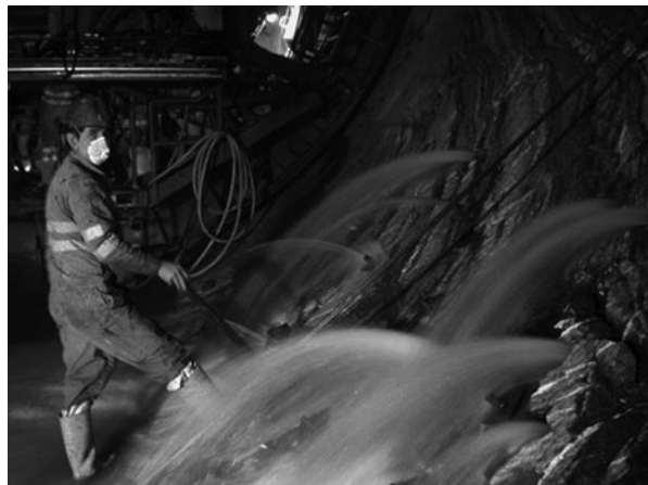
Fig. 2.12 Example of tunnel inflow during excavation works. (Wilhelm and Rybach 2003)
