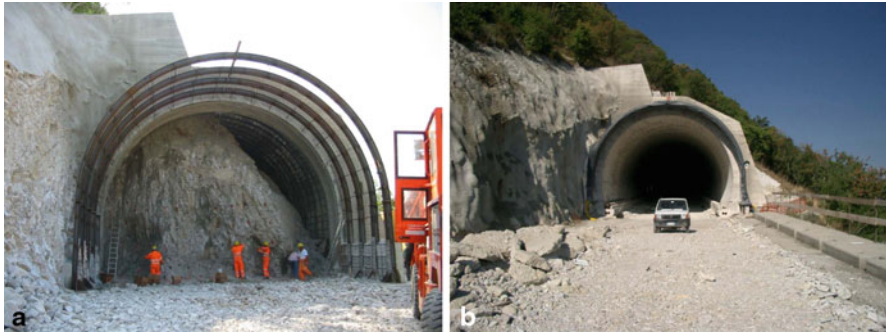
Fig. 2.7 Tunnel portal affecting the slope obliquely: in this case, stabilization structures were: a placement of tie rods on a reinforced concrete head-beam and a steel ribs-reinforced portal, b completion of the reinforced concrete structure. (By Pizzarotti)
