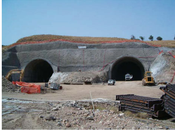
Fig. 1.17 An example of a tunnel portal with nailing of the slope. (By Pizzarotti)
