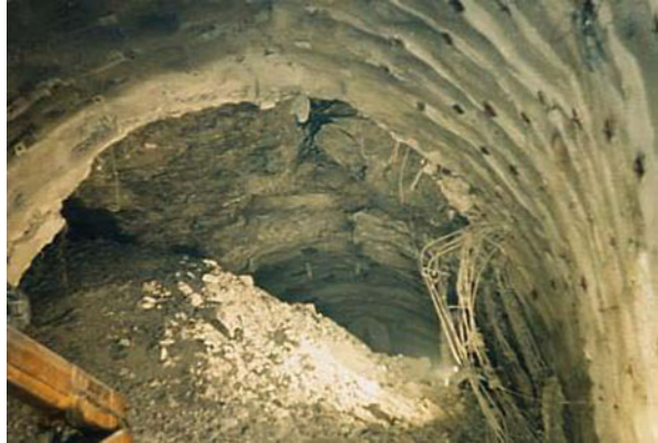
Fig. 1.1 Collapse due to block instability. (By Pizzarotti)
