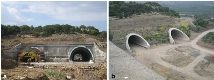
Fig. 1.18 Stabilization of a tunnel portal by retaining walls with anchors a during construction, b final configuration. (By Pizzarotti)
