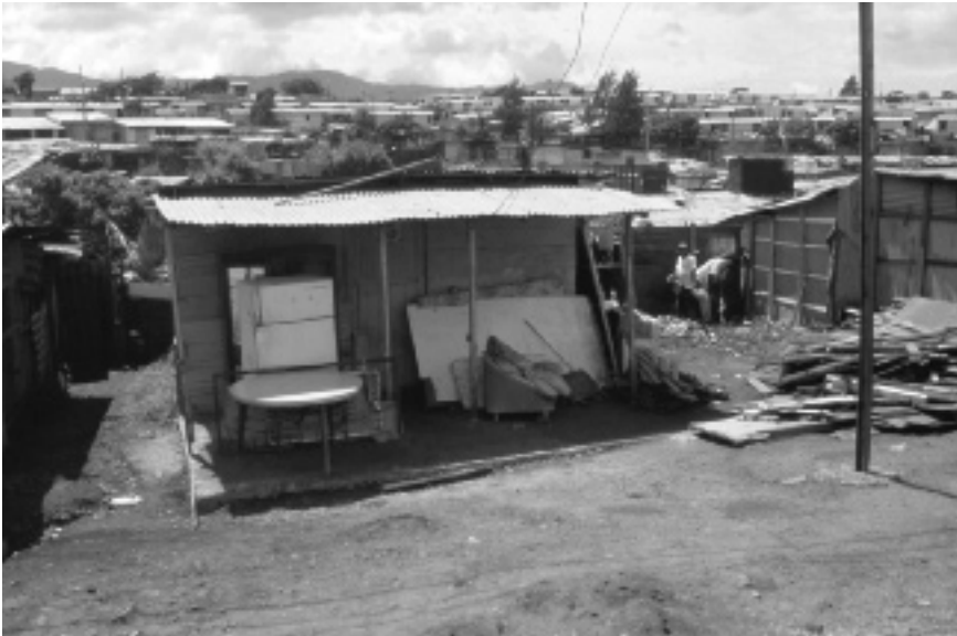
7.3 Reconstruction of a shack under way through mutual aid in an informal settlement in San José, Costa Rica (Harry Smith)
