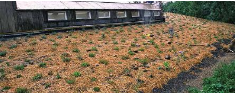
FIGURE 43.3. This living roof at the Upland Hills Ecological Awareness Center near Detroit, Michigan, sports a growing medium of volcanic stone, with a thin layer of earth and straw planted with sedums, which will eventually grow to cover the entire roof. Plants may need
