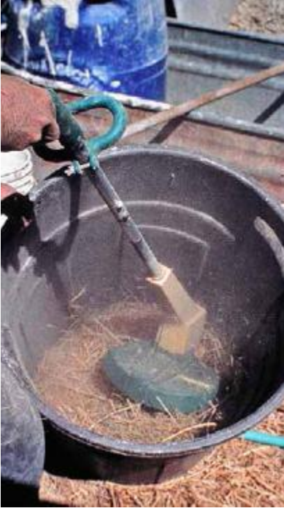
FIGURE 48.2. Breaking up straw for fine plaster using a weed whacker. [Credit: Janine Björnson]
