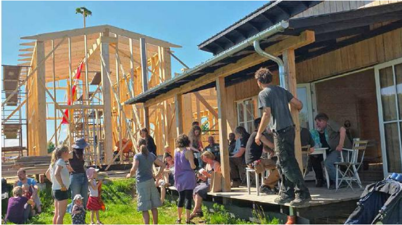
FIGURE 64.5. The wreath above the new house signals that this is a party to celebrate the completion of the roof structure. The community comes together for both the work and the celebrations. [Credit: Lukas Wassberg]
