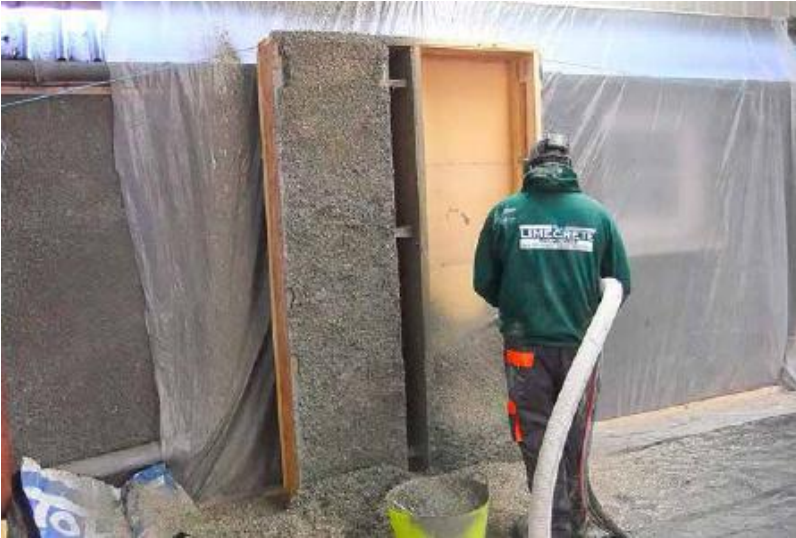
FIGURE 32.4. Hempcrete being sprayed onto a permanent shuttering board by the Limecrete Company, UK, to create a prefabricated panel. [Credit: Tom Woolley]
