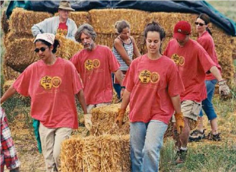
FIGURE 51.1. The empowerment of volunteers and the community is one of the greatest attributes of natural building. Here, a crowd of friends and strangers come together as one team to achieve a common goal. [Credit: Michael Rosenberg]
