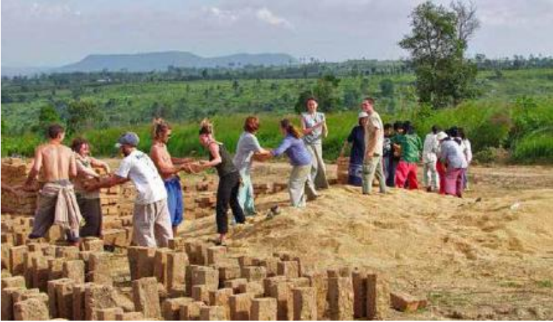
FIGURE 57.4. A human chain of 100 international participants carries adobe bricks from the brickyard to the building site on the first day of the Mun Yeun encampment. Working together towards a common goal helped us to quickly break down cultural and language barriers. [Credit: Janell Kapoor]
