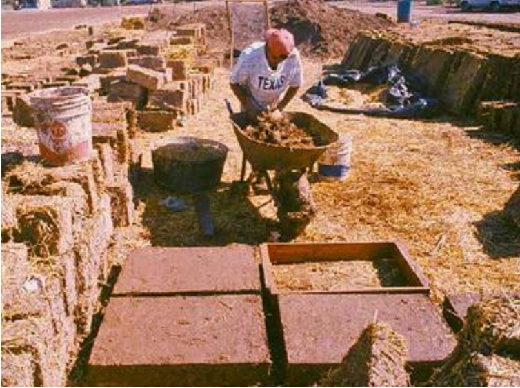
FIGURE 24.7. In Ciudad Obregon, the center of a grain-growing region in northern Mexico, the use of high-fiber adobes has become commonplace. These large blocks will be used to create insulating ceilings. [Credit: Catherine Wanek]
