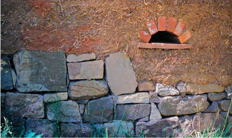
FIGURE 22.2. This small cob building in Oregon has a dry-stacked stone foundation. Stone stacked without mortar is one of the most ecological ways to build a foundation, but it can be vulnerable to intrusion by water and small animals, and to damage from earthquakes. [Credit: Michael G. Smith]
