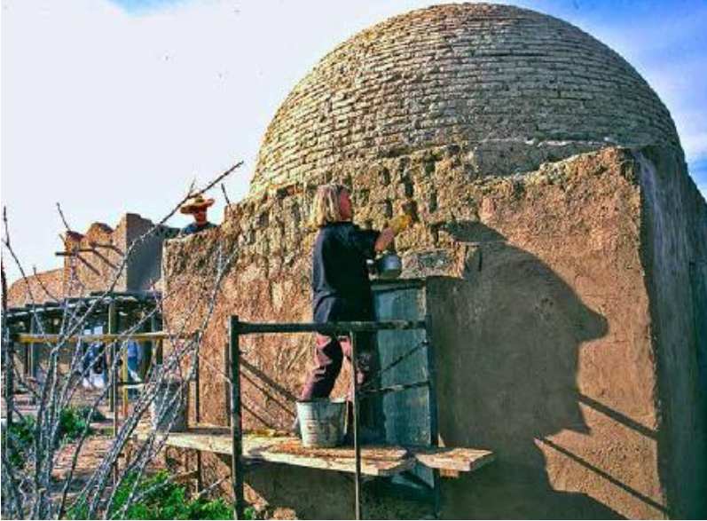
FIGURE 53.4. Woodless construction has been popularized in the US largely due to the efforts of Simone Swan in Presidio, Texas, who was an early promoter of the work of the Egyptian architect Hassan Fathy. Here an earthen dome is replastered by an intern during a workshop. [Credit: Catherine Wanek]
