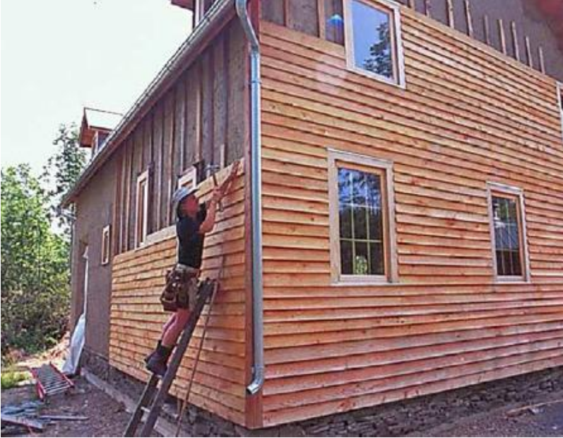
FIGURE 13.5. The vented rainscreen system is appropriate for marine climates and extreme moisture locations. It requires a minimum \frac{1}{4} in. (0.6 cm) gap between the siding and a weather-resistant air barrier behind it (in this building, lime-stabilized earthen plaster). Flashing and trim details need to be worked out in advance. This straw-clay home in Ithaca, New York, was built by Sarah Highland. [Credit: Catherine Wanek]
