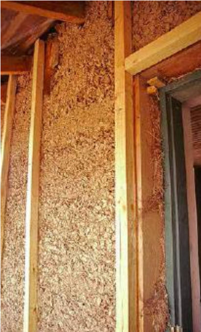
FIGURE 33.3. This woodchip-clay wall in Belarus will be covered with wooden siding for weather protection. The “rainscreen siding” will be attached to the furring strips, with a ventilated air space between the siding and the clay wall. [Credit: Catherine Wanek]
