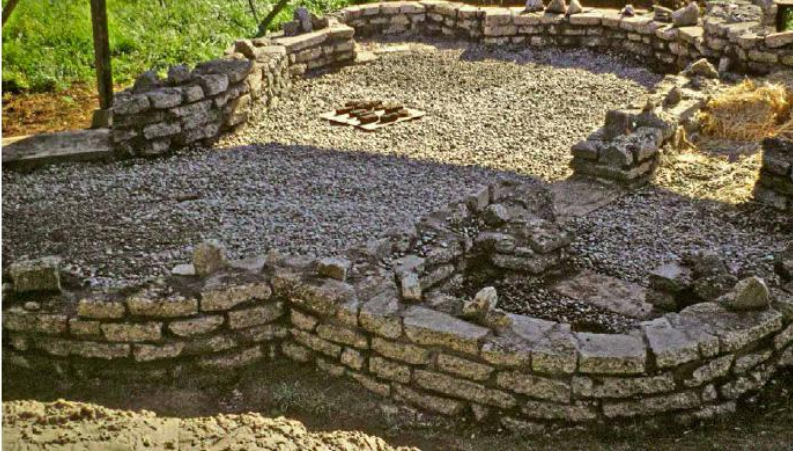
FIGURE 22.1. An urbanite foundation for a cob house, made of broken pieces of concrete sidewalk with a cement-sand mortar. Urbanite’s flat shapes and regular thickness make it easy to stack in stable courses, and it is readily available in urban areas, often for free. “Dinosaur spines” projecting upwards from the middle of the stem wall will help lock the cob walls to the foundation. [Credit: Eric Hoel]
