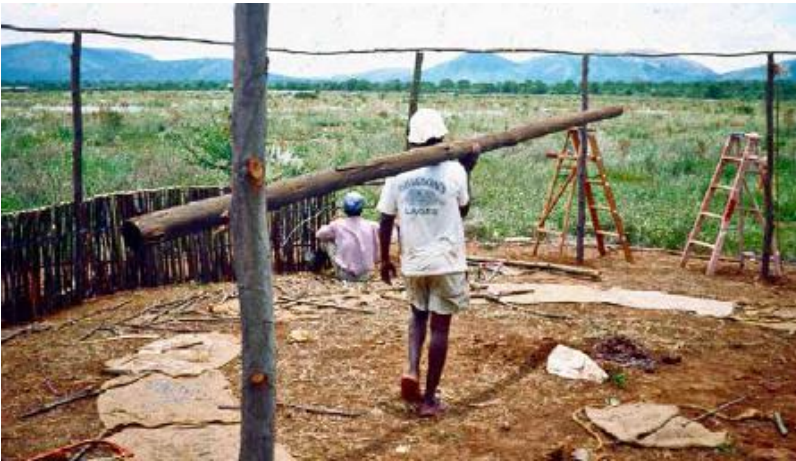
FIGURE 61.3. The community gathering space (Lekgotla) under construction. This design was based on traditional Tswana architecture. [Credit: Joseph F. Kennedy]
