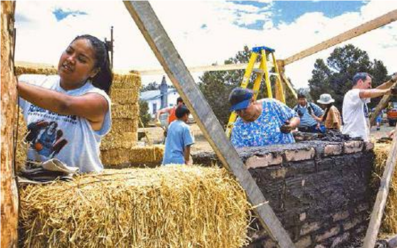
FIGURE 59.2. Builders Without Borders worked with the National Indian Youth Leadership Project (NIYLP) to build an earth-plastered straw bale hogan near Laguna Pueblo. [Credit: Catherine Wanek]
