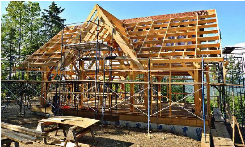
FIGURE 13.4. This lattice-frame roof structure creates a 16-in. (40.6-cm) cavity for insulation, while minimizing thermal bridging in the wooden frame. The 2 \times 8 rafters run vertically, with 2 \times 8 purlins attached horizontally on top. [Credit: Ace McArleton]
