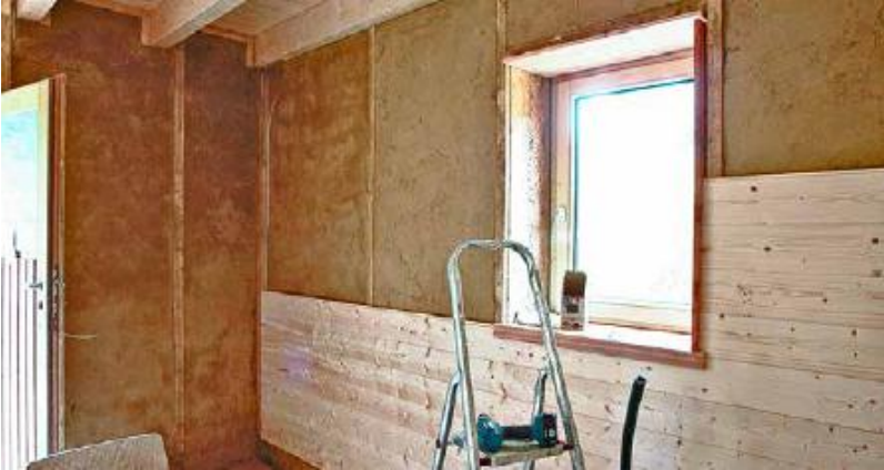
FIGURE 31.7. Even if you plan to finish a straw bale wall with a protective wood siding, it is essential to plaster it first. A continuous coat of clay plaster on both sides seals the bales against air, pests and humidity. Designer/builder Matthias Boehnisch, Windeck, Germany. [Credit: Catherine Wanek]
