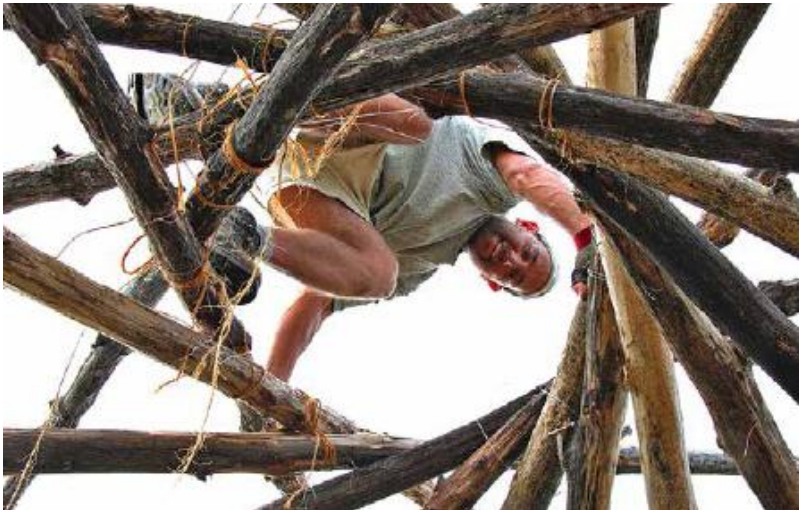
FIGURE 64.1. The author looking down through the oculus of a reciprocal roof that he helped install on a cob cottage at Dancing Rabbit Ecovillage. When building a reciprocal roof, the first rafter is supported by a “Charlie stick.” Once the remaining rafters are in place, the geometry is self-supporting and the Charlie stick can be removed. [Credit: Mark Mazziotti]
