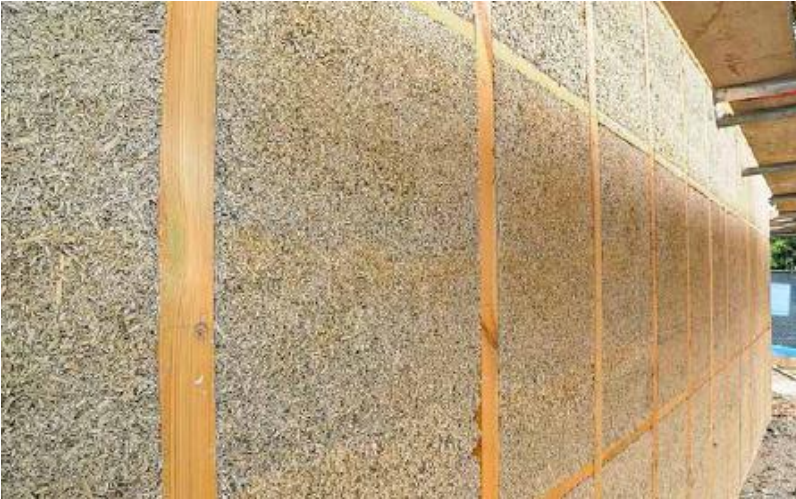
FIGURE 32.1. A hempcrete wall under construction showing the structural timber frame. When plastered, this assembly is insulating and airtight. [Credit: Miles Yallop Limecrete Co., UK]
