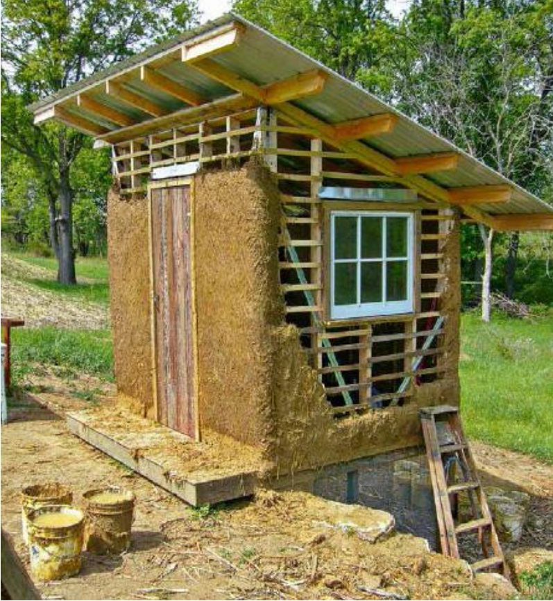
FIGURE 64.2. A modern wattle-and-daub application on the author’s outhouse. The plaster is a mixture of clay and crushed sorghum stalks or “pummies,” left over from sorghum syrup production. The long fibers are draped over the lath strips with a shingling effect. The sugars from the sorghum may have fermented this plaster; it has endured six years of driving rains in good repair. [Credit: Mark Mazziotti]
