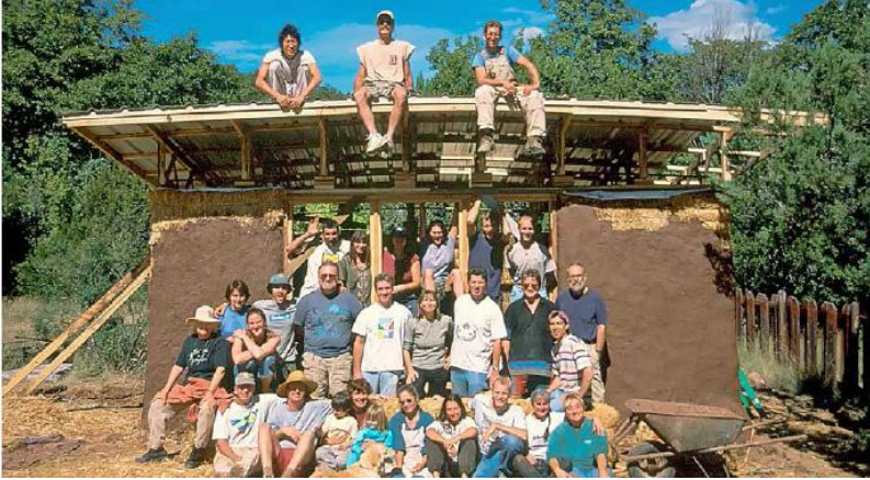
FIGURE 59.5. A Builders Without Borders straw bale training workshop in Kingston, New Mexico. [Credit: Pete Fust]
