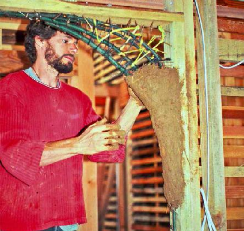
FIGURE 14.5. Michael G. Smith transforms a rectangular framed opening into an earthen archway by sculpting straw-rich clay over an armature of green sticks, nails and baling twine. The lathed interior walls of this northern California home will later be filled with woodchips and clay, with a cob wall separating the living space from the solarium. Earthen plasters will seamlessly meld the different materials for a unified appearance. [Credit: Michael G. Smith]
