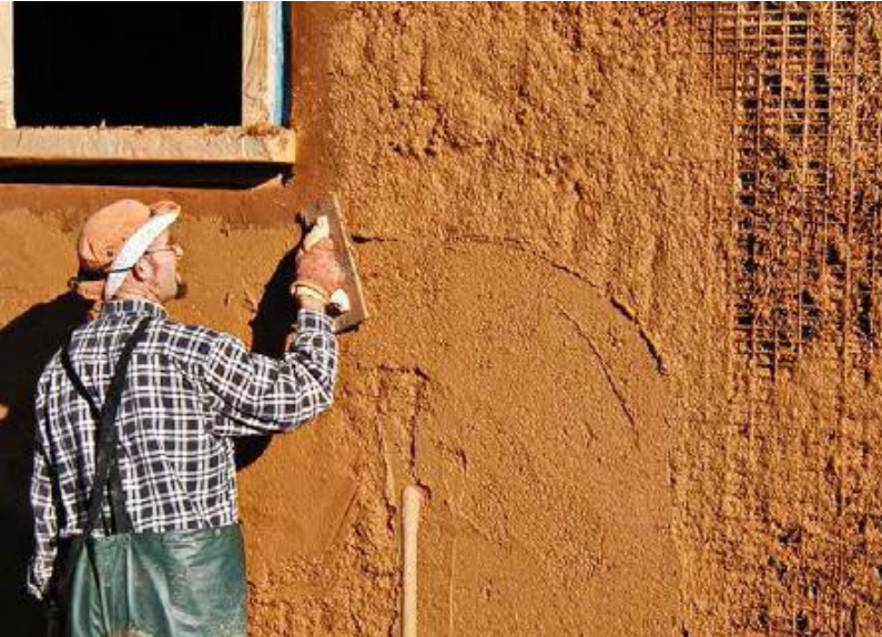
FIGURE 48.1. Earth plaster being troweled smooth after having been pneumatically sprayed onto the straw bale walls of Ridge Winery, Healdsburg, California. [Credit: Joseph F. Kennedy]
