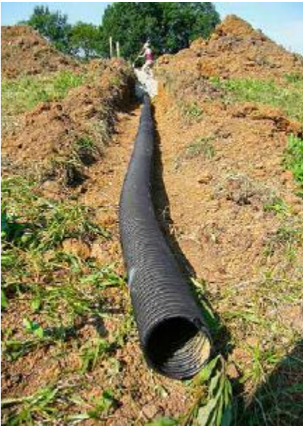
FIGURE 22.5. The bottom of a rubble trench should slope downhill “to daylight.” Sometimes this requires extending the trenches and the drainage pipe far from the building. [Credit: Mark Mazziotti]
