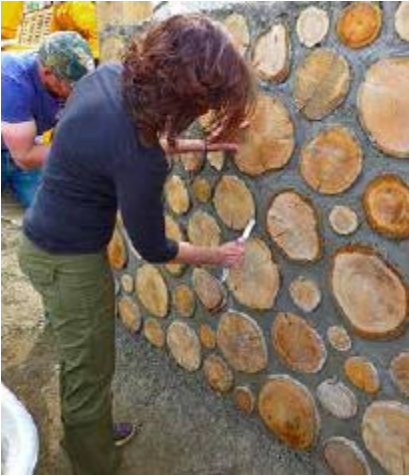
FIGURE 30.5. Pointing the mortar joint — here with a butter knife — is a very important part of the cordwood building process. Pointing maximizes the friction bond between the log ends and the mortar, beautifies the wall, helps repel water on the exterior; and lessens dust and cobweb buildup on the interior. [Credit: Jaki Roy]
