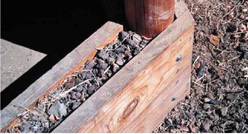
FIGURE 22.3. Novel building solutions often arise out of the desire to use locally available materials. At Emerald Earth Sanctuary in Northern California, there is no stone suitable for building, but there is an abundance of trees, including rot-resistant redwood. This foundation for a light straw-clay wall is made of site-milled redwood boards bolted onto either side of the structural posts, with the cavity between filled with lava rock for insulation and drainage. The drainage layer extends below the stemwall to help protect the walls and the earthen floor from water. [Credit: Michael G. Smith]
