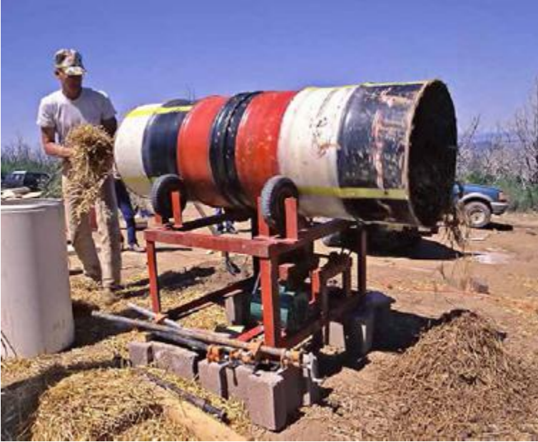
FIGURE 33.7. Alfred adds straw, clay and water into one end of his mixer as it turns. Out of the other end comes mixed straw-clay, ready to be packed into a wall. [Credit: Catherine Wanek]
