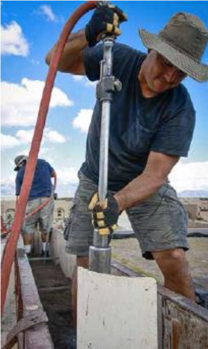
FIGURE 26.3. A modern rammed earth crew utilizes pneumatic tampers and steel form work to compress the clay, sand and cement mixture. In the foreground, a cut-off piece of PVC pipe is placed in the corner so that the finished rammed earth wall will have a rounded corner. [Credit: David Shaw]
