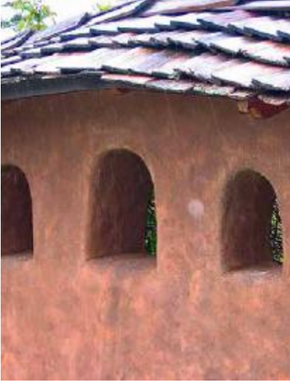
FIGURE 48.8. This plastered cob wall is protected from the elements by a shake roof. [Credit: Joseph F. Kennedy]
