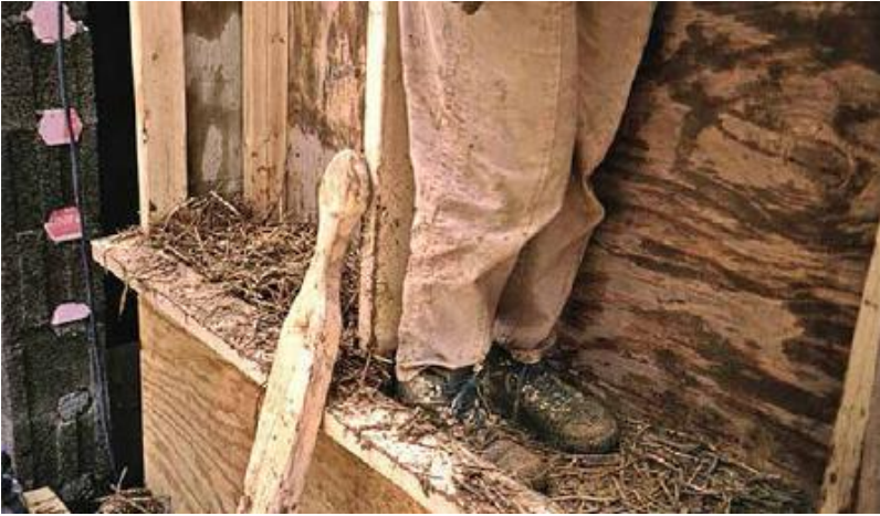
FIGURE 33.4. These 12 in. thick walls (30.5 cm) are tamped by walking in them. A tamper fashioned from a 2 × 6 is used to tamp corners. Note the reinforced plywood slipforms and the “Larsen truss” framing that allows the straw-clay insulation to run continuously through the middle of the wall. [Credit: EcoNest Co.]
