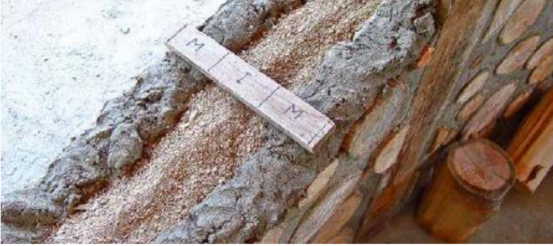
FIGURE 30.2. A “MIM-stick” helps the builder judge the width of the three components of the mortar joint. MIM stands for Mortar-Insulation-Mortar. This one, for a 12 in. (30 cm) cordwood wall, shows the width of the 4 in. (10 cm) inner mortar joint, the 4 in. of the sawdust insulation and the 4 in. outer mortar joint. [Credit: Jaki Roy]
