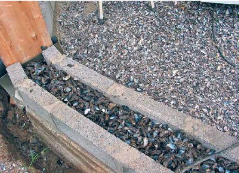
FIGURE 45.5. In Denmark, where mussel shells are available as waste from the seafood industry, they are used to provide insulation and drainage in a stemwall and under a floor. [Credit: Catherine Wanek]
