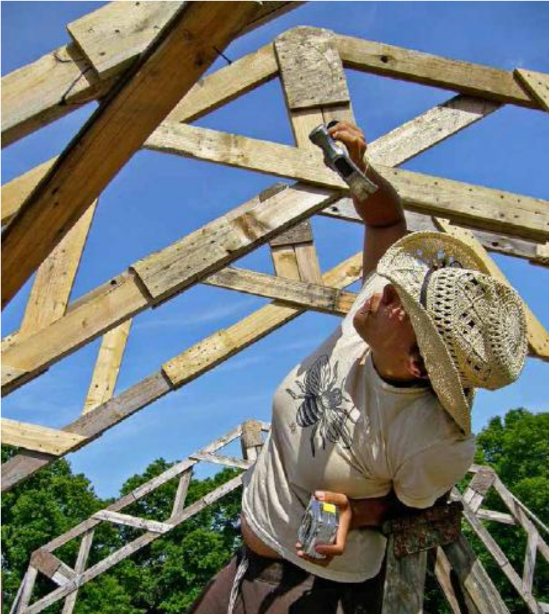
FIGURE 64.4. Intern Monica Chaplin installing a pallet wood truss. The trusses were assembled on the second-floor deck and then erected in place to create the walls and roof for the second floor of the author's house. [Credit: Mark Mazziotti]
