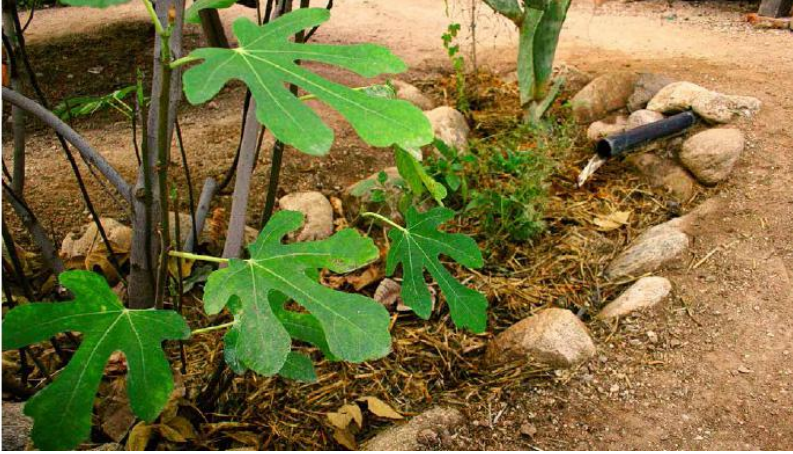
FIGURE 18.7. This greywater drain outlet empties into a mulched and vegetated infiltration basin that also harvests rainwater and surface runoff. The pipe discharges above the mulch to keep roots from growing into and clogging the pipe. (Reproduced with permission from Rainwater Harvesting for Drylands and Beyond , Volume 1, 2nd Edition, by Brad Lancaster. HarvestingRainwater.com .) [Credit: Brad Lancaster]
