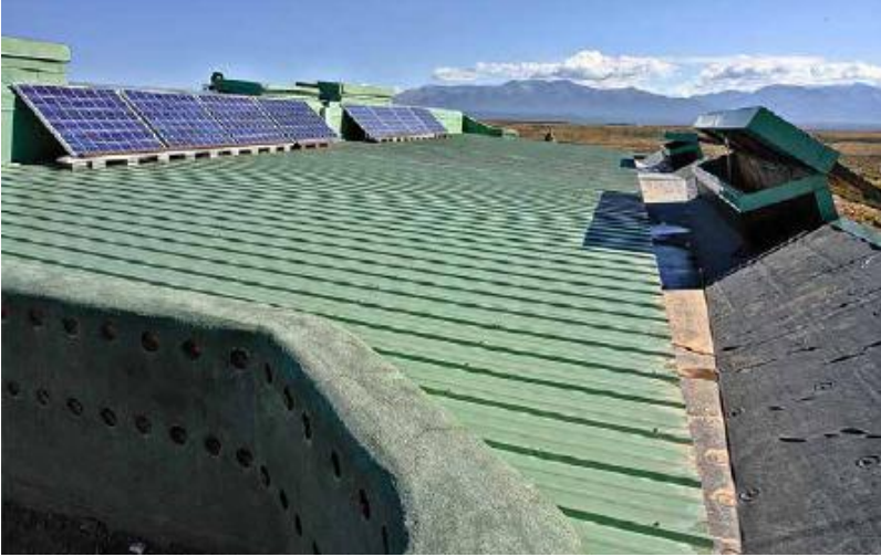
FIGURE 40.3. This long-lasting metal roof harvests rain which is stored in a cistern for the use of residents, while the photovoltaic system harvests solar energy, to power their electrical needs. Note the ventilation ports on the right. [Credit: Catherine Wanek]
