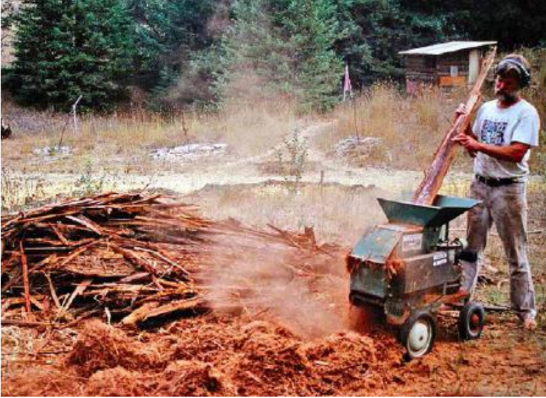
FIGURE 45.4. At Emerald Earth Sanctuary in California, redwood bark left over from onsite lumber milling was run through a chipper-shredder. The resulting material — lightweight, rot-resistant and fire-resistant — was used as roof insulation. [Credit: Michael G. Smith]
