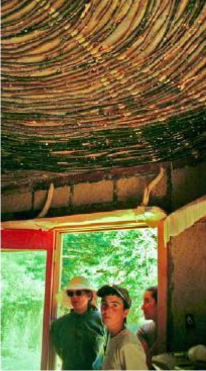
FIGURE 19.3. Small saplings and branches harvested as part of forest management practices can find many applications in natural buildings. Here, branches have been attached to the rafters in preparation for an earthen plaster in the author’s home at Emerald Earth Sanctuary. [Credit: Michael G. Smith]
