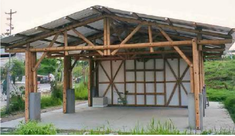
FIGURE 38.2. This small bamboo pavilion features concrete foundation piers for additional structural strength and to protect the bamboo from water damage. [Credit: Darrel DeBoer]
