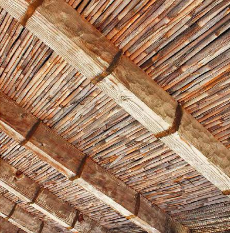
FIGURE 21.5. Reeds have been lashed with rawhide to wooden rafters to faithfully recreate the 18th-century Spanish techniques used to build the Presidio in Santa Barbara. [Credit: Joseph F. Kennedy]
