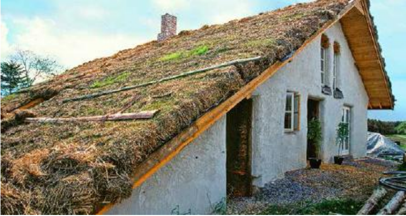
FIGURE 43.2. This layer of straw bales will gradually decompose and provide a growing medium for a living roof. The roof structure must be strong enough to support the loads of straw that will at some point become saturated with water. [Credit: Catherine Wanek]
