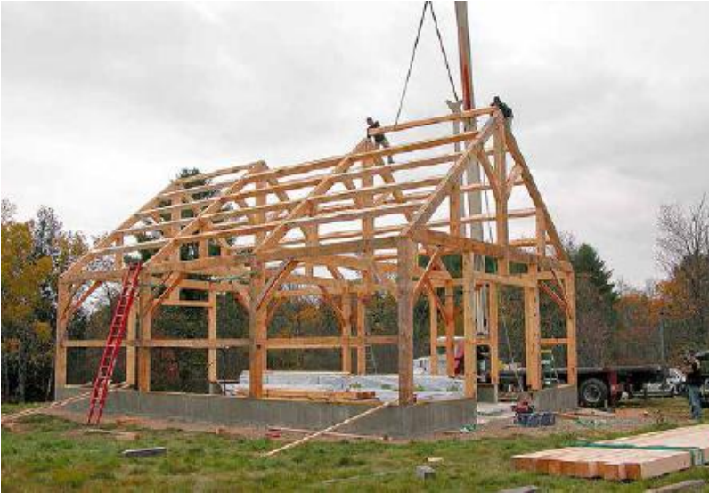
FIGURE 36.7. This four-bent frame uses king post trusses to create a clear span first-floor area. The bents span 30 ft., and the bay spacing is 16 ft., creating a 30 x 48 ft footprint. The bents are connected using top plates at eaves level, wall purlins and roof purlins. Note the crane being used to lift the heavy timbers into place. [Credit: Steve Chappell]
