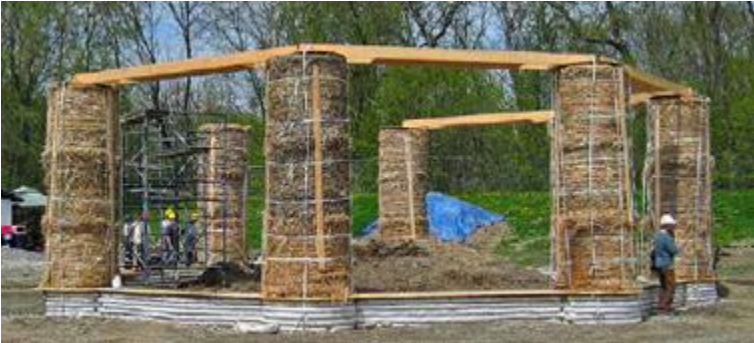
FIGURE 32.8. The structural columns for this community performance space in Madoc, Ontario, Canada, are formed from large round hemp bales. [Credit: Chris Magwood]
