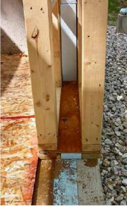
FIGURE 13.3. This double-stud wall eliminates thermal bridging and creates space for more insulation while incorporating standard framing practices. In this picture, two 3.5 in. (9 cm) stud walls with a 5 in. (12.7 cm) space in between for insulation create a super-insulated wall assembly. The structural loads can be borne either by the interior or exterior frames, or both. [Credit: Robert Riversong]
