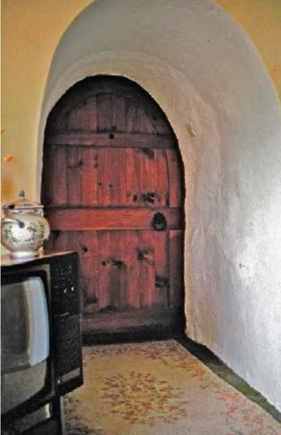
FIGURE 25.1. The walls of traditional cob homes in Britain ranged from three feet thick to occasionally nearly twice that, as shown by this doorway in an old Devon home. These extra-thick walls produced a stable interior temperature despite the cool, damp climate. [Credit: Catherine Wanek]
