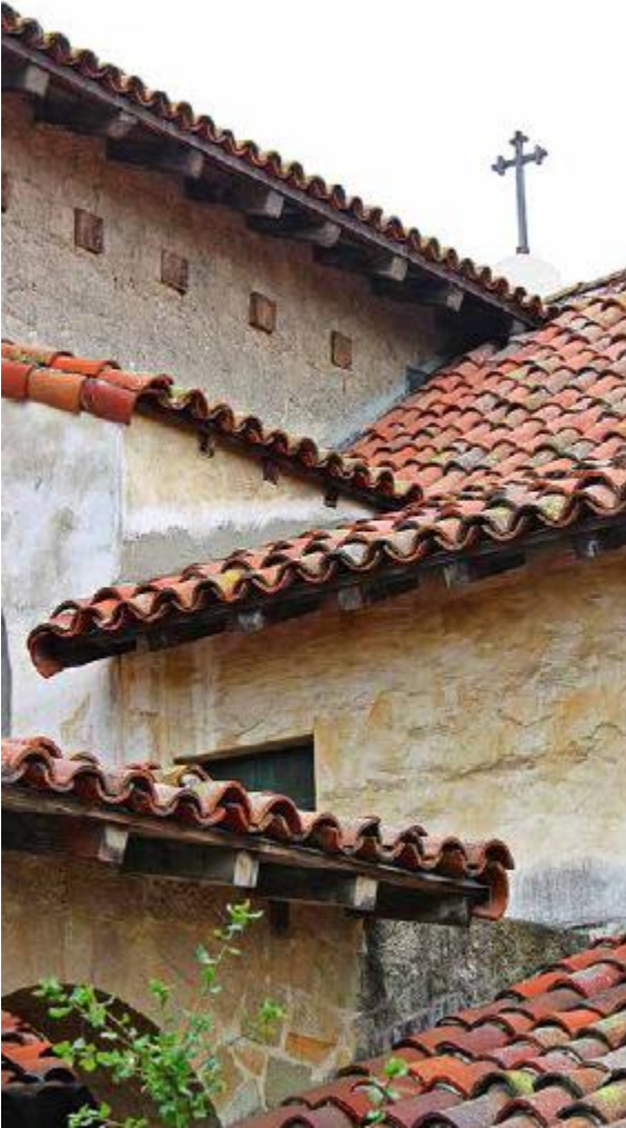
FIGURE 42.1. A cascading series of clay tile roofs. Santa Barbara Mission, California. [Credit: Joseph F. Kennedy]
