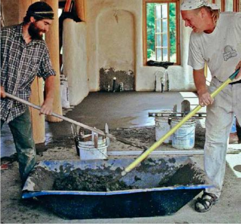
FIGURE 47.5. The final layer of an earthen floor should be one of the last steps in constructing a natural home. All of the finish plaster, carpentry and rough plumbing have been completed in this cob house prior to installing the finish floor. [Credit: Michael G. Smith]
