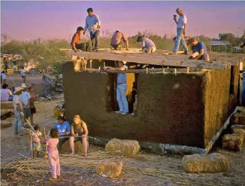
FIGURE 59.1. Working in Ciudad Obregón, Mexico, with extreme budgetary constraints, Athena and Bill Steen evolved a model of self-help housing by organizing week-long hands-on workshops in which participants and local families worked side by side building comfortable homes from locally available materials. [Credit: Catherine Wanek]
