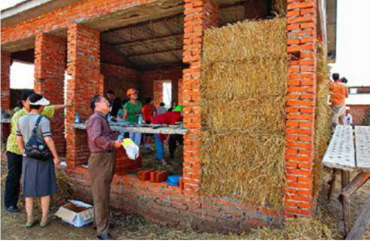
FIGURE 54.3. This ADRA straw bale workshop is implementing a design by architect Kelly Lerner, which was informed by Chinese vernacular homes. In 2005, this ADRA initiative won the United Nations World Habitat Award. [Credit: Catherine Wanek]
