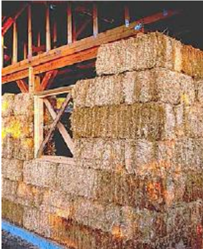
FIGURE 31.4. Straw bales are most often used as “infill” insulation within a structure of wood, steel or adobe. They may be notched around posts, or the bale wall may stand to the inside or outside of structural members, as shown here. [Credit: Catherine Wanek]
