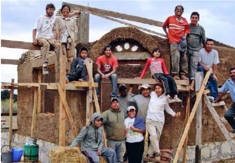
FIGURE 51.2. This demonstration building in Oaxaca, Mexico, was constructed in two weeks as a collaboration between local architect Valentina Marquez Mendez, instructor Michael G. Smith, paid builders and volunteers. Such projects have been instrumental in introducing natural building techniques to communities all over the world. [Credit: Valentina Marquez Mendez]
