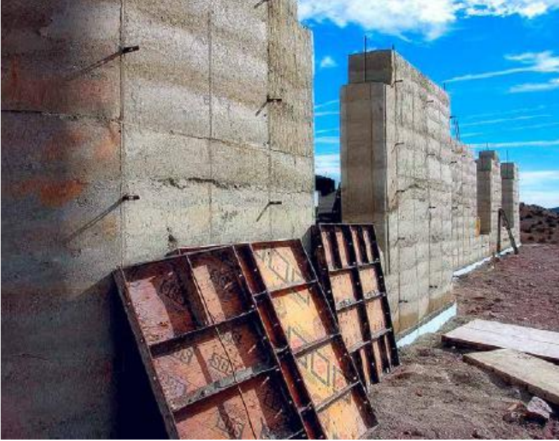
FIGURE 26.4. Soledad Canyon Earth Builders uses locally sourced crusher fines with three percent Portland cement as a “stabilizer.” The cement is dry mixed with the crusher fines, before water is added. Soil mixtures are tested for compressive strength before being used in the construction of a home. [Credit: David Shaw]
