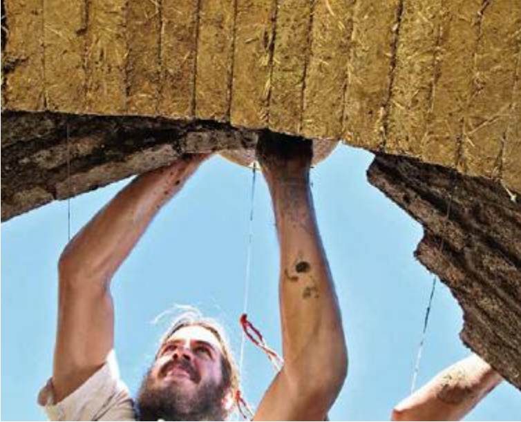
FIGURE 24.9. This Nubian vault is being built of small high-fiber adobes. Straw-rich blocks have many advantages when used overhead: less weight to lift and handle; better insulation; more resistance to seismic forces; and less likelihood of injury in the case of collapse. [Credit: Michael G. Smith]
