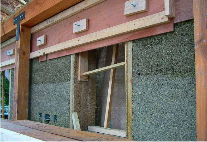
FIGURE 32.2. Detail of temporary plywood forms used to cast hemcrete for the Hemp Cottage, Crossgar, Northern Ireland. [Credit: Rachel Bevan Architects]
