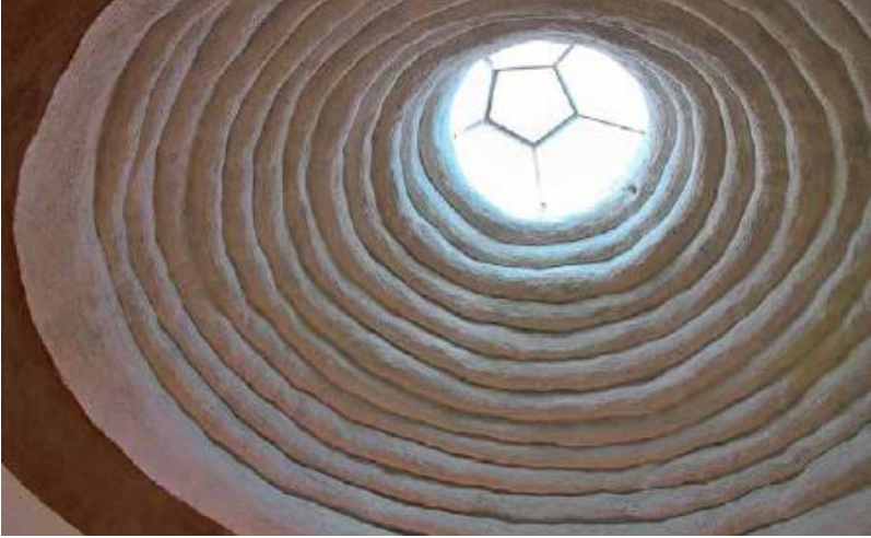
FIGURE 28.3. Tubular earthbags utilized to create a self-supporting dome structure at CalEarth, Hesperia, California. [Credit: Joseph F. Kennedy]
