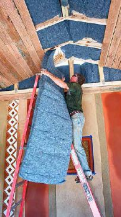
FIGURE 45.3. Cotton batt insulation made from recycled denim material is widely available in the United States. Here, Eric Hempstead installs Ultratouch cotton batts to insulate the roof of a demonstration ecohouse built by Builders Without Borders in Washington, DC. [Credit: Catherine Wanek]
