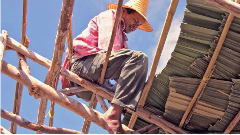
FIGURE 57.5. Local volunteers roofed the village council hall with palm fronds. The fronds were attached to the frame with bamboo “twist ties” split with a machete. [Credit: Janell Kapoor]
