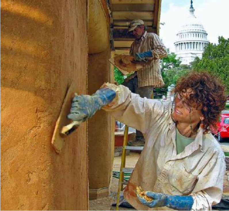
FIGURE 49.3. Lime plasters are applied with a hawk and trowel and smoothed out with a wooden float. Here, Kaki Hunter and Doni Kiffmeyer plaster the BWB Straw Bale Ecohouse at the US Botanic Garden in Washington, DC. [Credit: Catherine Wanek]
