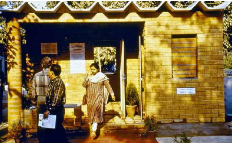
FIGURE 62.4. This demonstration house was built in Delhi in 66 hours. [Credit: Serge Mâini]
