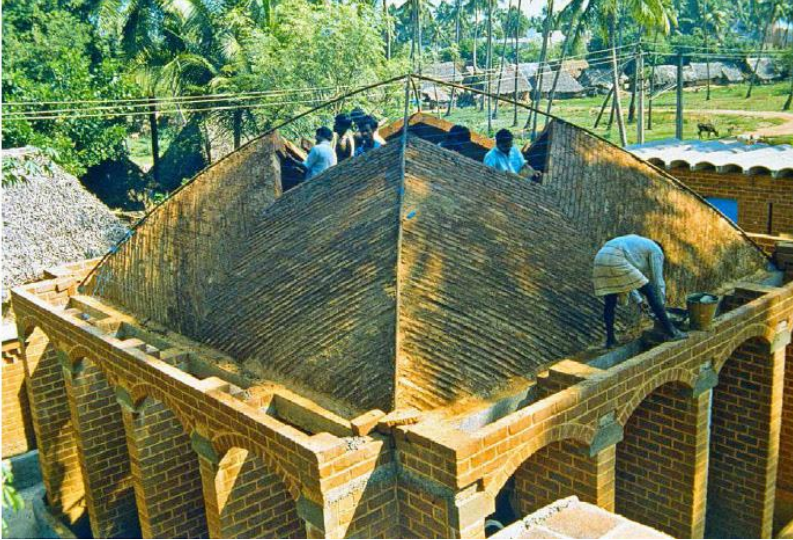
FIGURE 27.4. Construction of a school covered by groined CEB vaults in Auroville, India. [Credit: Serge Maini]
