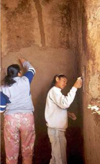
FIGURE 3.2. Many natural building techniques are easy to learn, often without specialized training or expensive tools. This empowers people who would be excluded from the modern construction industry to participate in building their own homes. In Anapra, Mexico, these girls are learning to plaster with clay on the straw bale home that is being built for their family through a collaborative effort led by Builders Without Borders. [Credit: Catherine Wanek]
