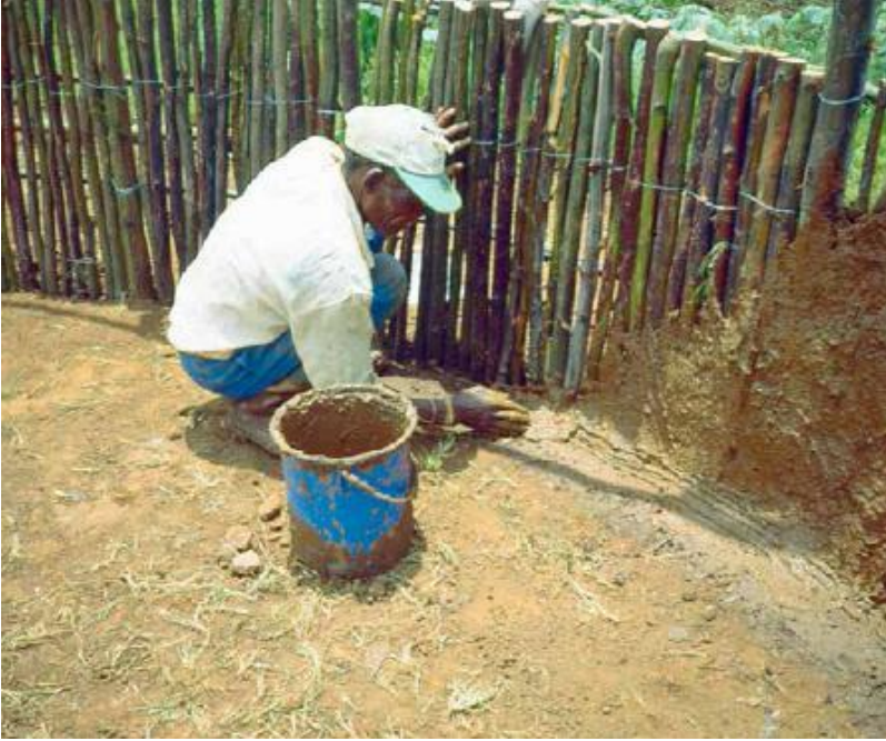
FIGURE 34.4. Plastering a traditional Tswana-style building at Tlholego, South Africa. [Credit: Joseph F. Kennedy]
