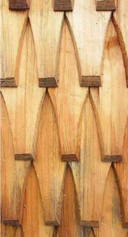
FIGURE 2.5. Wooden shingles, handcrafted from rot-resistant trees, create a long-lasting weather-proofing exterior on a Norwegian Stave Church. [Credit: Tim Tolitson]
