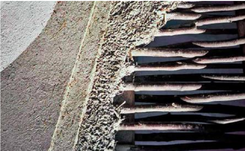
FIGURE 34.1. Detail of plaster layers on a wattle-and-daub panel. [Credit: Joseph F. Kennedy]
