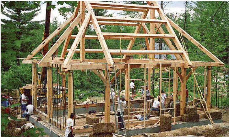
FIGURE 35.5. The frame for the Fox Maple library was cut and assembled during a timber-framing workshop in
