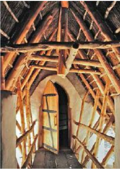
FIGURE 37.3. This earthen house in Balstrop, Texas, utilizes wooden poles for the roof structure and railings. Note thatch above. [Credit: Catherine Wanek]
