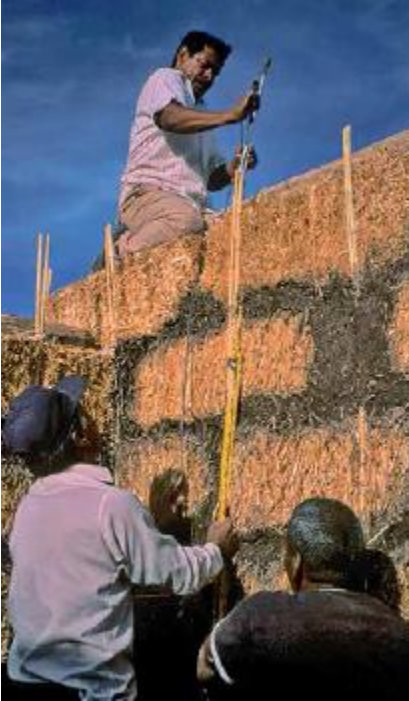
FIGURE 52.1. Creative and appropriate use of available materials is demonstrated by this straw bale project in Mexico. [Credit: Catherine Wanek]
