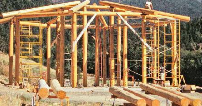
FIGURE 37.1. The community house under construction at the Full Bloom community in Oregon. This building utilizes locally harvested Douglas fir poles for framing. [Credit: Michael G. Smith]
