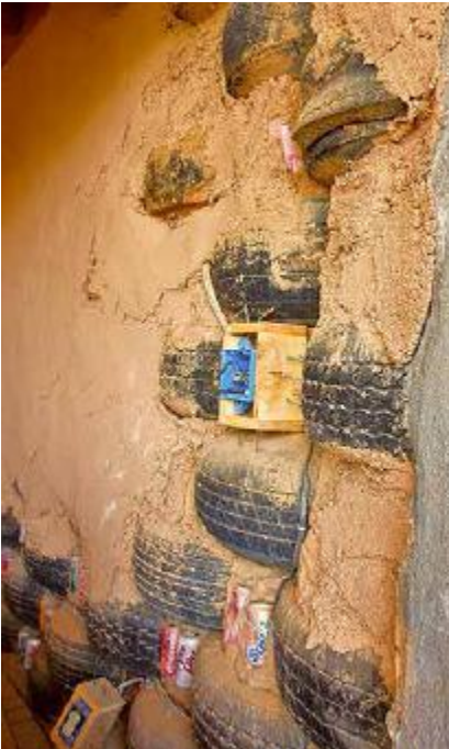
FIGURE 40.2. The walls of an Earthship are built from tires, rammed with dirt. [Credit: Catherine Wanek]
