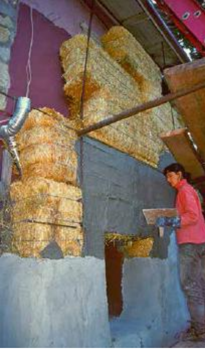
FIGURE 15.2. Creating an insulating straw bale wrap around a steel shipping container. [Credit: Will Coquillette]
