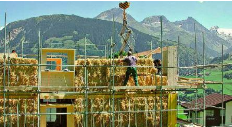
FIGURE 31.10. In the Swiss Alps, where winter snow can pile up to 33 ft. (10 m) high, jumbo straw bales plastered with lime outside and clay inside support the considerable roof loads, plus snow loads. Due to the high insulation value of the four-foot-thick walls, residents can rely almost entirely on solar heating through the cold, but sunny, winters. [Credit: Werner Schmidt]
