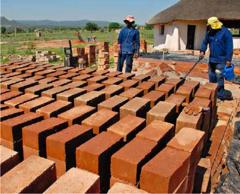
FIGURE 27.2. Compressed earth blocks curing in the sun. Dennilton, South Africa. [Credit: NextAid]
