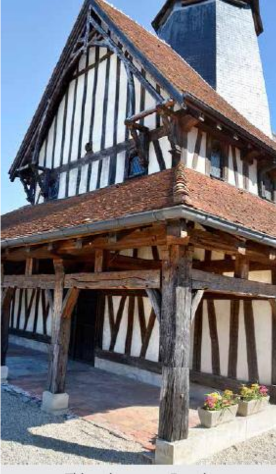
FIGURE 35.1. This 15th-century French timber frame church with wattle-and-daub infill demonstrates that oak timbers, infilled with natural materials, can last for centuries. [Credit: Steve Chappell]
