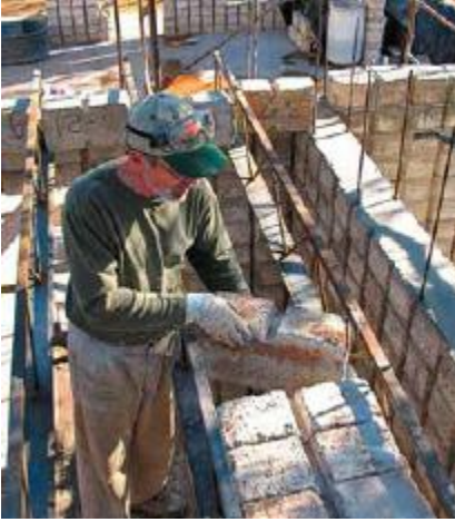
FIGURE 41.4. Eli Sutton built his house from papercrete blocks stacked and reinforced with rebar and cement mortar. In this photo, he is constructing a papercrete roof. When the blocks are all in place, a thick layer of papercrete, reinforced with rebar, will be poured on top. [Credit: Eli Sutton]
