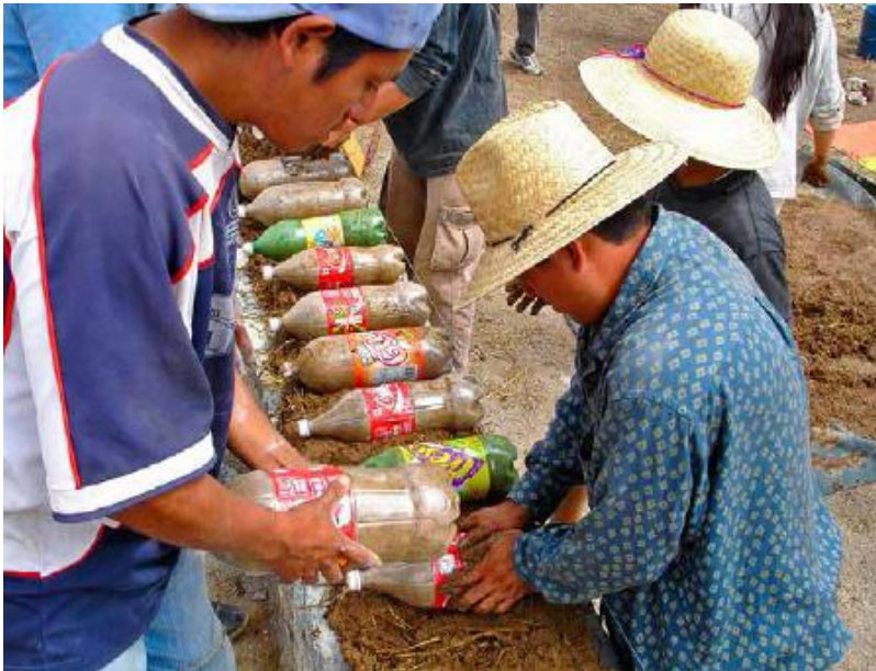
FIGURE 39.2. Plastic bottles can be effectively “upcycled” by filling them with sand, earth or plastic trash (for an insulating unit) and stacking them in mortar to create walls. [Credit: Valentina Mendez Marquez]
