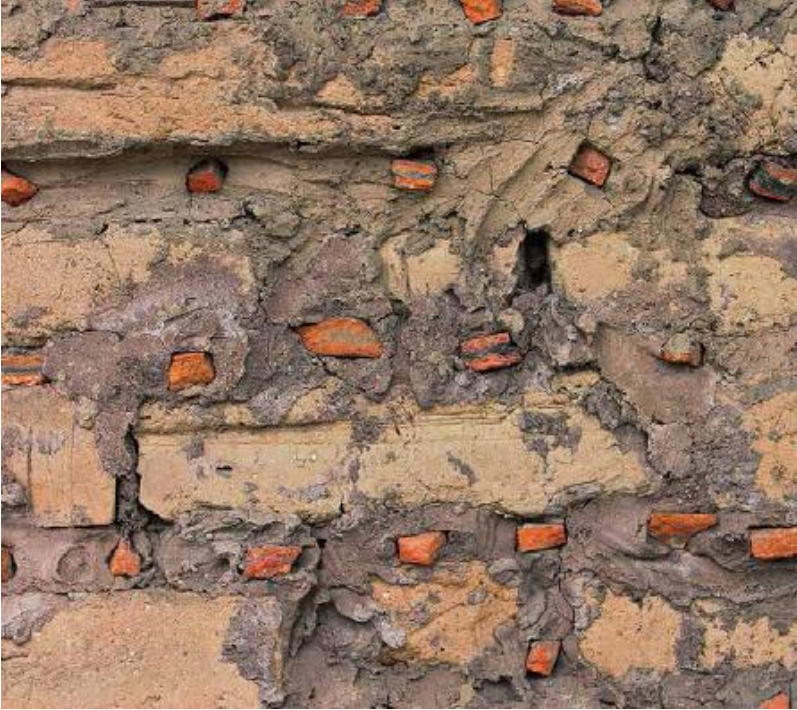
FIGURE 21.9. Broken pieces of ceramic tile are pressed into the mortar of this adobe wall to provide an additional “key” for the initial layer of earth plaster. [Credit: Joseph F. Kennedy]
