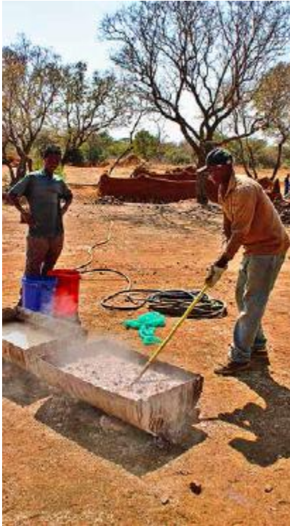
FIGURE 49.2. Mixing quicklime with water is called slaking. Lime plasters are a global tradition, from China to England to South Africa. [Credit: Joseph F. Kennedy]
