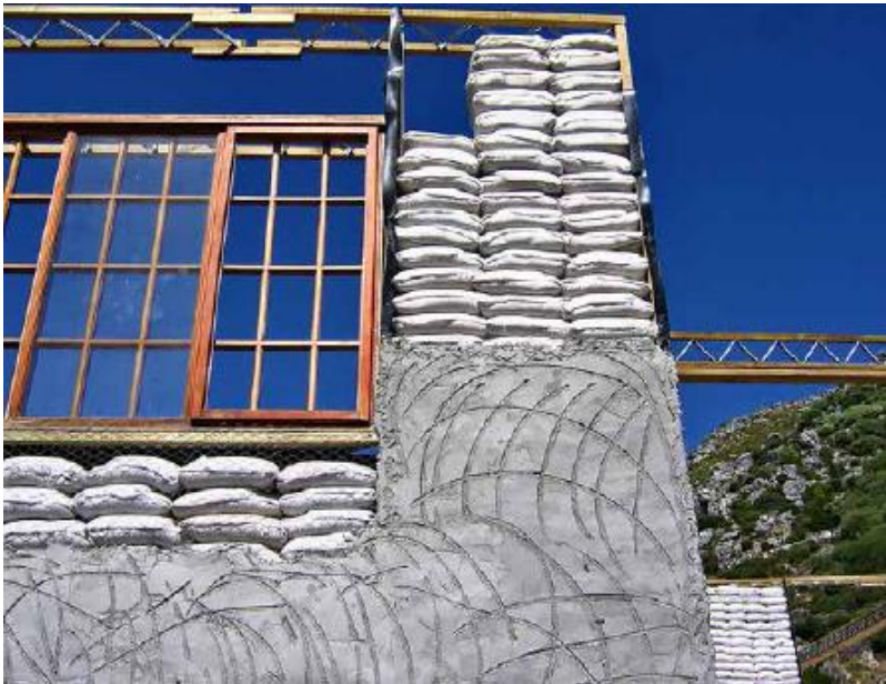
FIGURE 28.5. A unique earthbag system that utilizes plastered sand-filled bags laid between structural frames. Cape Town, South Africa. [Credit: Joseph F. Kennedy]
