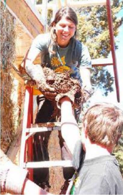
FIGURE 1.4. Natural building techniques allow people with minimal training to work together to build an inexpensive home. These systems often require a lot of labor but little cost in materials and tools. Here, workshop participants apply a base coat of clay plaster to a straw bale wall. [Credit: Catherine Wanek]
