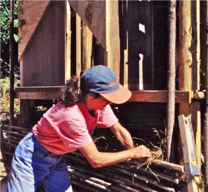
FIGURE 19.4. Stuffing the Hermitage wall cavity with insulation made from site-harvested dried grasses and clay. The round-pole structural frame is also visible. [Credit: Michael G. Smith]
