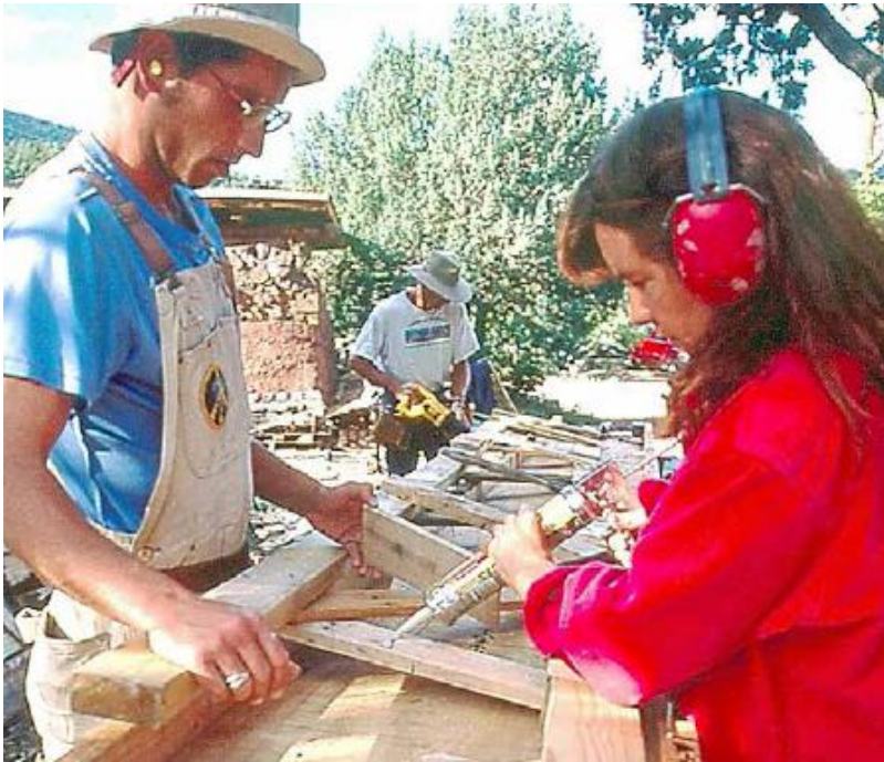
FIGURE 39.4. Making pallet trusses at a Builders Without Borders workshop. [Credit: Catherine Wanek]
