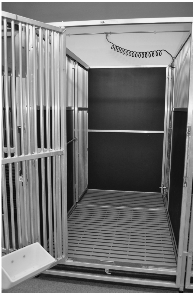
FIGURE 26.3 Permanently fixed large animal run for housing dogs, pigs, sheep, goats, or other larger laboratory animal species. Fixed runs require methods for sanitization in place. (Photo by Michelle Wallace-Fields.)
