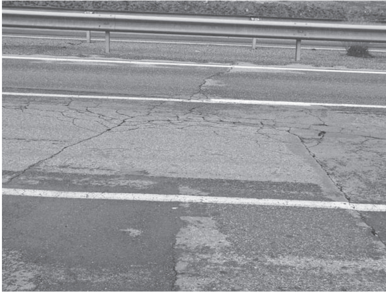
Figure 1. Typical crack pattern observed in an area with hot dry summers and cold winters.
