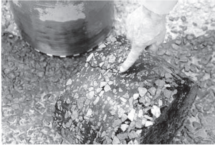
Figure 1. Core from motorway showing top-down cracking.
