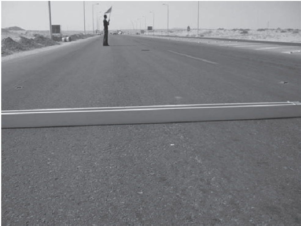
Figure 3. Pavement condition of Khursaniyah access road.
