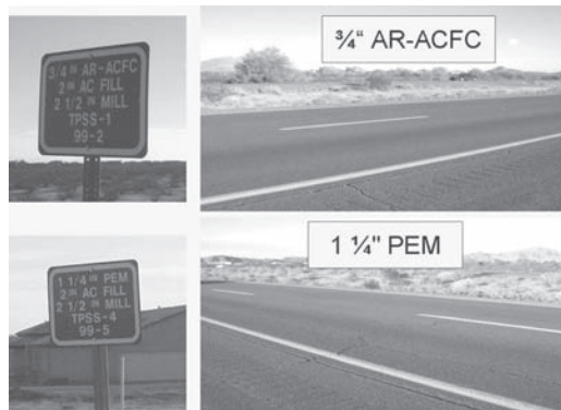
Figure 4. Example of pavement surface condition in 2007 for two pavement types after eight years of service.
