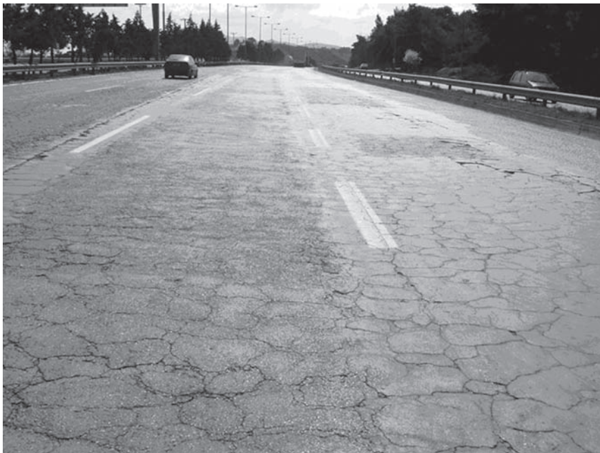
Figure 1. Typical distressed section of the existing pavement.
