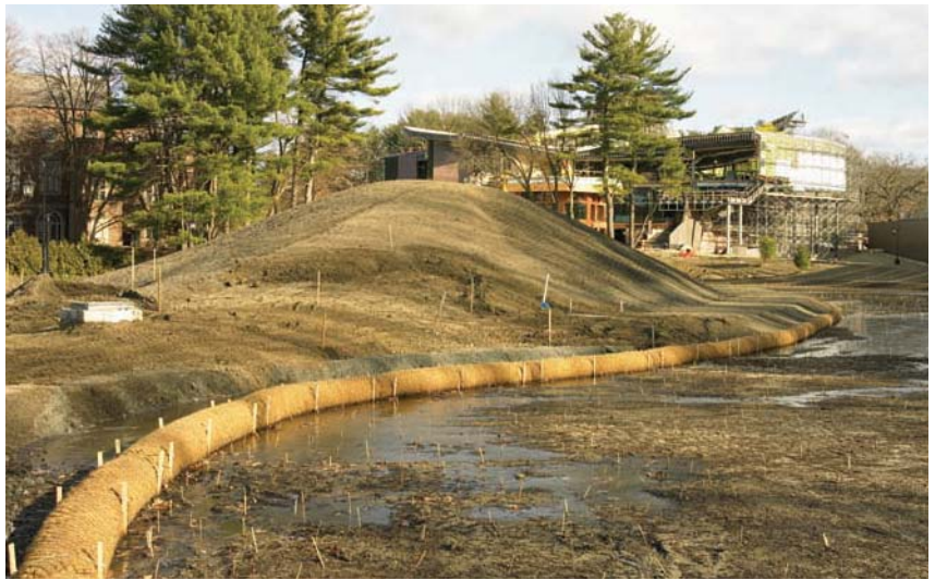
Reinvigoration of Alumnae Valley, Wellesley College, Wellesley, Massachusetts, 2001–05 (work in progress). Designed wetland will filter particulates, absorb nutrients, and lower temperature before releasing the treated water into Lake Waban.
