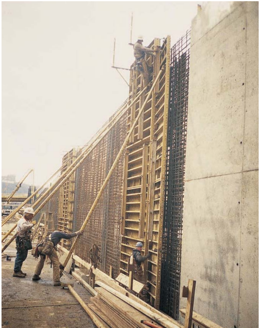
ABOVE and OPPOSITE: Steel fabrication built to withstand ice floes reinforces the concrete access ramps
