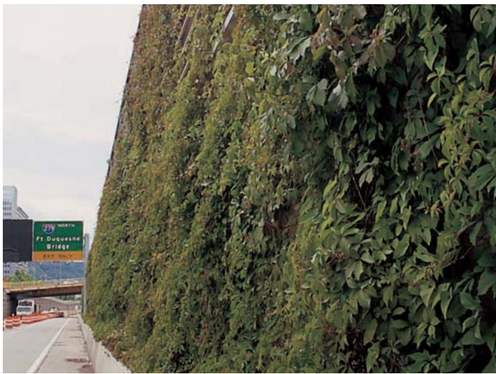
Virginia creeper engulfs the highway side of the ramp structure.
