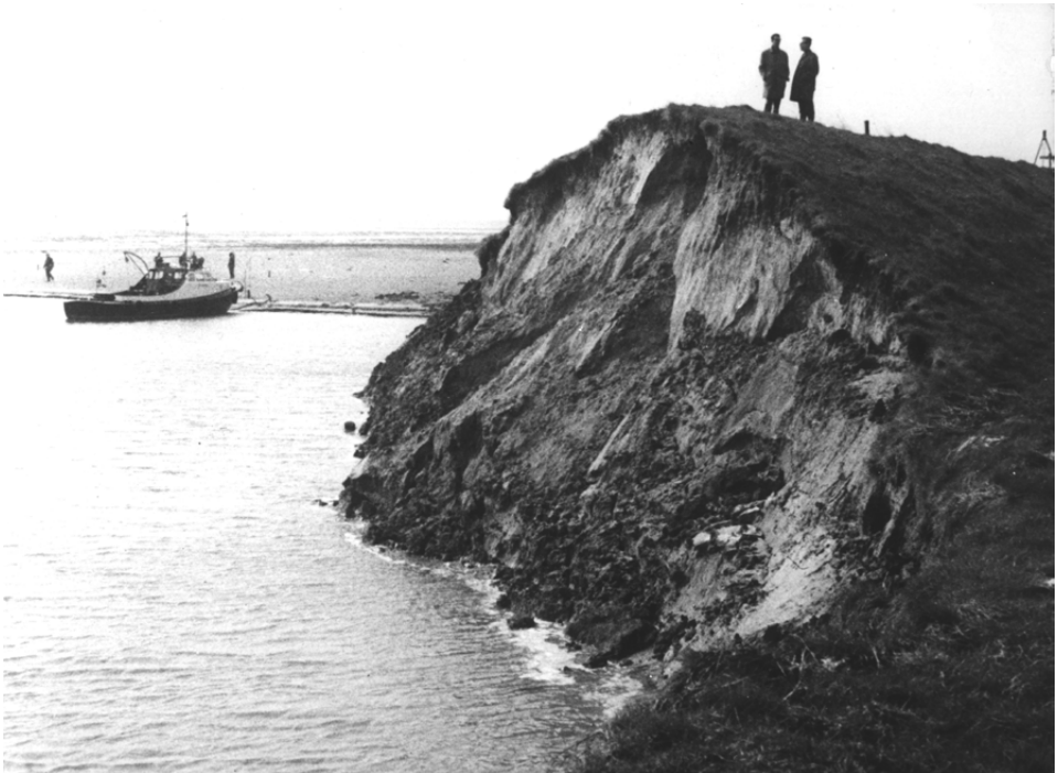
Slide of dike slope (Zeeland), courtesy GeoDelft
