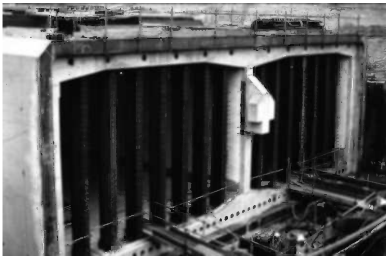
Figure 14.15 Nose and chin end support. (Photo courtesy of Kent County Council/BAM Nuttall/Carillion/Philip Lane.)
