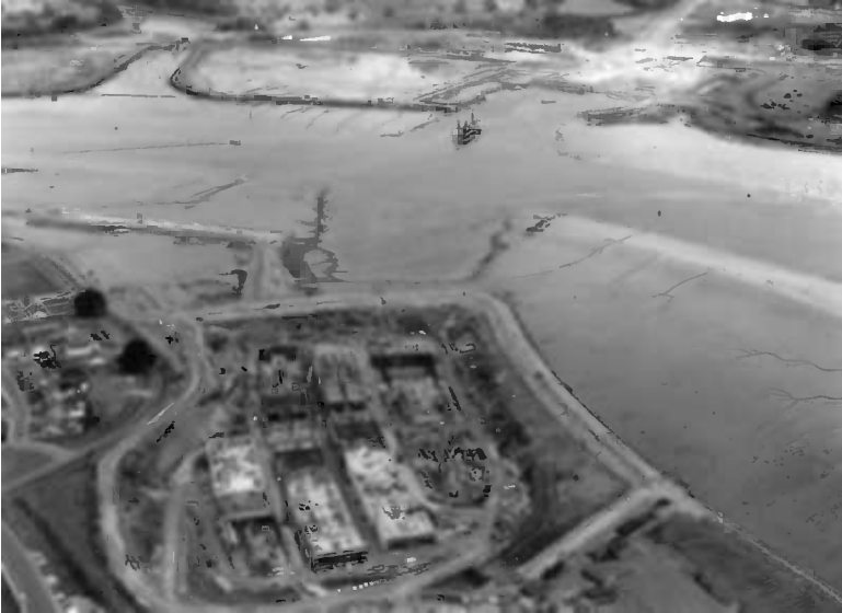
Figure 5.1 Construction of Jack Lynch Tunnel. (Photo courtesy of Cork City Council/ Robert Bateman.)
