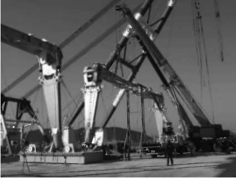
Figure 14.27 External positioning system (EPS) used on the Busan Tunnel. (Photo courtesy of Strukton Mergor.)
