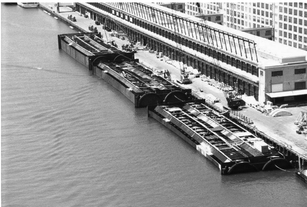
Figure 2.7 Ted Williams steel tunnel elements at concreting jetty. (Photo courtesy of W. Grantz.)
