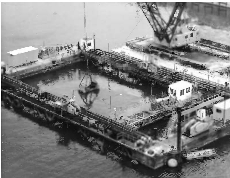
Figure 12.4 Screeding frame used on the Fort McHenry Tunnel. (Photo courtesy of W. Grantz.)
