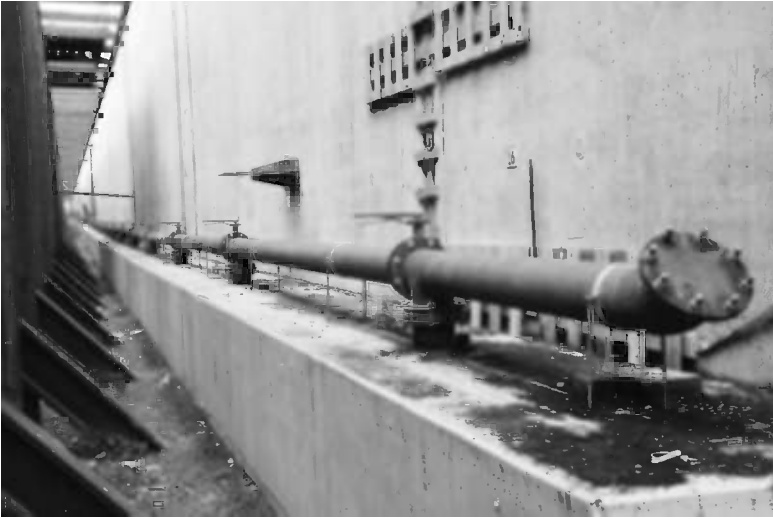
Figure 12.3 Pipework for sand flow. (Courtesy of NRA/DirectRoute.)
