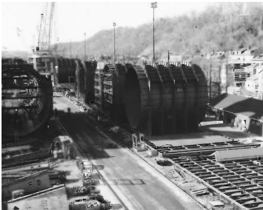
Figure 14.4 Fabrication of the Fort McHenry Tunnel elements. (Photo courtesy of W. Grantz.)
