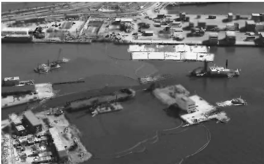
Figure 5.2 Silt curtains in use during dredging for the Bjørvika Tunnel. (Photo courtesy of Statens Vegvesen.)
