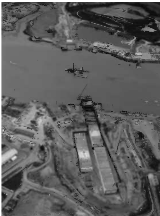
Figure 4.8 Constructing tunnel elements in the approaches. (Courtesy of Kent County Council/BAM Nuttall/Carillion/Philip Lane.)
