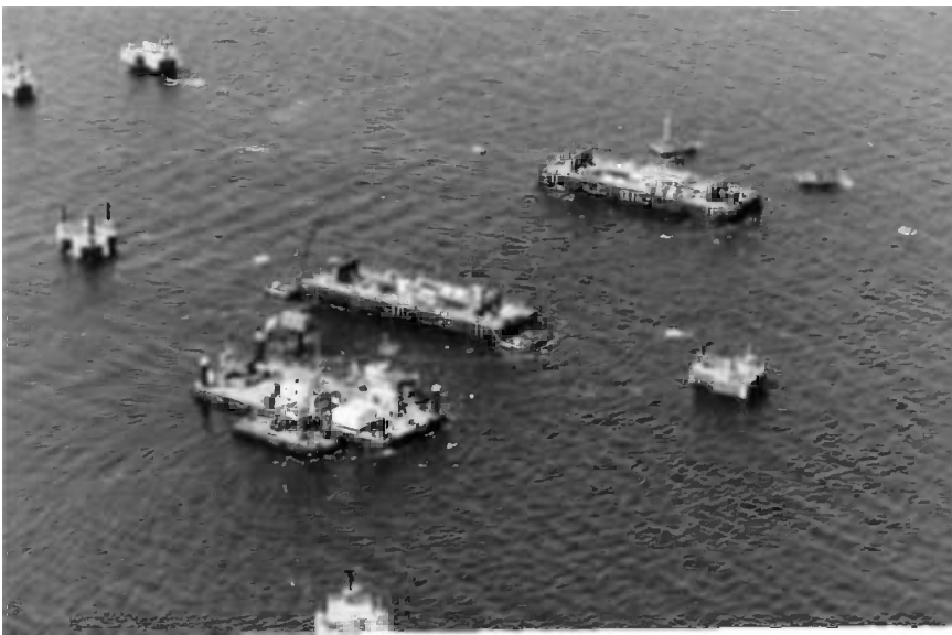
Figure 14.26 Anchor platforms used for immersing tunnel elements on the Øresund project. (Photo courtesy of Øresundsbron.)
