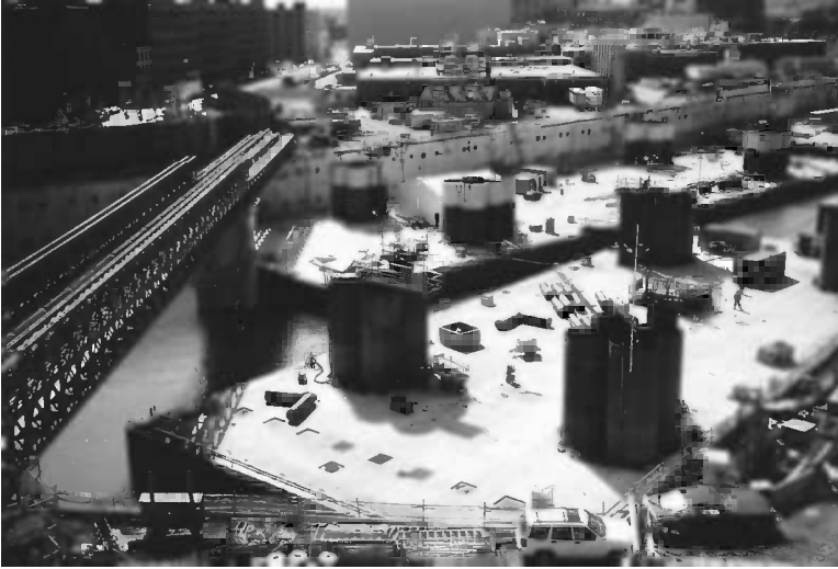
Figure 14.20 Immersion cylinders used for the Fort Point Channel Tunnel. (Photo courtesy of D. Wrock.)
