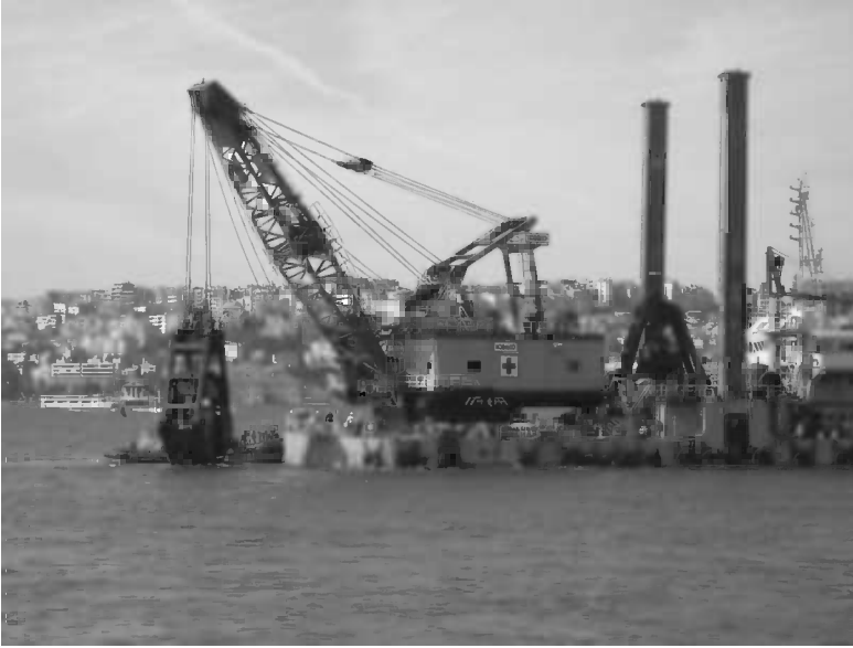
Figure 13.1 Clamshell dredging on the Marmaray Tunnel (27 m 3 grab). (Photo courtesy of W. Grantz.)
