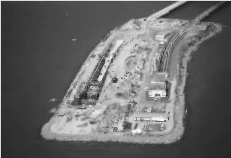
Figure 13.10 Transition island at the Hampton Roads Tunnel. (Photo courtesy of W. Grantz.)
