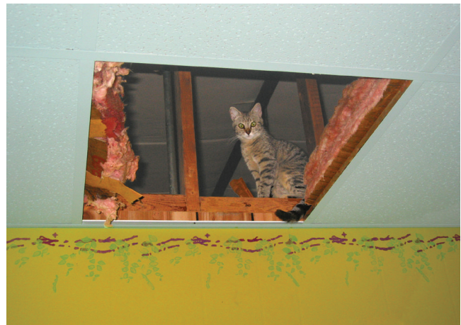
Figure 76-8. Particular attention to the provision of solid surface ceilings in housing enclosures is essential to prevent the escape of crafty cats into the rafters. Once in the ceiling, cats may be difficult to recover and may become injured and/or cause substantial damage to facilities.
