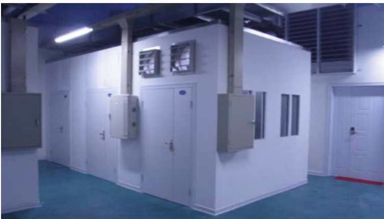
Fig. 30.2 Data center with container-type modular design of Hanyun Company
