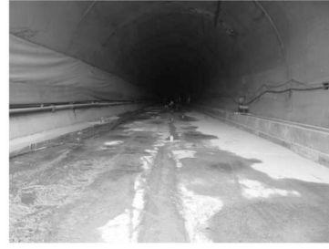
Figure 3. Longitudinal cracks on the inverted arch at the entrance of the tunnel.
