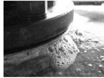
A. Leakage of safe valve nozzle
