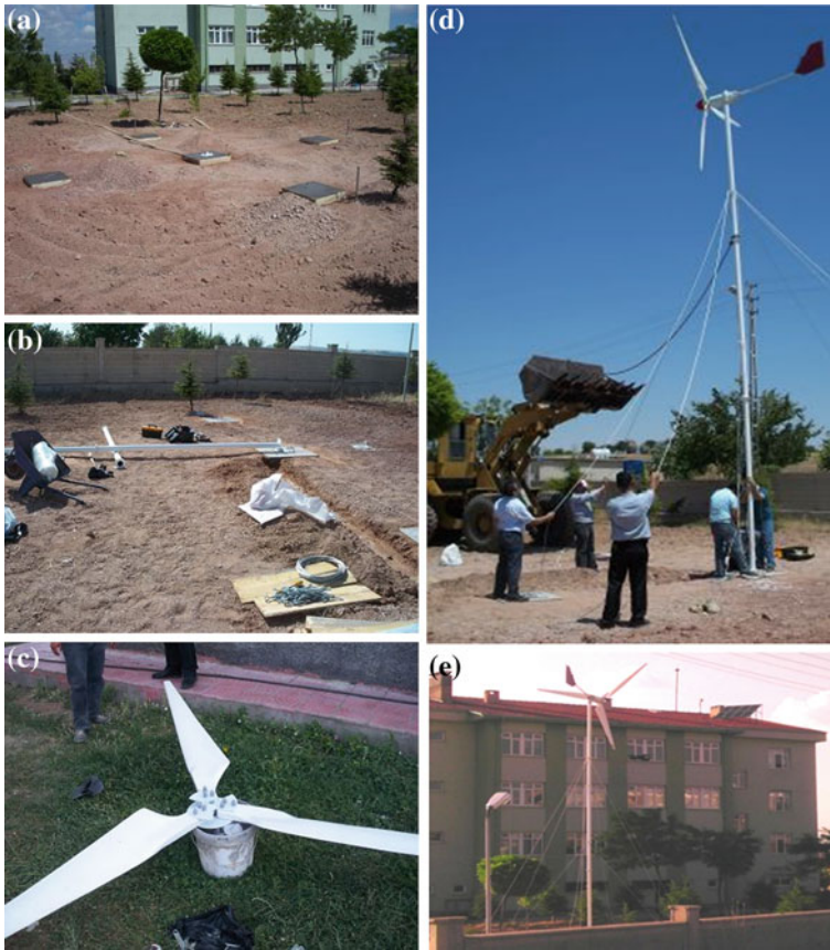
Fig. 2 Installation of hybrid renewable plant, a base concrete of WT, b tower connection, c assembling of blades, d building-up the turbine, e completed installation of plant
