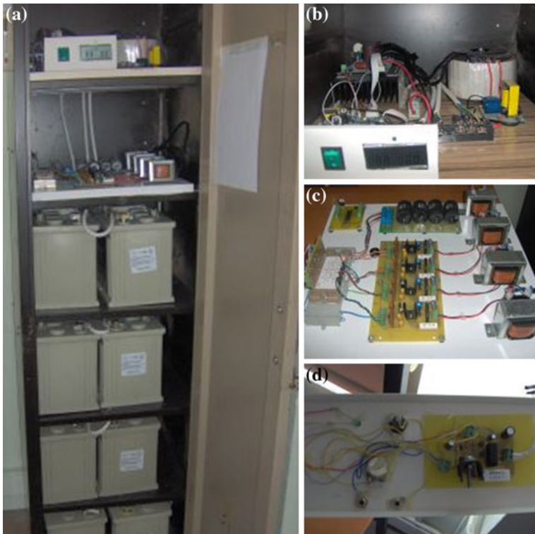
Fig. 4 Energy control system and components, a the cabinet of batteries and converters, b converters, c inverter and controller, d SMPS assembly located in training desks
