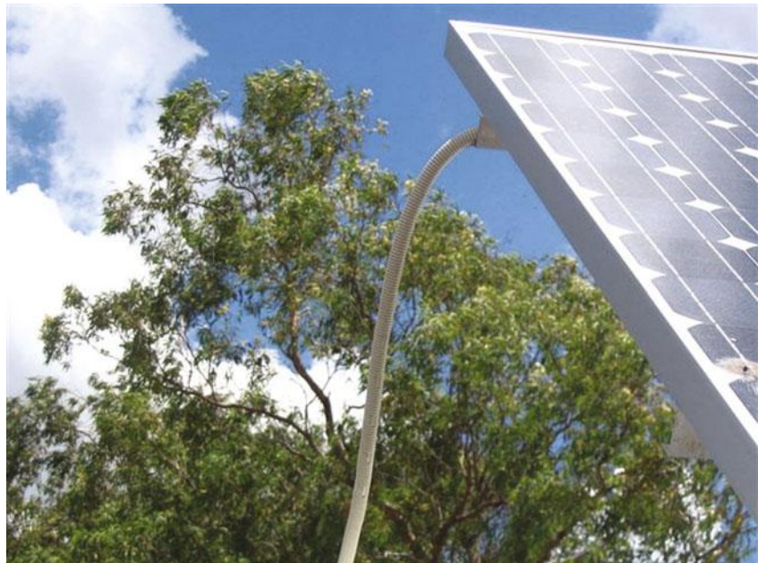
Figure 10.5 Example of an array cable left loose and unsupported
