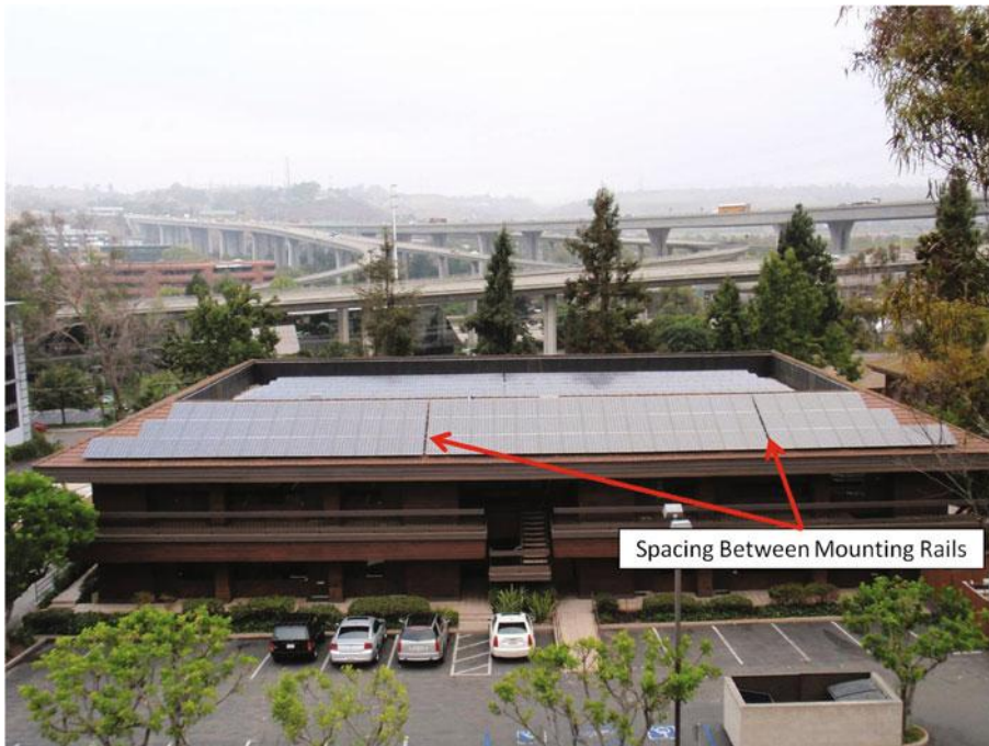
Figure 14.14 The mounting rails have been installed with periodic gaps between adjacent rails allowing the metal rails to thermally expand without damaging the mounting structure
