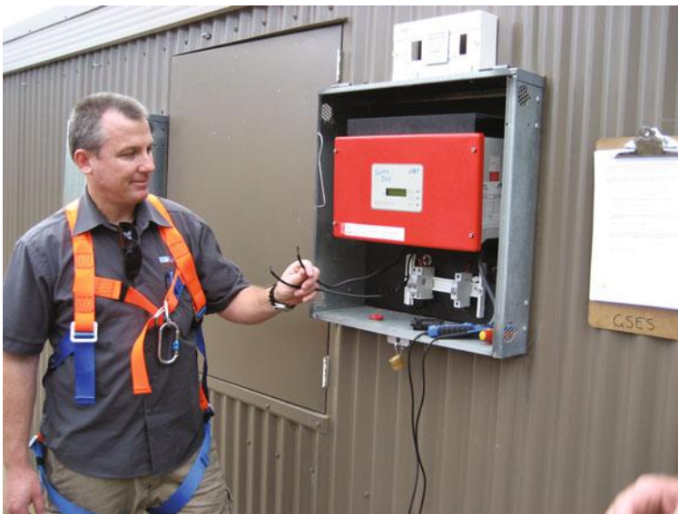
Figure 5.3 An electrician tests a grid-interactive inverter
