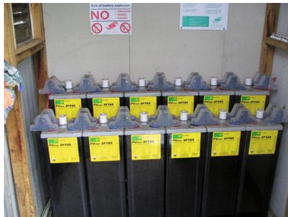
Figure 1.6 Batteries in a stand-alone solar electric system
