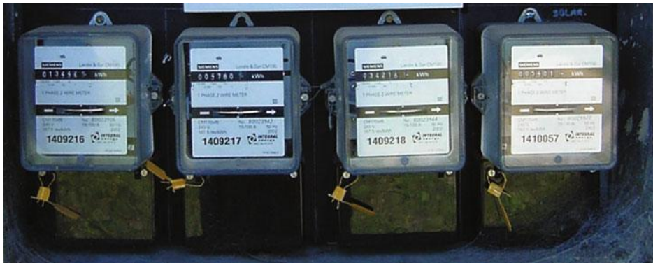
Figure 5.42 Multiple meters are common, often for off and on peak demand metering and large appliances like ducted air-conditioning
