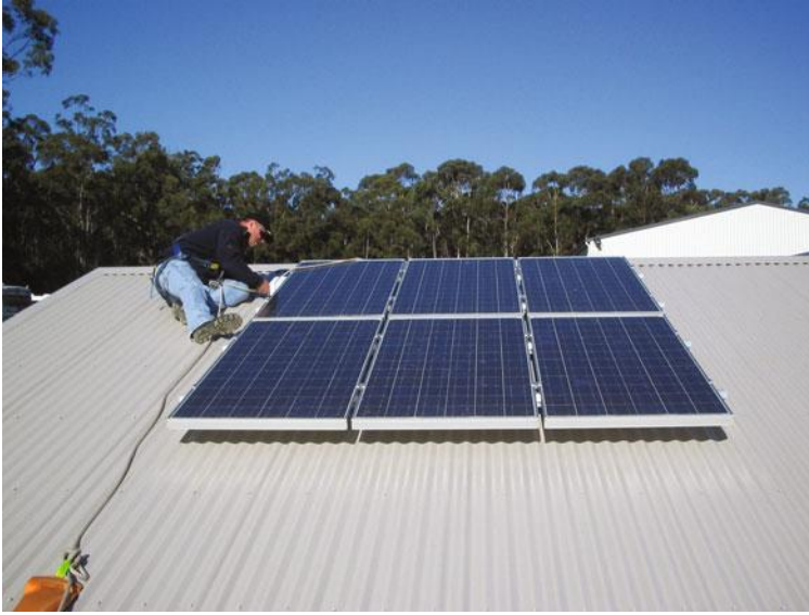
Figure 10.6 An electrician installs a small white PV combiner box next to the array
