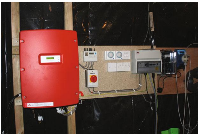
Figure 14.31 The inverter is located in the pool shed behind the PV array; the inverter is connected to a generation meter which measures the PV array's power output, then to a lockable double pole isolating switch and then directly into one of the miniature circuit breakers located on a distribution board in the shed
