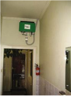
Figure 7.19 Badly located inverter; the system owners will have great difficulty accessing information from this inverter
