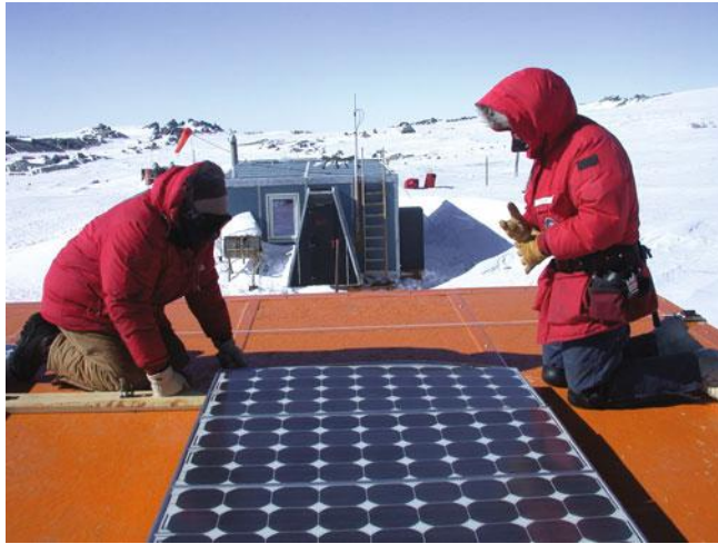
Figure 4.20 PV modules perform well in cold and sunny areas. They are often used as a power source in Antarctica during the summer. However, because there is so little light in winter, diesel generators are typically used as back-up
