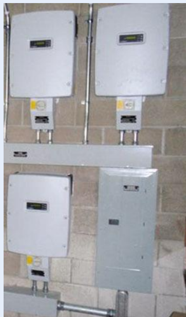
Figure 5.30 These inverters are designed for the US market and incorporate a large UEDS beneath the inverter
