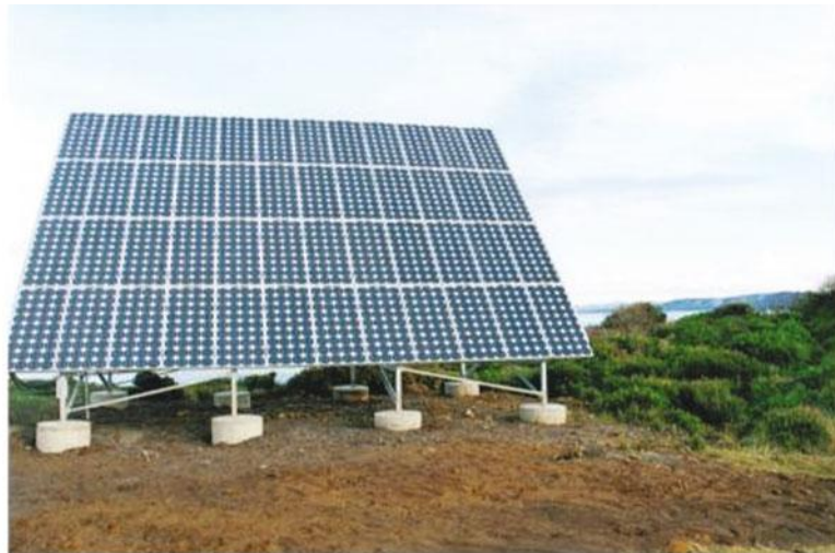
Figure 6.13 Large ground-rack mounted installation
