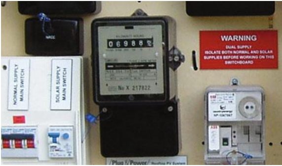
Figure 5.34 Rotating barrel style meter, here shown accompanied by signage for a PV installation
