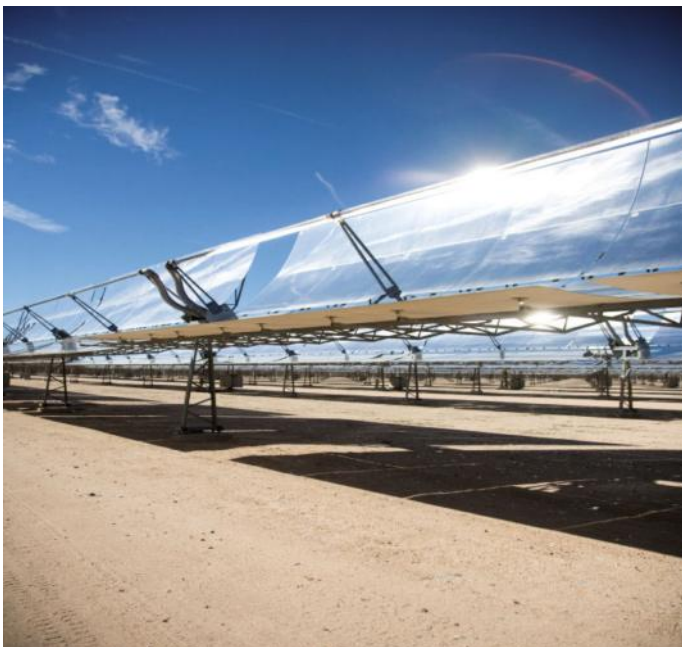
Figure 1.14 A CSP installation in the Nevada Desert. Parabolic mirrors concentrate sunlight to heat the water running through the thin tubes in front of the mirrors
