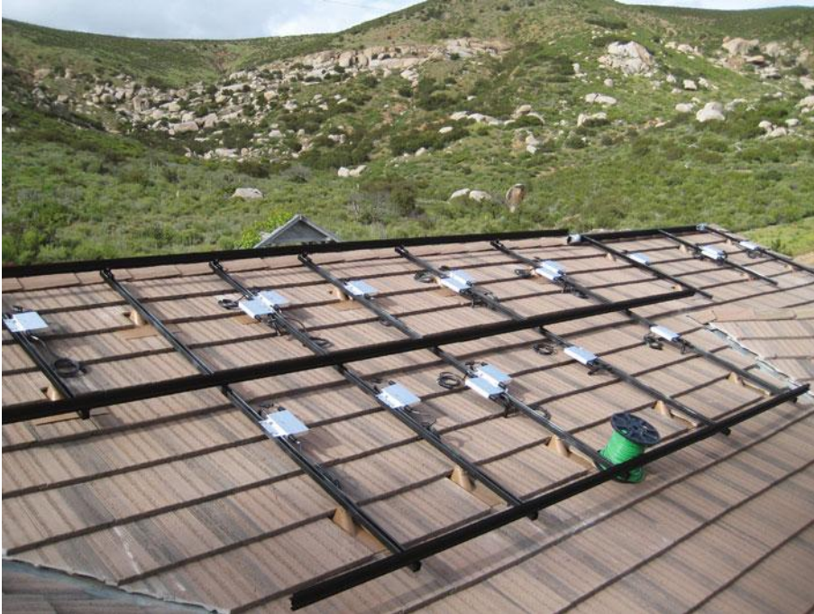
Figure 14.21 In order to overcome the challenges presented by this residential roof, the system designer decided to forgo the traditional central inverter system architecture and install micro-inverters on each solar module. The micro-inverters are mounted on to the rails directly beneath the modules and convert the DC current from the PV module into AC current. Each individual micro-inverter has its own MPP tracking system so that the performance of each PV module is completely independent of its neighbours. The AC outputs are connected in parallel and then feed directly into the residential main service panel
