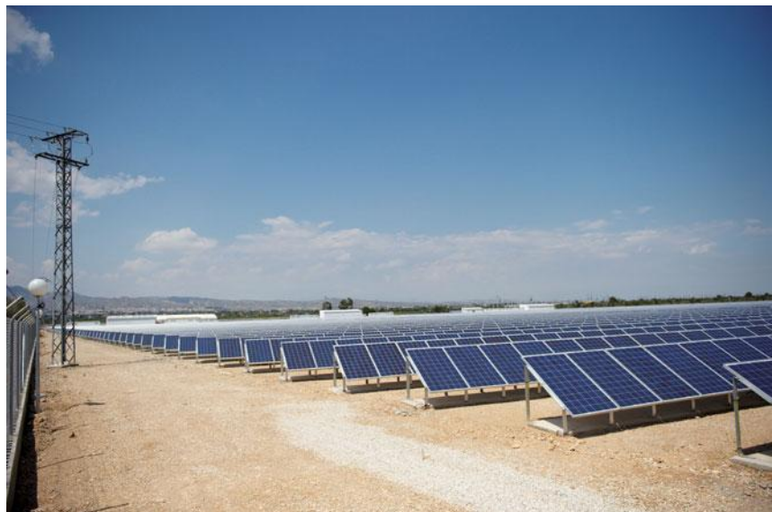
Figure 1.9 Alicante, Spain, 5.6MW p central PV system
