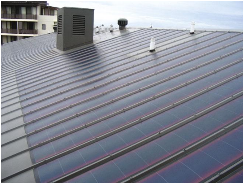
Figure 6.12 Amorphous laminates installed on metal roofing in Australia
