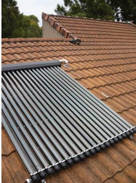
Figure 1.13 A solar hot water system with an evacuated tube collector
