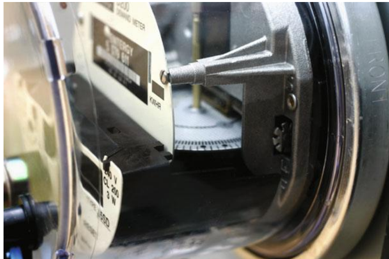
Figure 5.36 The single rotating disc in the centre of this net meter is clearly visible: when electricity is consumed (by loads within the building) it rotates forwards and when electricity is produced (by the PV system) it rotates backwards
