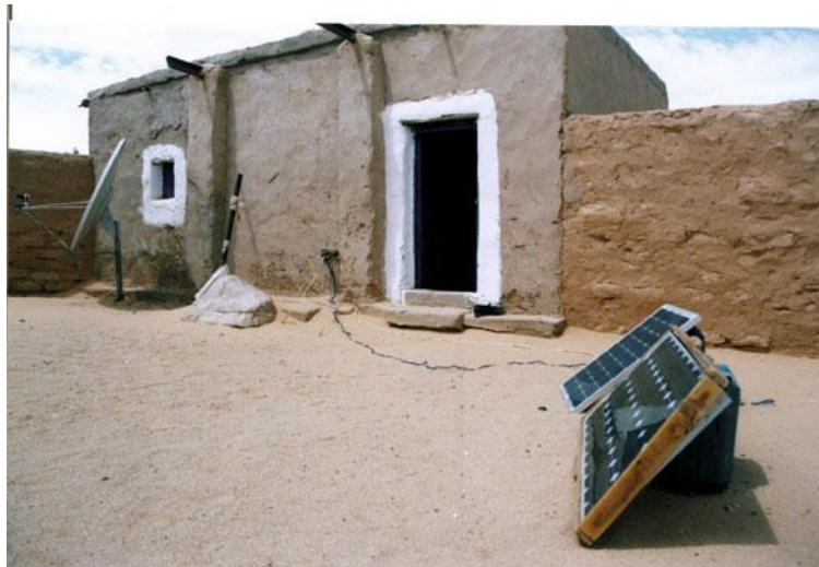
Figure 1.5 Small off-grid solar electric systems are often the most convenient and cost-effective option for those living in rural areas of the developing world such as the West Sahara, where this system is located
