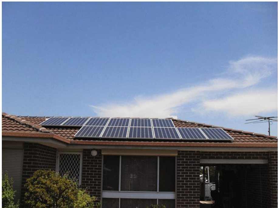
Figure 14.18 The PV array blends in with the profile of the roof and is aesthetically pleasing while allowing some cooling air flow beneath the modules
