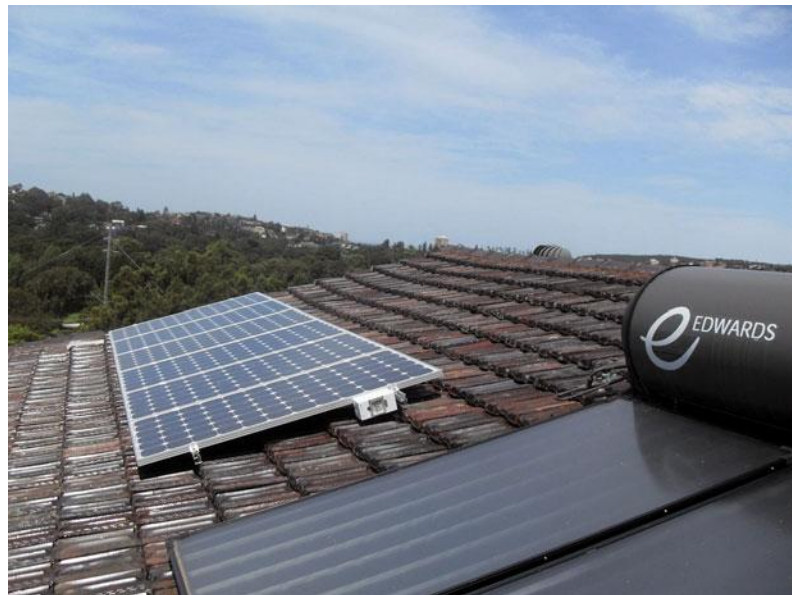
Figure 1.12 This system includes a solar electric system (back) and flat plate solar hot water system with a storage tank (front)
