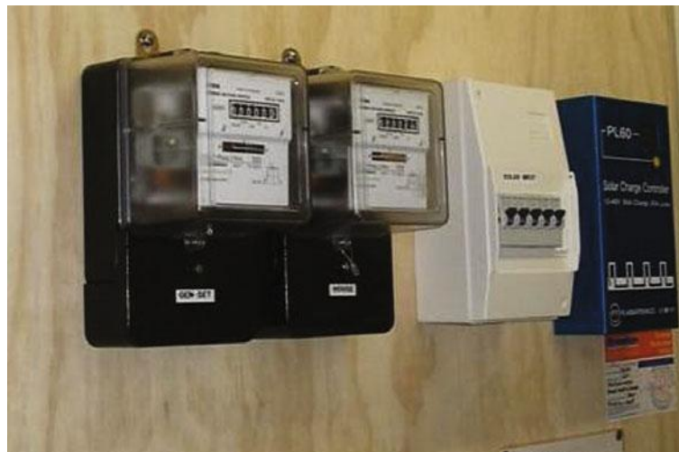
Figure 5.40 Two metering devices, one measuring the power generated and one measuring the power used
