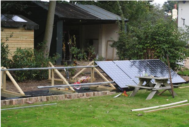
Figure 14.30 The PV array is ground-mounted in the owner's garden
