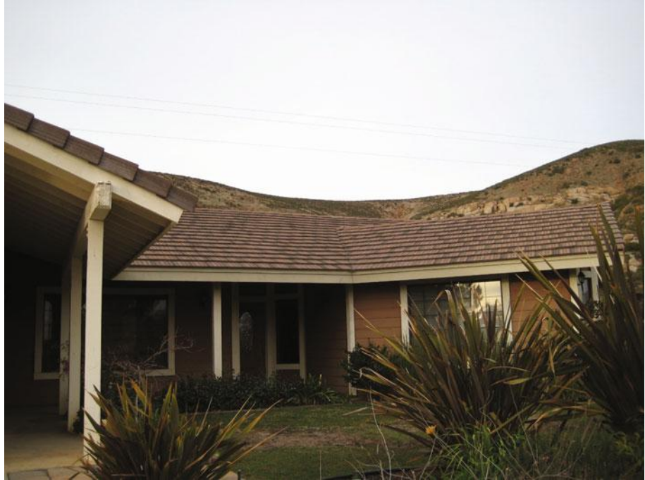
Figure 14.20 This flat tile residential rooftop presented some common design challenges for a typical PV system using a centralized inverter; there are several different roof orientations with suitable solar access (south, west and east). In addition there is not enough available space on each roof face to mount a complete series string, meaning that modules within the same series string would have to be mounted facing different orientations. Modules facing different directions would receive different amounts of solar radiation (see Chapters 7 and 9) and hence have different power outputs. As discussed in Chapter 4, it is not desirable to connect PV modules with very different outputs in series and the total power output of the system would suffer
