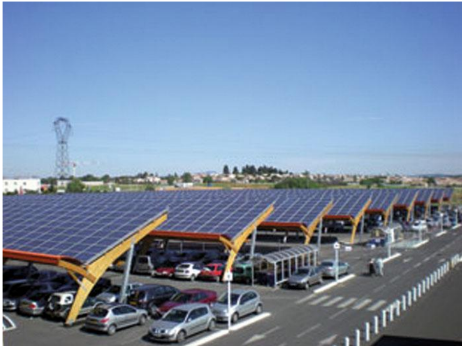
Figure 6.10 BIPV awnings developed by Sunvie and integrated into a car park; this 1.15MWp installation is located in St Aunès, France
