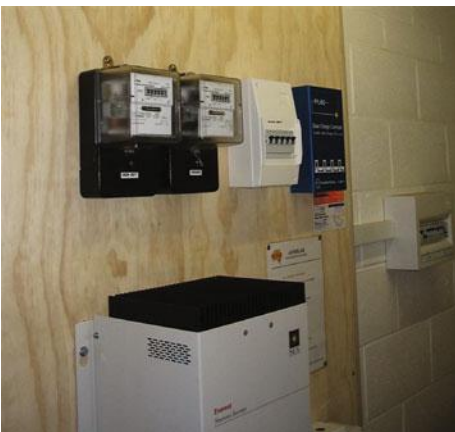
Figure 7.20 Well-located BoS components are protected, well-ventilated and neatly installed
