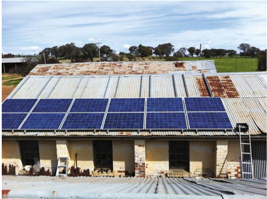
Figure 14.29 In this photograph the metal rails that make up the mounting structure are clearly visible
