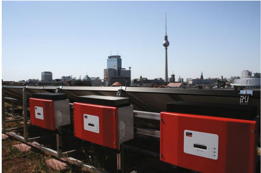
Figure 14.1 Three inverters are used, one for each array
