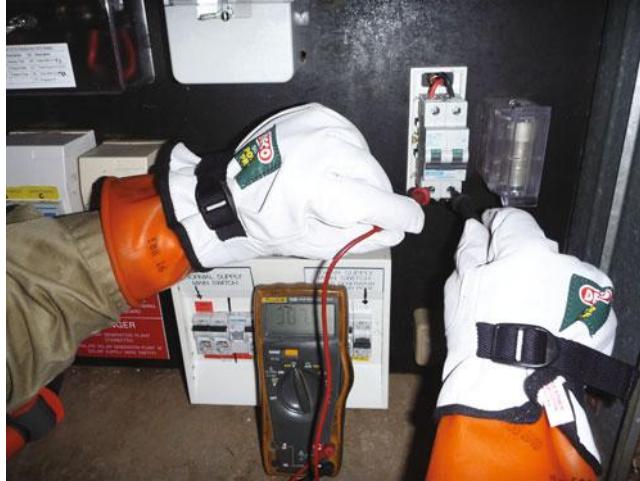
Figure 11.1 An electrician checks the open-circuit voltage and polarity of an array cable entering the inverter
