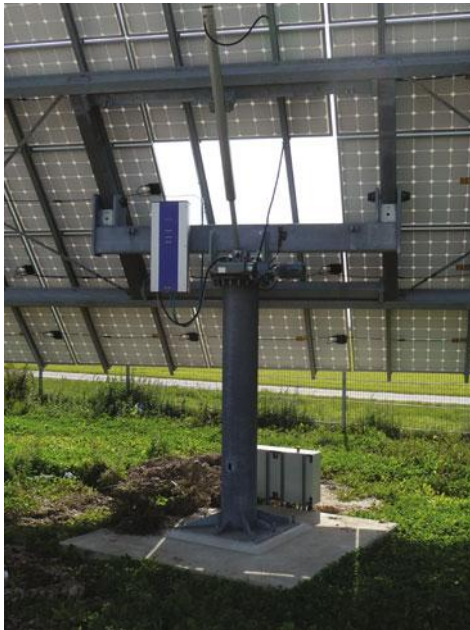
Figure 6.17 The tracking hardware can be seen on the back of this array
