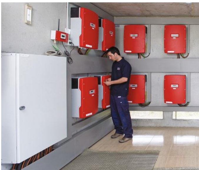
Figure 5.15 For very large installations a whole room of central inverters may be required. These are SMA Sunny Mini Central inverters
