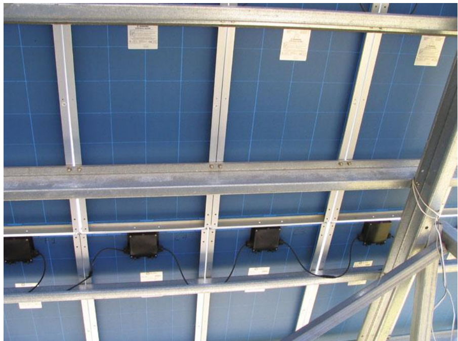
Figure 5.24 Module junction boxes on the back of modules in a PV array
