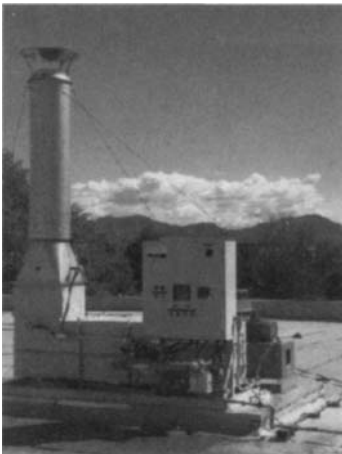
Figure 8-15 An operating catalytic oxidizer (courtesy of Stealth Industries, Inc.).
