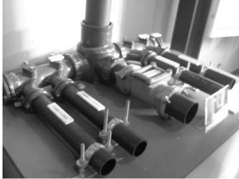
Fig. 1.38 Sewage header of KSI
