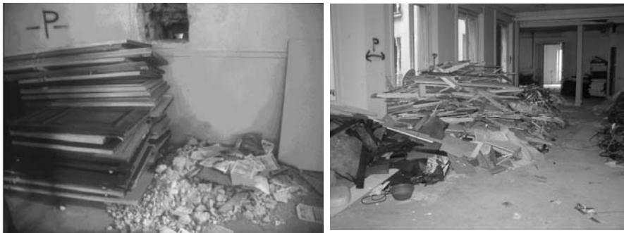
Fig. 6.21 A "P" on the wall indicates lead paint
