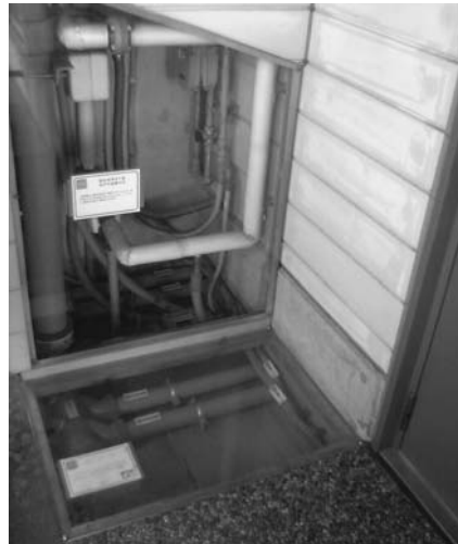
Fig. 1.37 Outside sewage system of KSI
