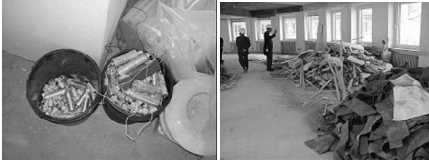
Fig. 6.18 Fluorescent lamps, paper and rubber are also separated
