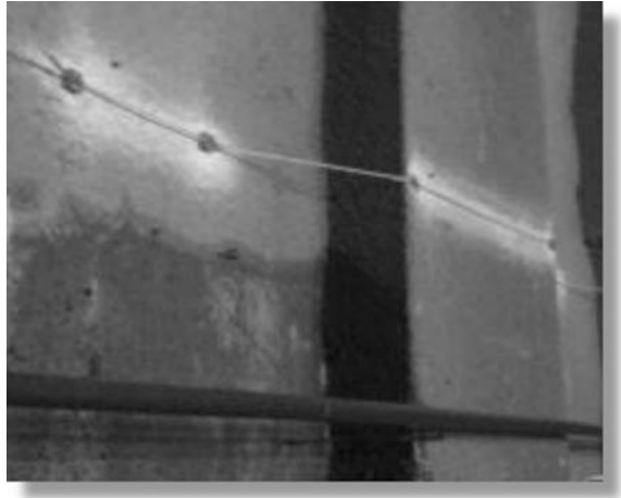
Fig. 5 Distributed sensing cable installed on tunnel wall [SMARTEC, Switzerland]
