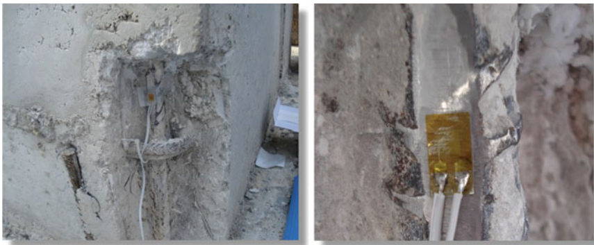
Fig. 8 Gauge-type sensors installed on civil structure pier. Work executed in the framework of the EC co-funded project “MEMSCON” [FP7-NMP]
