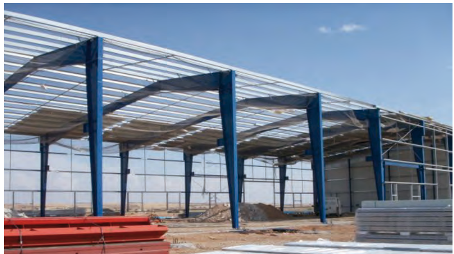
Figure 5.9 Single portal frames with tapered columns and rafters under construction in Spain
