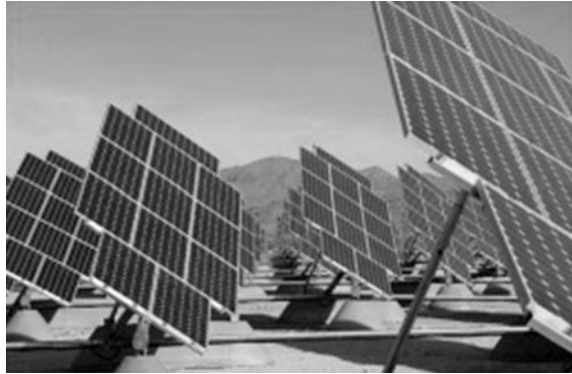
Fig. 7.9 A high capacity solar farm tracking sun in two axes
