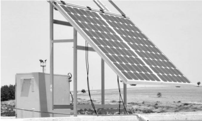
Fig. 7.13 Picture of the fixed photovoltaic panel system
