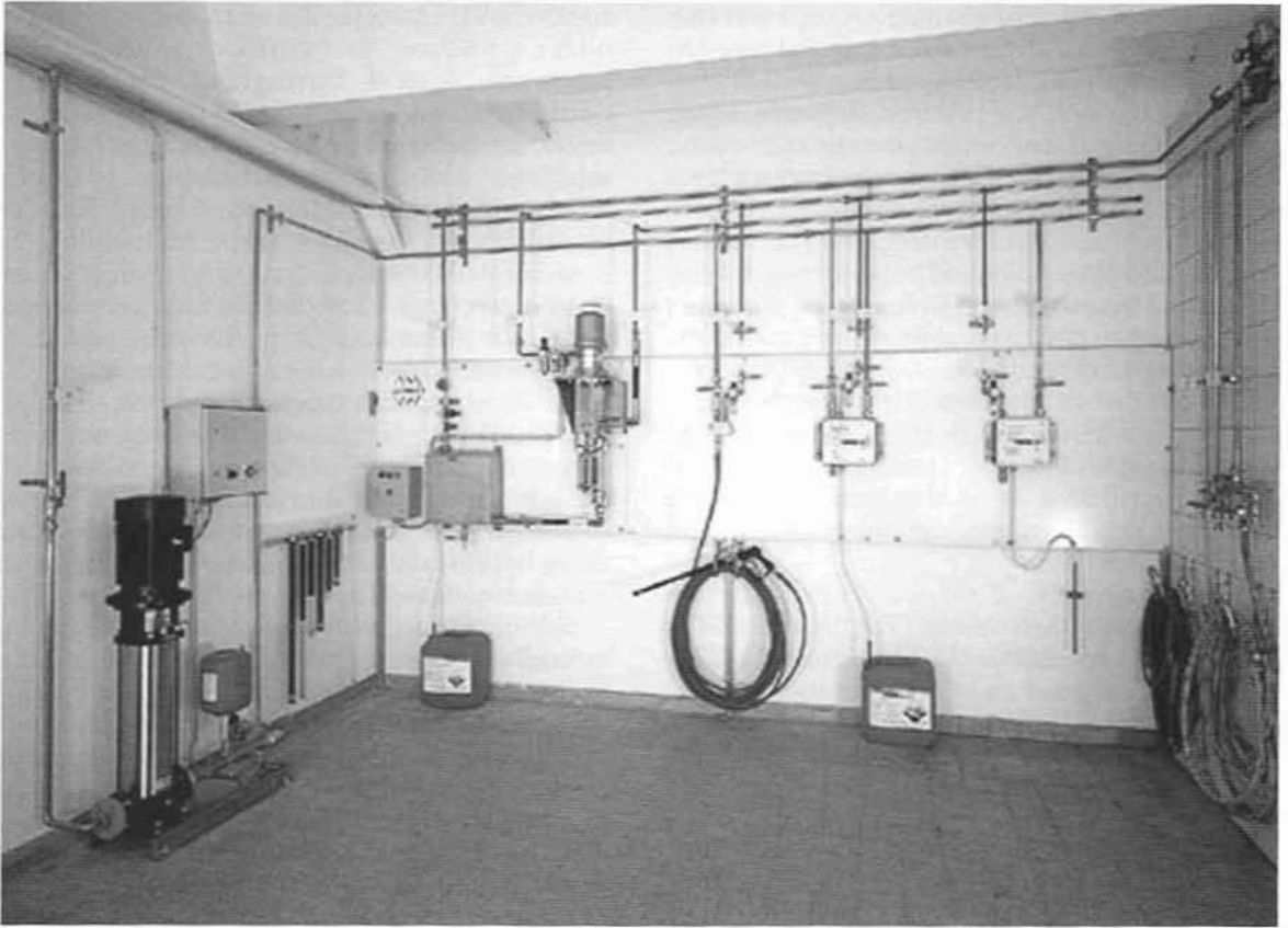
Fig 6.1 Demonstration room showing installations of central and satellite foam and rinse stations.
