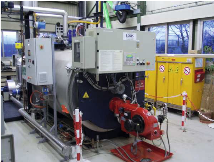
Fig. 2. Boiler side view
