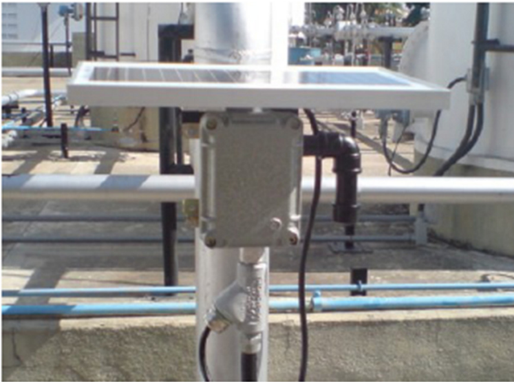
Fig. 2 RFD sensor node Setup with solar panel
