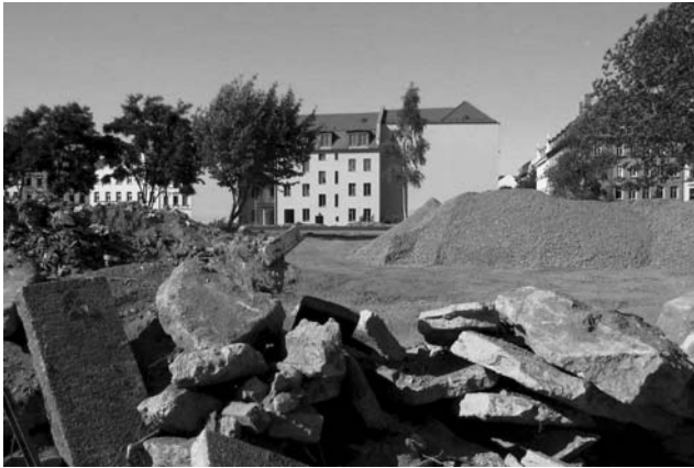
Figure 28.2 Large-scale demolition of densely built-up housing structures in inner parts of the Wilhelminian-time city (built between 1870 and 1910): new open spaces for experimental design of recreational green infrastructure (Source: D. Haase).
