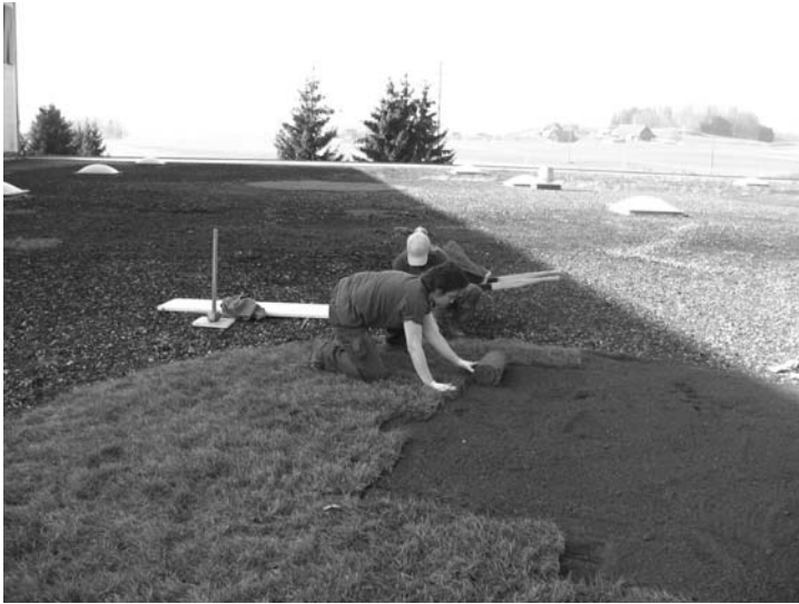
Figure 18.2 Installation of circular patches of turf (2.5 cm deep) on the top of 4 cm of ‘ricoter’, a Swiss compost recycling product developed for establishing rooftop vegetation. The original ‘substrate’ on this roof was medium-sized gravel (2007, N. Baumann).
