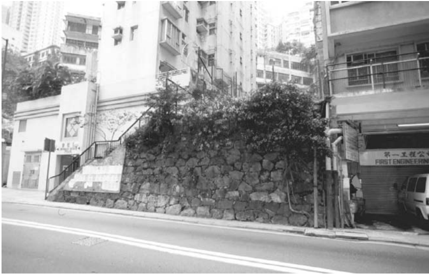
Figure 17.3 Old stone walls are considered by developers as obstacles to redevelopment, which often results in drastic modification or outright demolition, posing the most serious threat to wall ecology; the original line of old stones walls along this road has been largely removed in the course of urban redevelopment, leaving this small remnant segment. (Bonham Road, Hong Kong, July 2000, C.Y. Jim).
