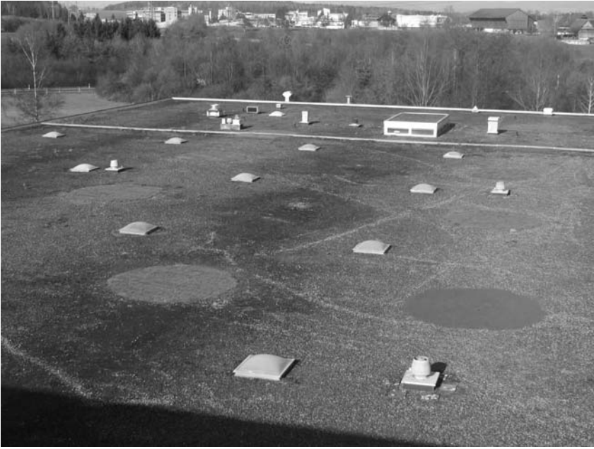
Figure 18.4 View of the roof in Rotkreuz just after the completion of the vegetation improvement works (2007, N. Baumann).
