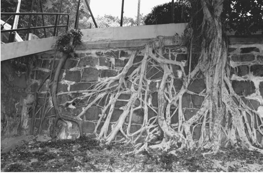
Figure 17.2 Some wall trees have been hacked or removed completely in the course of overzealous maintenance that is often fuelled by unsubstantiated concerns about wall stability; note that the Banyan strangler roots began their life as soft and flexible aerial roots, and subsequently became lignified and fused if they managed to acquire sufficient water and nutrients mainly from the soil lying behind the wall; poor workmanship in wall maintenance, as illustrated by crude pointing of the joints by modern Portland cement, could sanitize the wall habitat and prevent future vegetation growth (Forbes Street Playground, Hong Kong, June 2007, C.Y. Jim).
