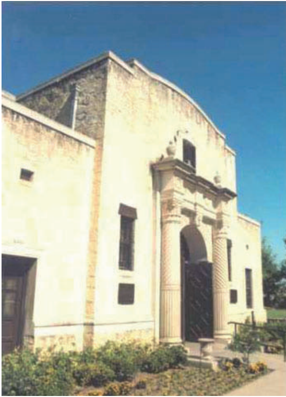
Fig. 22. Microbial adhesion and consequent deterioration only occurred at the top (dark) part of the building. The lower, protected portion was free of bacteria and deterioration.
