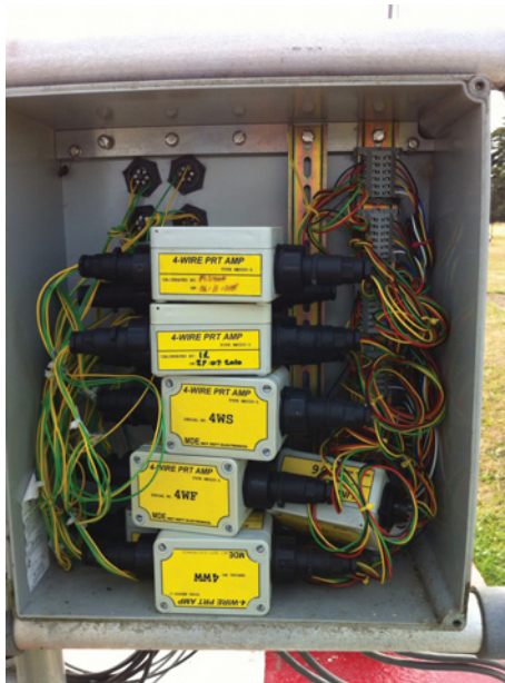
Figure 3.27 A set of platinum resistance thermometer signal conditioning amplifiers used for soil temperature measurements. Each channel's signal conditioning electronics is mounted within an individual weatherproof box, with weatherproof connectors at each end (sensor connections at one end, power supply and signal output at the other). The set of devices is mounted within an outer weatherproof cabinet.
