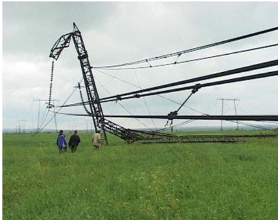
Fig. 6.6 OTL-220 kV support deterioration under the influence of a hurricane
