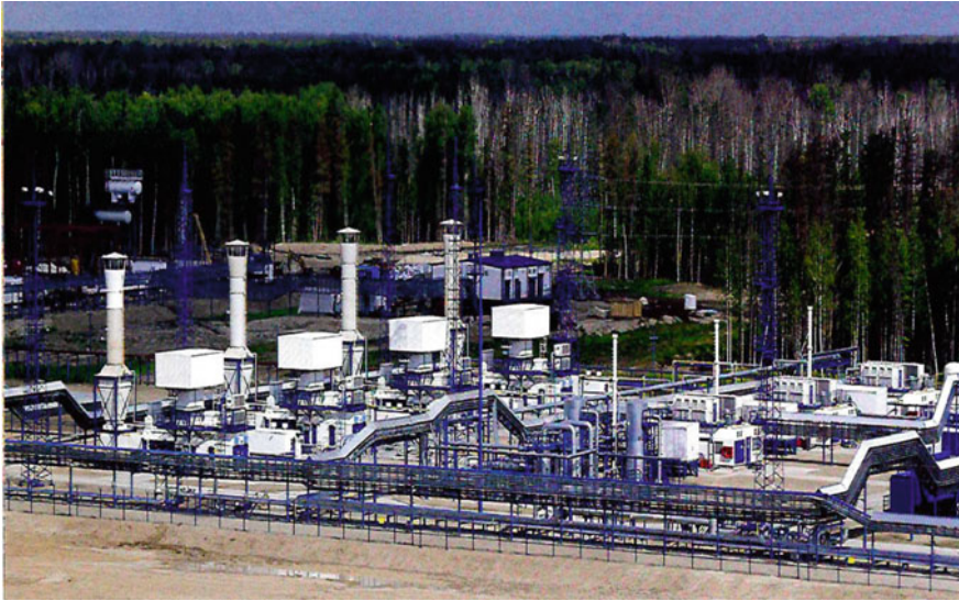
Fig. 4.7 Gas turbine power plant using associated gas (capacity of 24 MW, owned by “Gazpromneft-Vostok”, Russia)
