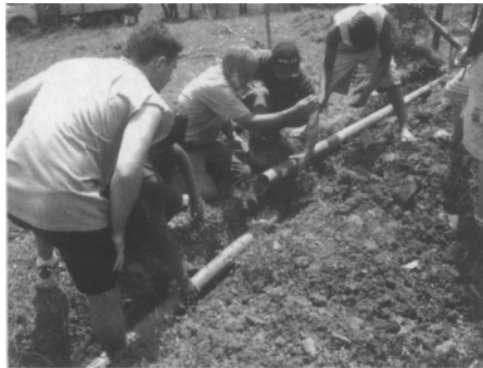
Villanova University engineering students and faculty work on a pipeline of a water network in Waslala, Nicaragua
