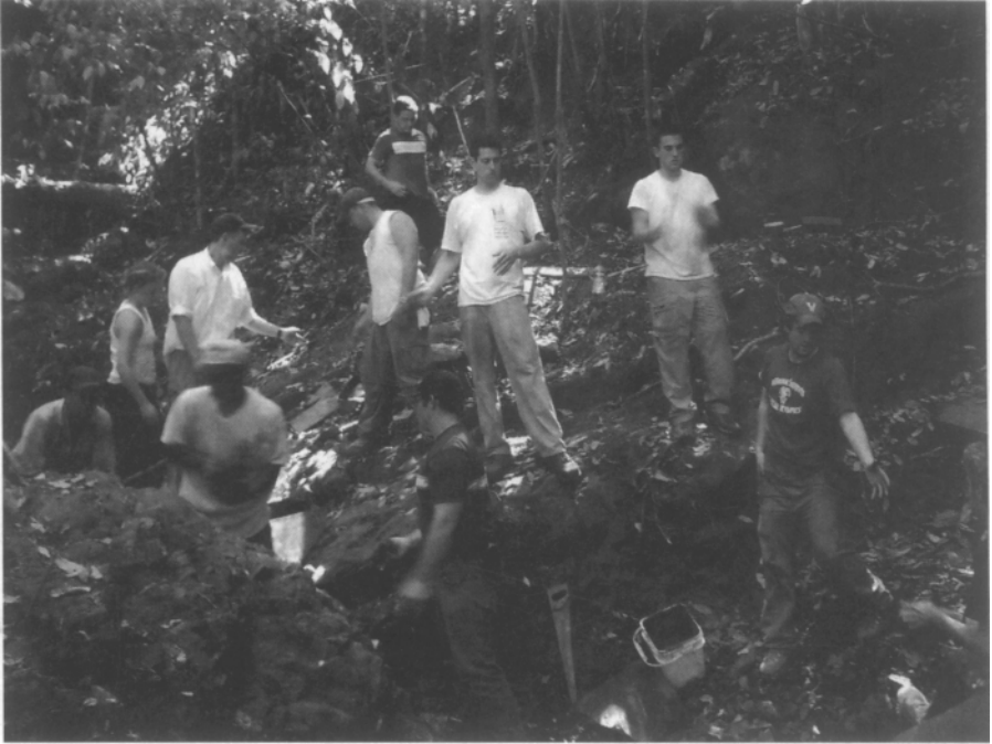
Students and faculty from Villanova University work with technicians in Waslala, Nicaragua preparing to construct a reservoir.
