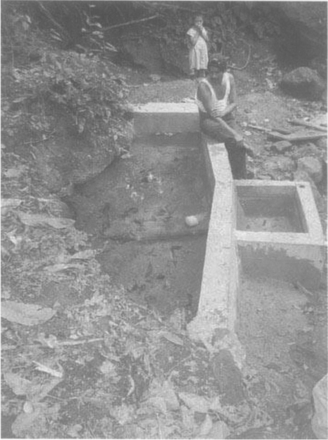
Figure 13.4 A spring box under construction in central Nicaragua. A cast-in-place concrete cap was installed after this photo was taken (see Fig. 1.2).
