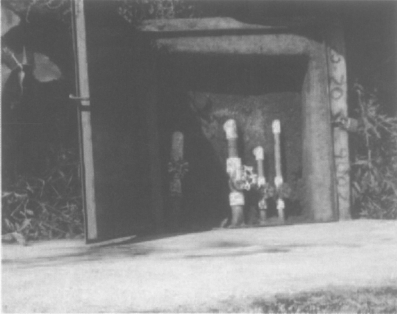
Figure 15.17 Protected valve box.
