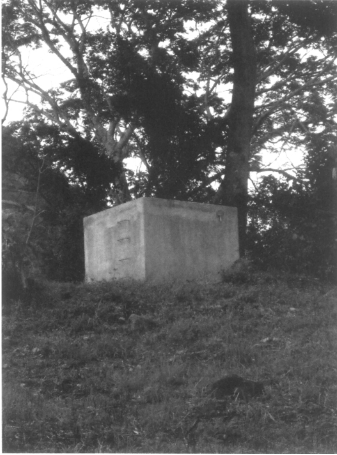
Figure 1.6 A concrete storage tank. The capacity is \sim 14 \text{ m}^3 .
