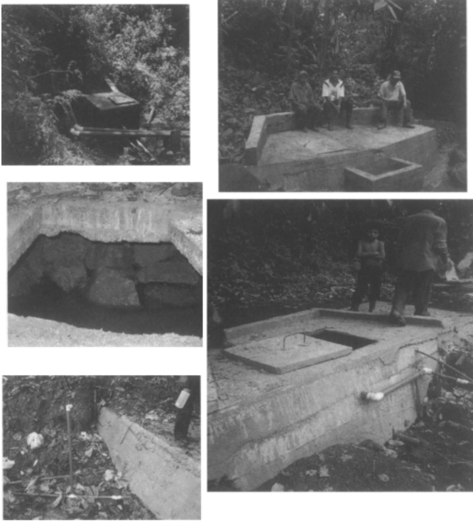
Figure 1.2 Photos of reservoirs. All are constructed of poured concrete. Clockwise from upper left: a covered reservoir separated from uncovered section by a screen filter (PVC pipe in foreground awaits installation), a totally covered reservoir with a concrete valve box in front, a totally covered reservoir with cover partially removed for access to clean filter inside, a dam to hold back water before construction of the reservoir (the vertical PVC pipe downstream from the dam is a vacuum breaker; see the discussion in Section 1.3.6), inside view of a totally covered reservoir.
