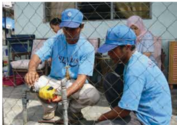
Meter replacement: Ensuring accurate billing through replacement of aging meters in Kuala Lumpur. Photo by Abdul Raof Ahmad, Corporate Communications and Public Affairs Division, SYABAS.
