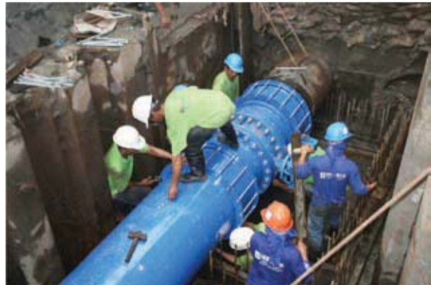
Contractors at work during an interconnection activity in Sta. Mesa, Manila. Photo by Federico Juane.
