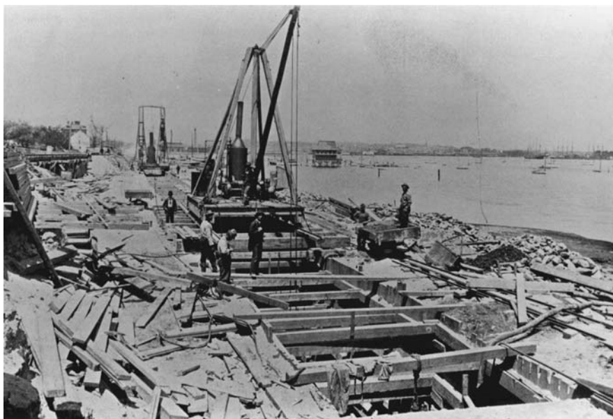
Fig. 5.4 Building sewers along the Providence River. From the Annual Report of the City Engineer for 1894.
