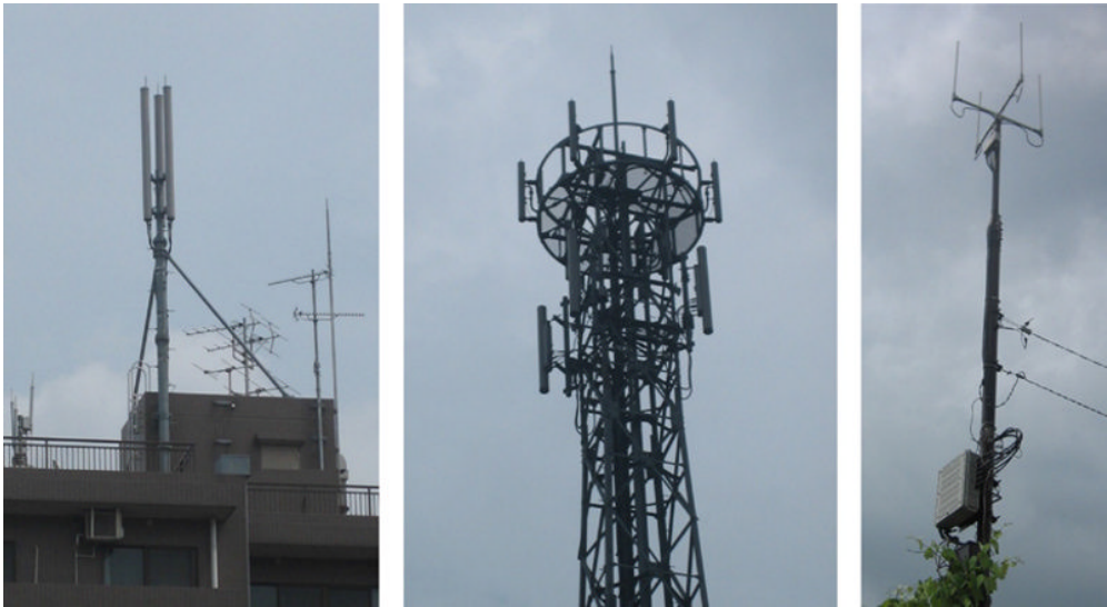
Figure 10.10 Base station antennas
