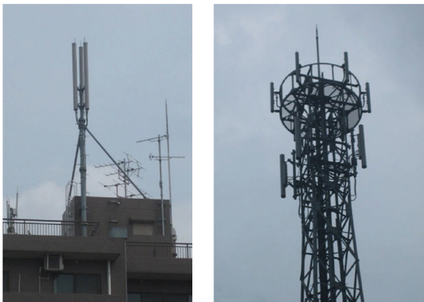
Figure 13.5 Two macrocell base station antennas
