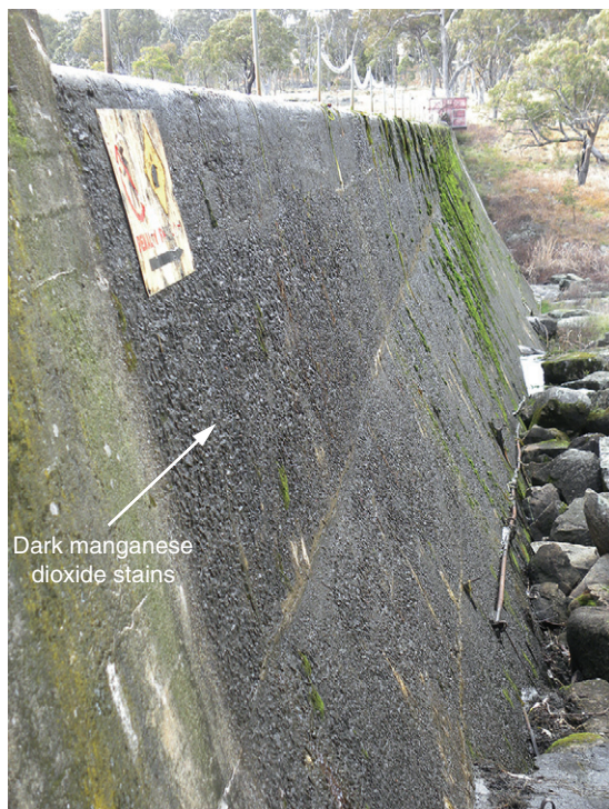
Figure 3.14 The dark stains on the wall of this reservoir arise from oxidation and precipitation of dissolved manganese into insoluble manganese dioxide on contact with oxygen. (Source: Darren Ryder.)
