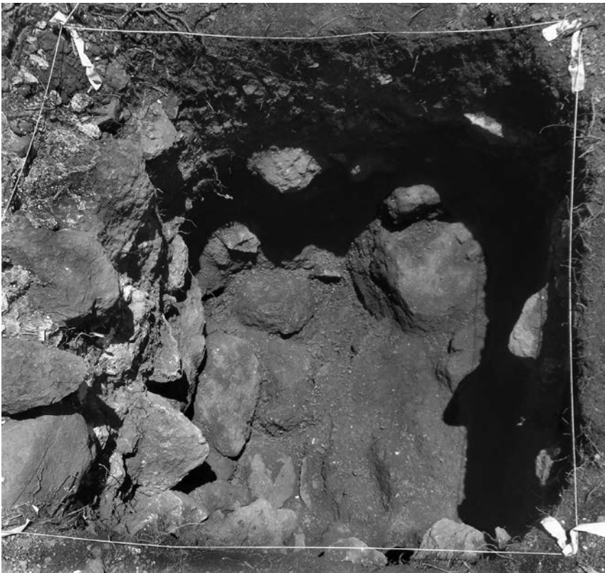
Figure 3.5. Plan view of unit A2 in the downslope side of the main Lettsom house foundations showing (on the left) a highly irregular and unfinished wall face, never meant to be seen.
