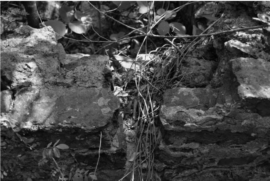
Figure 5.3. Gun loop from a non-Quaker site on Norman Island (Phase II, a room to the immediate west of the original building [see figure 2.15]) viewed from outside the structure, obliquely from above, after the wall in which it was set was partially ruined.
