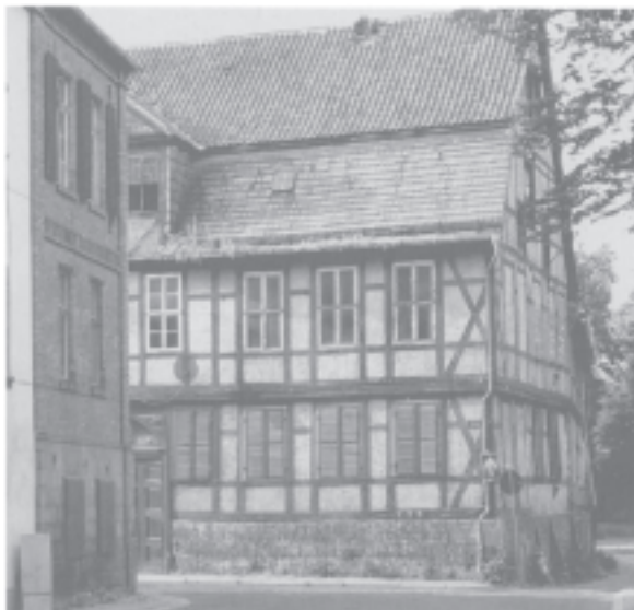
Fig. 4 There remains a considerable amount of work ahead in safeguarding the medieval architecture of Quedlinburg.
