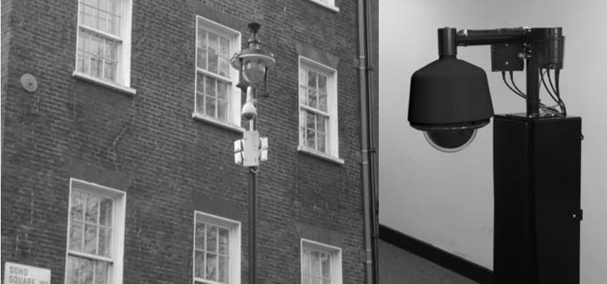
Figure 36.1: Wireless CCTV Deployment.
