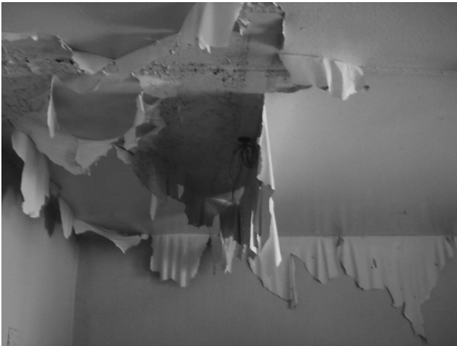
Figure 7.1 H-Block prison cell with evidence of decay on the walls c.2007.
