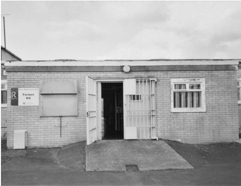
Figure 5.9 Front of H-Block 4, which shows a window facing into the front yard had been blocked since construction, January 2006.
