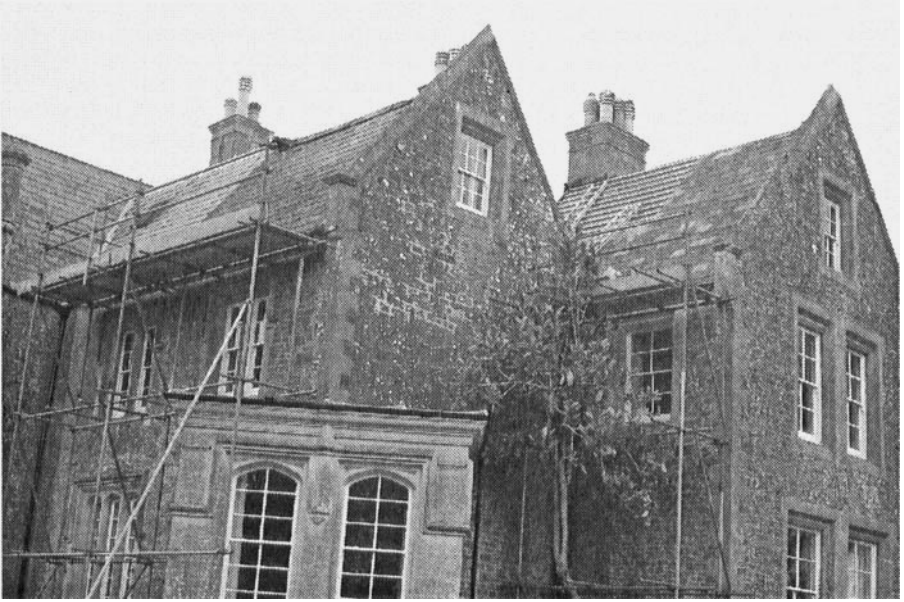
Figure 5.2 The roof of this listed property is being repaired using similar slates to the original, but the guttering is now plastic, painted to resemble the original cast iron.
