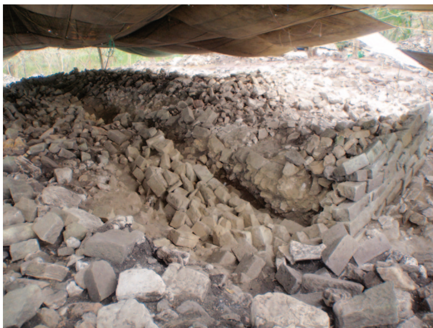
Fig. 10.2 Structure 10, Rastrojón, in its collapsed state
