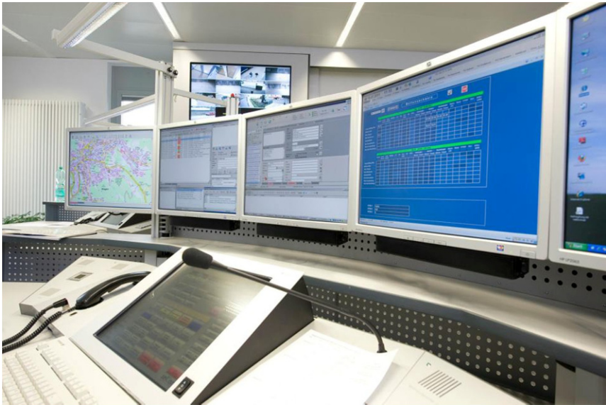
Figure 36: Work infrastructure in the control center
