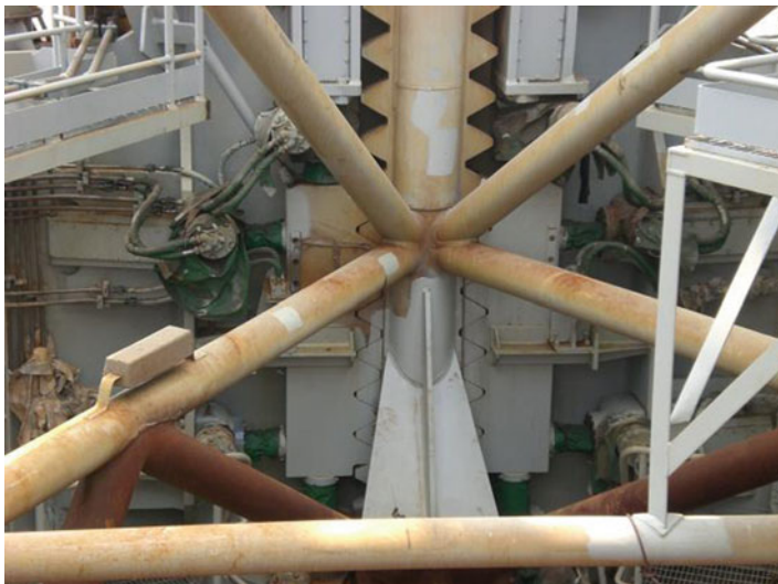
Fig. 10.9 Rack chocks are inserted against the leg's racks to transfer the vertical load away from the pinions (Source: Remedial Offshore)
