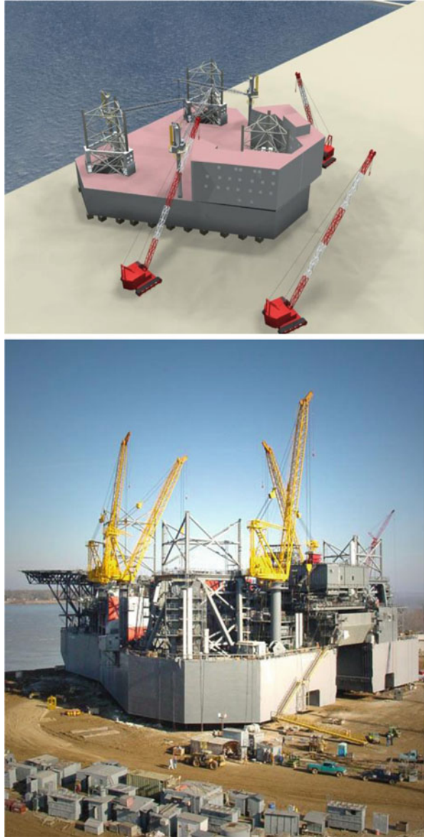
Fig. 11.5 Topside installation on F&G JU 2000E ( top ) and Bob Palmer ( bottom ) at the LeTourneau Vicksburg, Mississippi yard (Source: Freide and Goldman)
