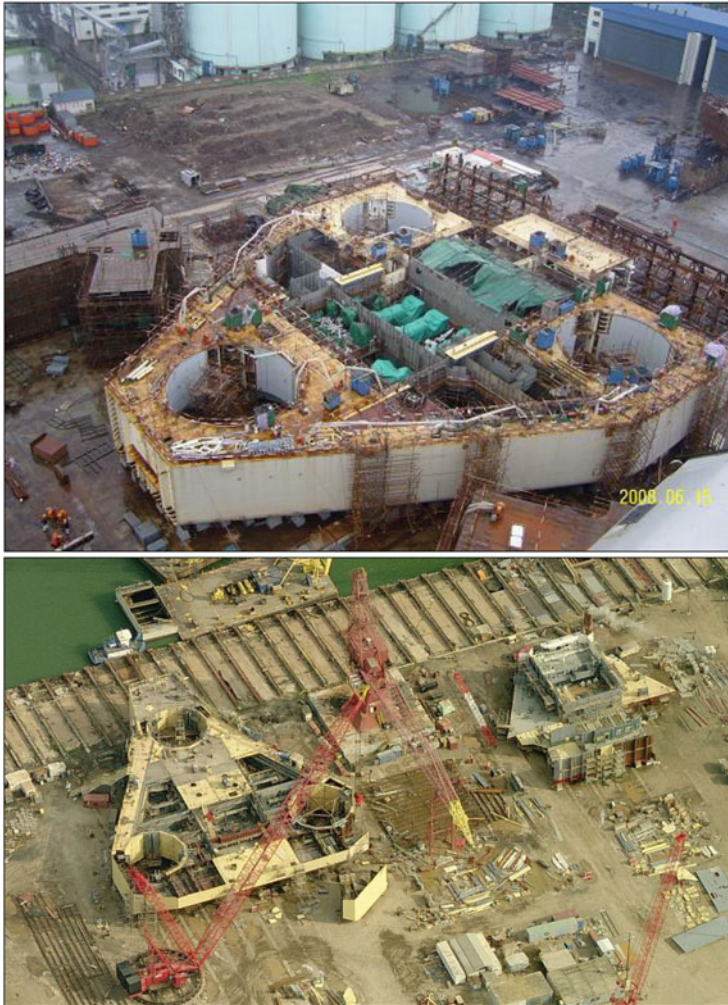
Fig. 11.4 Hull construction of a F&G Super M2 rig ( top ) and two LeTourneau Super 116s at the AmFELS Brownsville, Texas yard. In the top image, much of the hull has been completed and machinery has been installed on the lower decks. In the bottom image, two hulls are under construction. (Source: Remedial Offshore; Microsoft)
