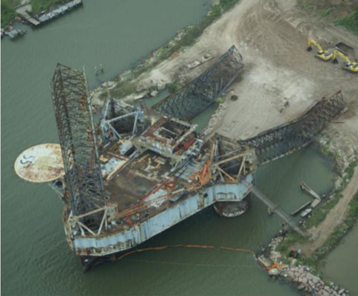
Fig. 1.24 The dead-stacked jackup rig Zeus being dismantled in Freeport, Texas (Source: Texas General Land Office)
