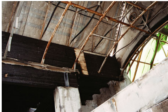
Fig. 3.4 Charring of the glued-laminated beams and bending of the steel beams
