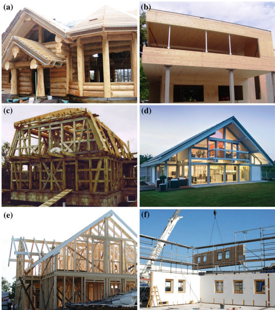
Fig. 3.15 Overview of the basic structural systems in timber construction; (a) log construction, (b) solid timber construction, (c) timber-frame construction, (d) frame construction, (e) platform-frame construction, (f) panel construction; photograph by F. Kager
