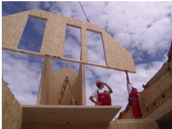
Fig. 3.19 Platform-type erection in the massive panel timber construction, photograph by F. Kager
