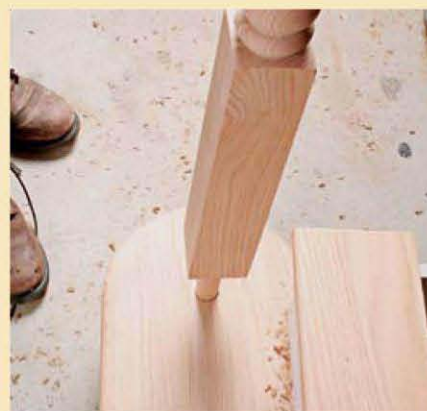
A thick dowel secures this newel. Usually 1\frac{1}{4} in. in diameter, the dowel is glued into a hole drilled plumb into the tread.
