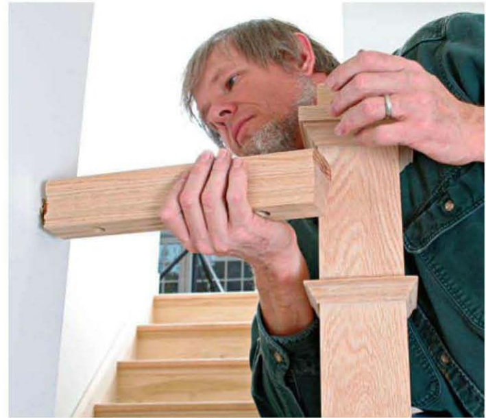
A combination of finesse and force. Slip the rail over the dowel in the wall and pull back on the newel to horse the rail into place.
