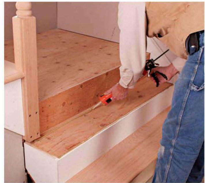
Finish treads and risers transform a rough stair. The plywood subtreads and subrisers got the house through construction; now it's time to dress the stair with finish-grade material.
