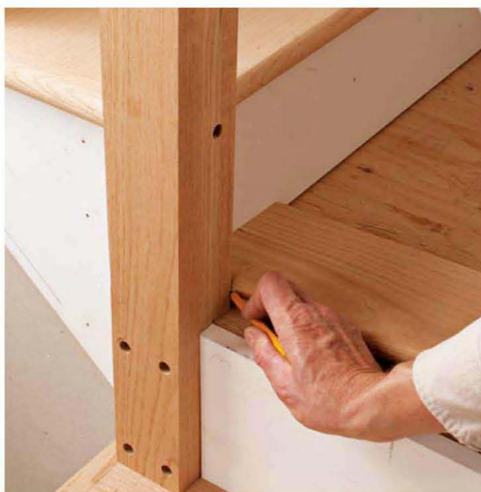
Mark the landing tread to fit the newel. Hold the landing tread just behind its installed location to mark the notch that will fit it around the newel.
