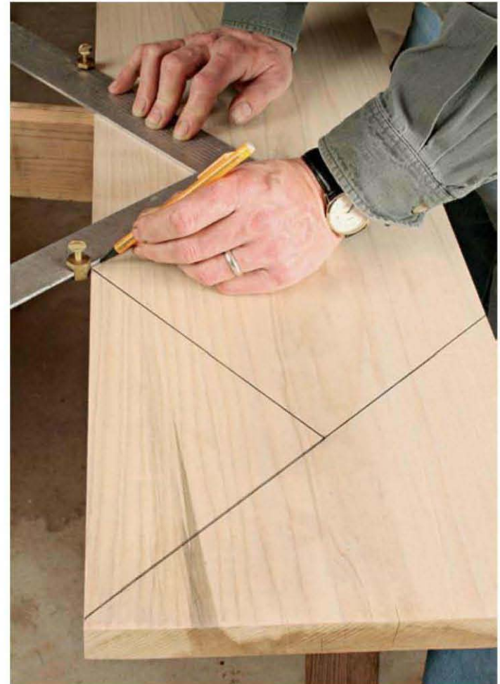
Finished notched stringers lay out like any notched stringer. A framing square with stair gauges set at the rise and run lays out the stringer. The fact that the riser cuts will be miters doesn't affect the layout.
