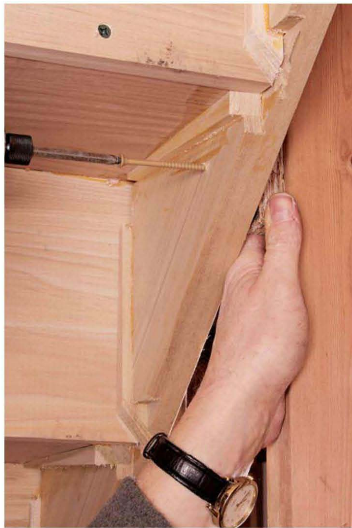
Fasten stringers to the framing from below. At installation, shim between the stringer and the studs, and drive long screws from the back of the stairs.
