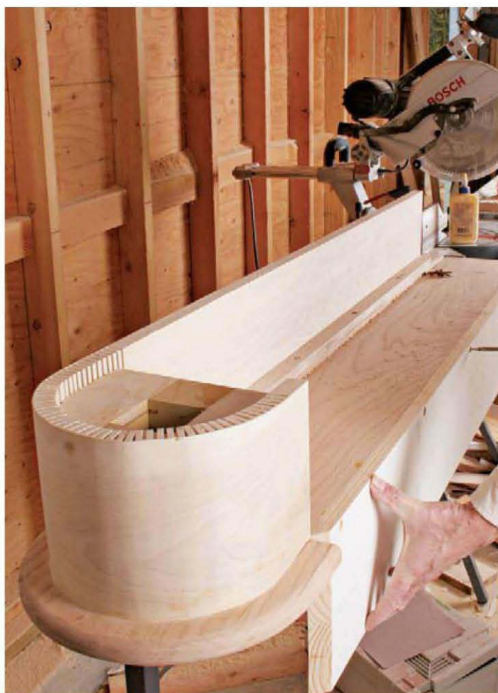
Stairbuilding requires both shop and site work. This bullnose starting step was made in a shop but joined to the stair on site.
