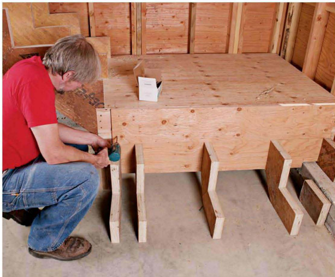
Stairs turn at landings, which are built during the framing stages. Stout construction is called for, as a landing supports both flights of stairs.
