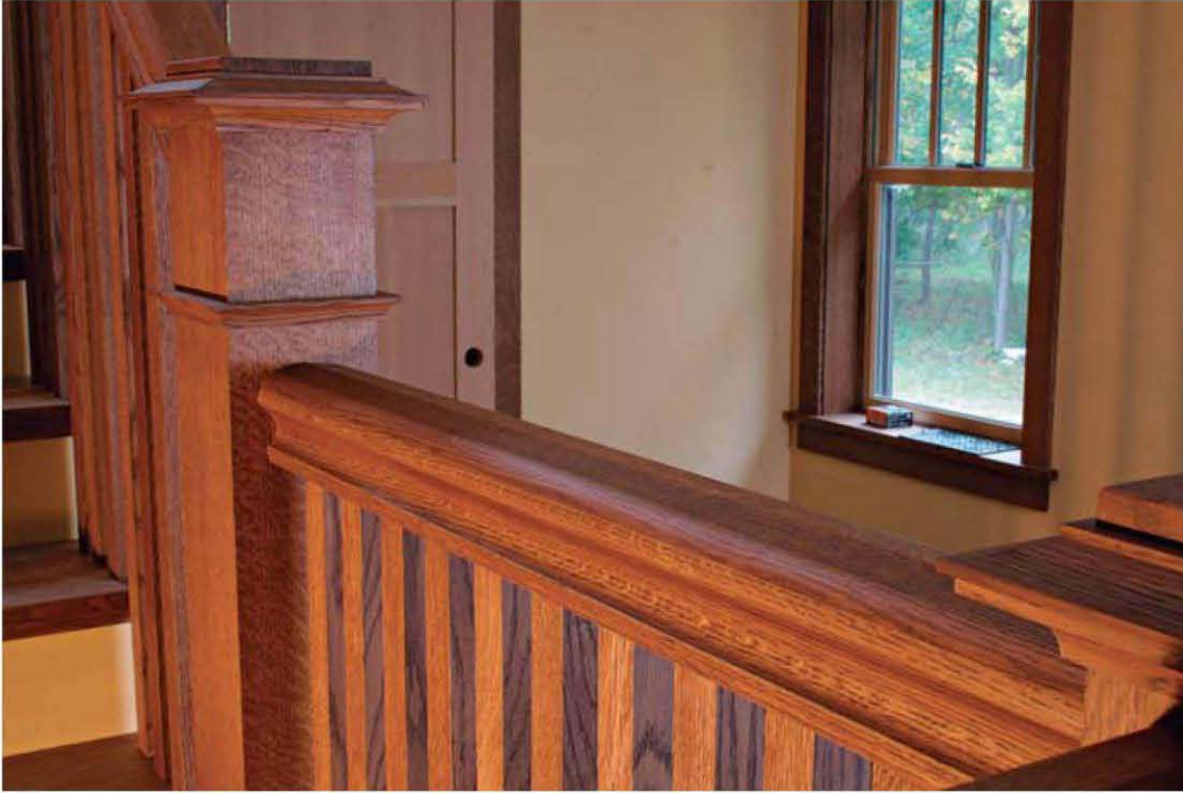
A fully custom balustrade wouldn't be complete with a manufactured rail. This one was made by profiling a glued lamination.
