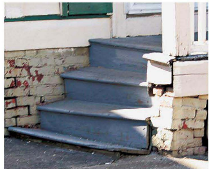
These stairs may once have been safe, but the crazy quilt of varying riser heights and out-of-level treads is an accident waiting to happen.
