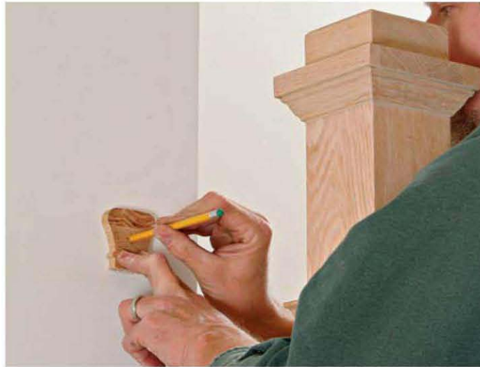
Lay out where the rail hits the wall. A center-drilled section of rail is used to mark for a dowel hole to be drilled in the wall. The rail section is also used to lay out centers for drilling the newel and the rail.
