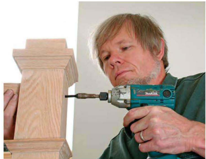
Impact driver sets the screw. Driven into the pilot hole through a \frac{1}{2} -in.-dia. countersink hole, a LedgerLok secures the balcony rail.
