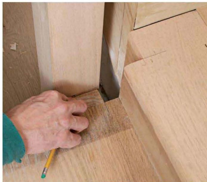
Mark the height of the tread in place. The most accurate way to measure is often not to measure but to mark in place.
