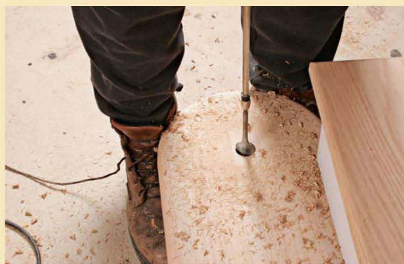
A spade bit follows the pilot hole. A quick-release extension provides the length needed for the long dowel.
