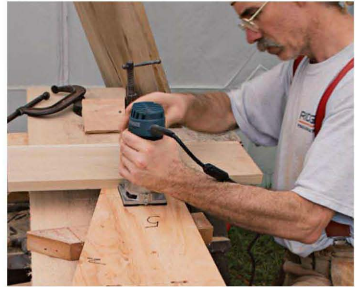
Slots allow movement. Use a 1/4-in. straight bit to slot the subtreads for screws. These slots allow treads to move relative to the plywood so they don't split.
