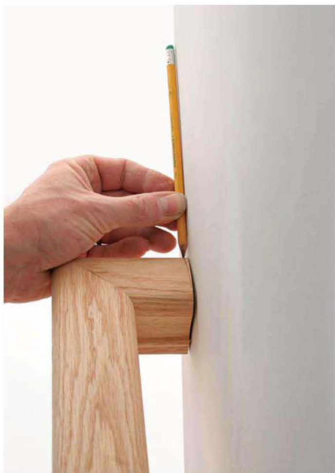
Houses aren't ever perfectly plumb, level, square, or straight. Stairbuilding skills include fitting finish work to such imperfect conditions.
