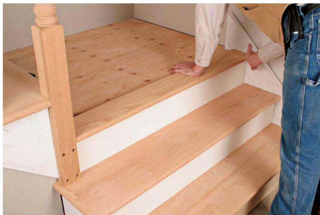
Fasten the landing tread for the long term. Use plenty of subfloor adhesive under the landing tread, and nail it down with hand-driven 8d finish nails. Drill pilot holes for the nails near the ends.
