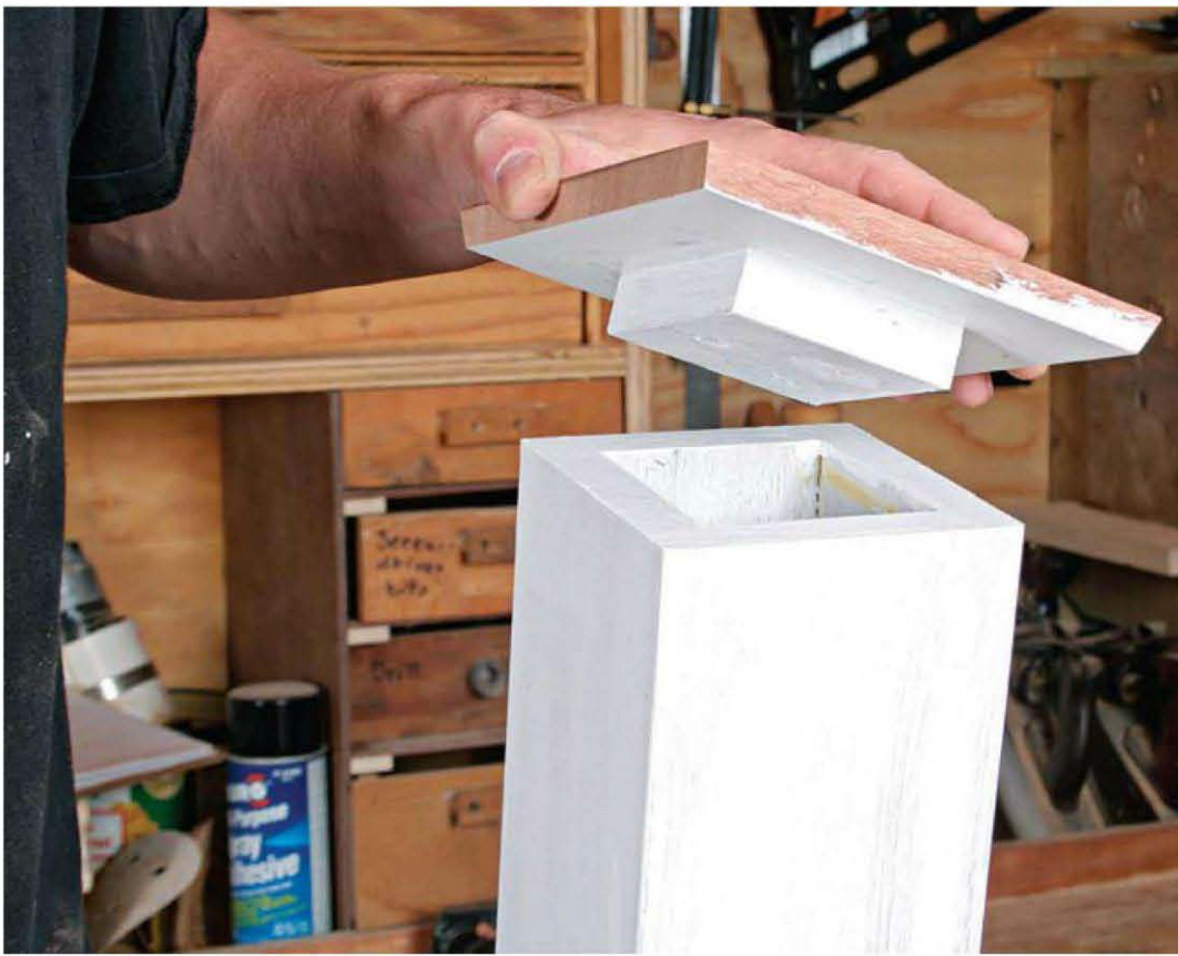
Avoiding exposed fasteners in the cap. A block screwed to the bottom of the primed cap slips into the newel.
