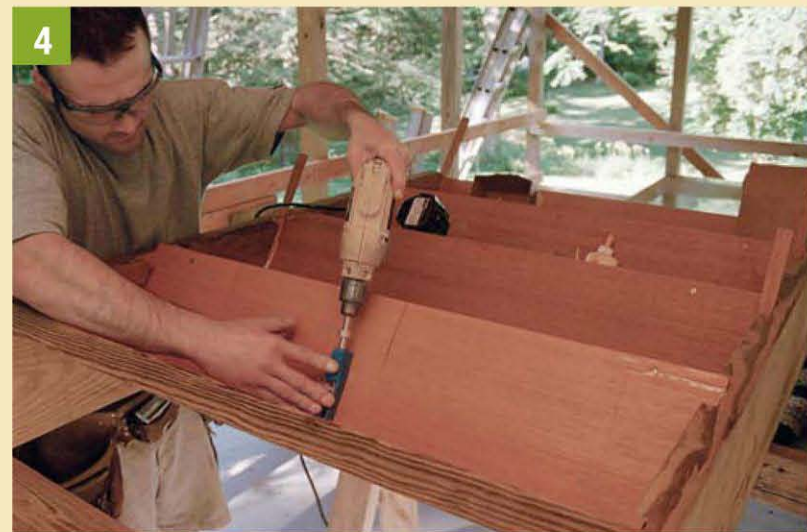
4 A pocket-screw jig and a proprietary bit make angled screw holes to join the top of the risers to the treads.
