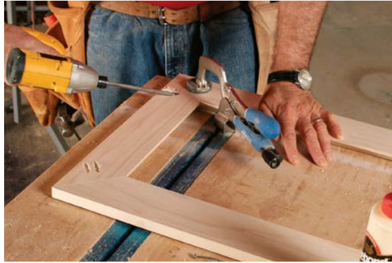
A PAIR OF POCKET SCREWS (Kreg® micro jig) at each miter creates a tight joint. The holes are then plugged and sanded flush.
