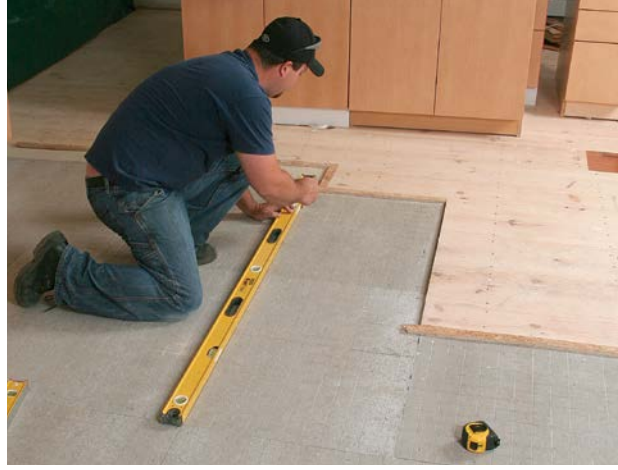
WORK FROM THE END. With the position of the sink's overhead light as a starting point, use the kitchen designer's measured drawings to determine the end of the island. Measure from the wall cabinets to create a parallel line that the island will follow.
