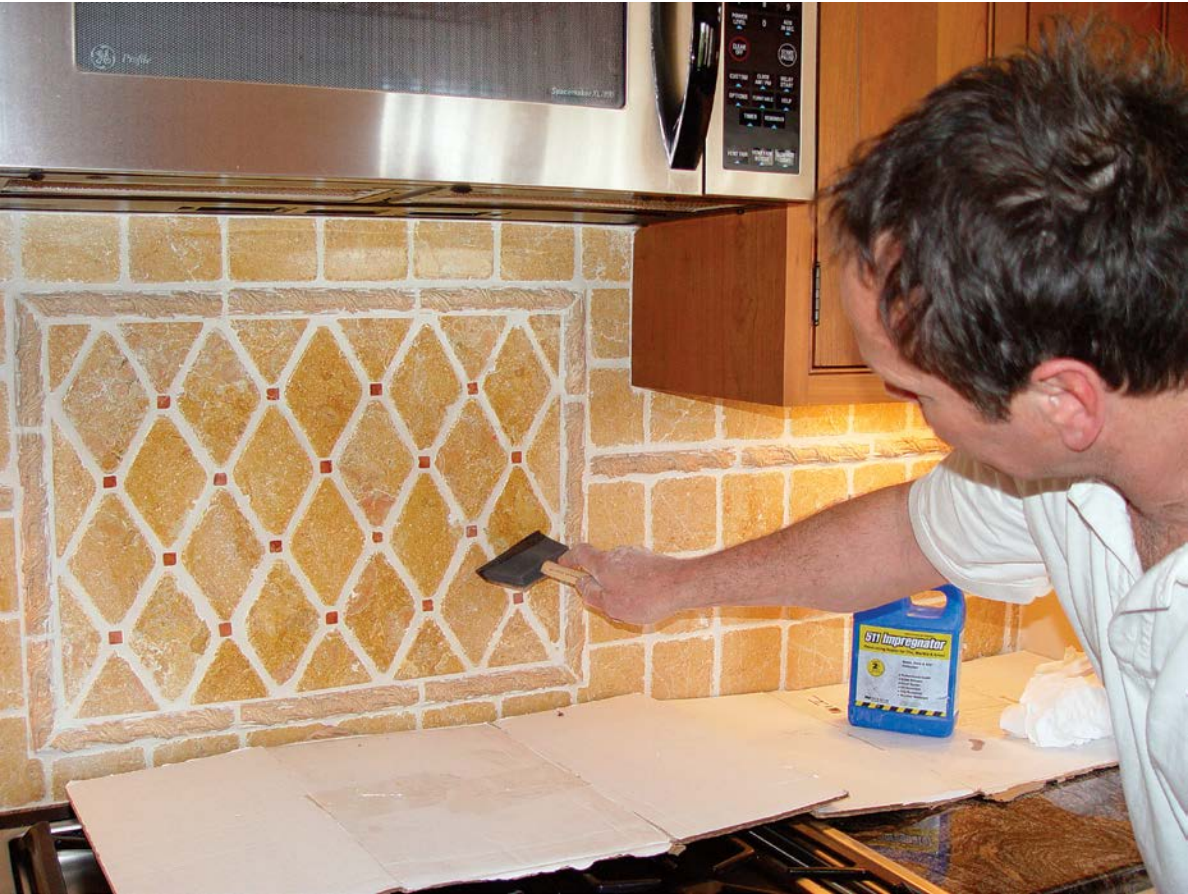
WHEN THE GROUT HAS CURED FOR 48 HOURS, a final coat of sealer provides additional protection for the tile and the grout.
