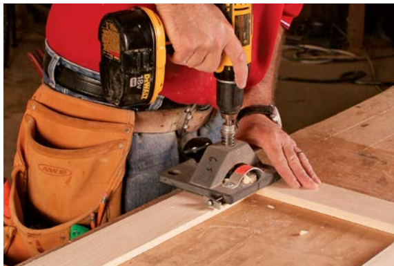
A HINGE-BORING JIG ( www.eurolimited.com ) makes quick work of preparing each door to receive the new concealed hinges.
