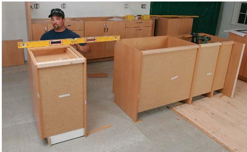
CHECK ACROSS THE GAP. Where there's a gap in the island's cabinet run for a dishwasher or other appliance, use a long level to ensure that both cabinets are at the same height. Check front and back to confirm that the cabinet tops are in the same plane. Also make sure the cabinets are spread at the proper distance and their sides are parallel.
