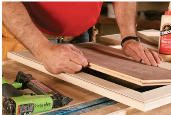
CUT THE OLD DOORS DOWN to the appropriate size to become panels, and cut a matching rabbet around each so that it will sit about \frac{1}{4} in. below the front face of the frame.
