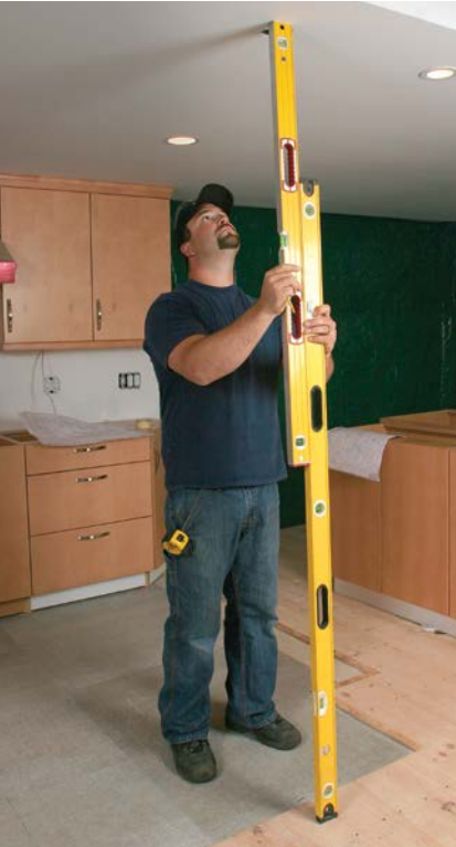
CENTER THE SINK. Using a pair of levels, transfer to the floor the location of the light fixture centered over the sink. This becomes the starting point for the layout.
