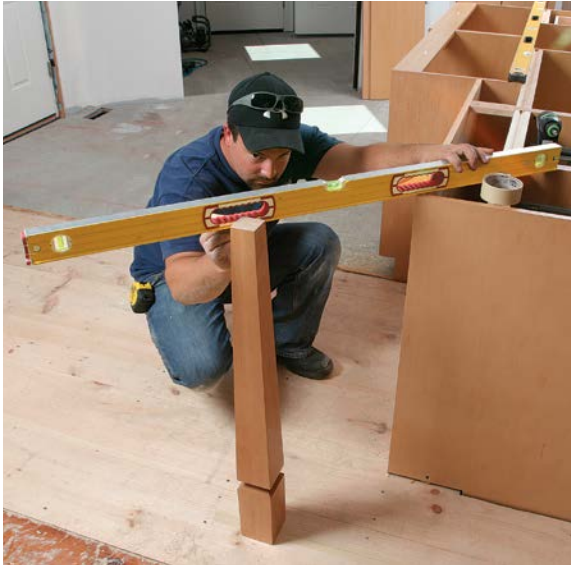
LOCATE THE LEGS, AND CUT THEM TO LENGTH. A pair of legs support the eating area's overhanging countertop. Use a pair of levels as straightedges to position the legs in plane with the cabinets.
