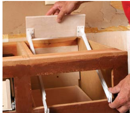
ATTACH THE BRACKETS AND DRAWER SLIDES to a plywood cleat, and install each preassembled unit as one piece.
