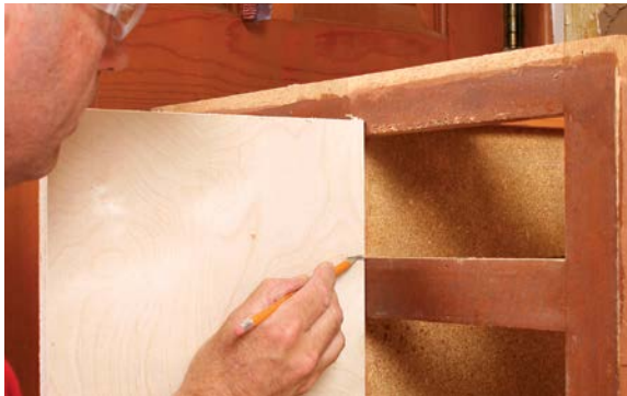
AFTER CUTTING A BACKER BOARD equal to the interior width of each cabinet, use the face frame as a template to mark the drawer-slide mounts before nailing the panel into place at the back of each cabinet.
