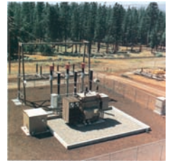
Courtesy of Waukesha Electric Systems.
