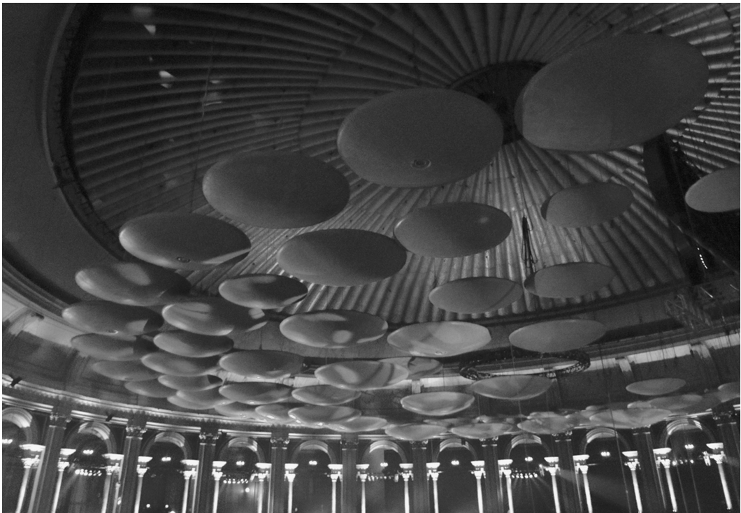
Figure 3.37 Looking up at the volume diffusers used to prevent sound that can cause echoes reaching the dome in the Royal Albert Hall. (Courtesy of Egghead06, commons.wikimedia.org/wiki/File:AcousticDiscsRoyalAlbertHall.JPG .)
